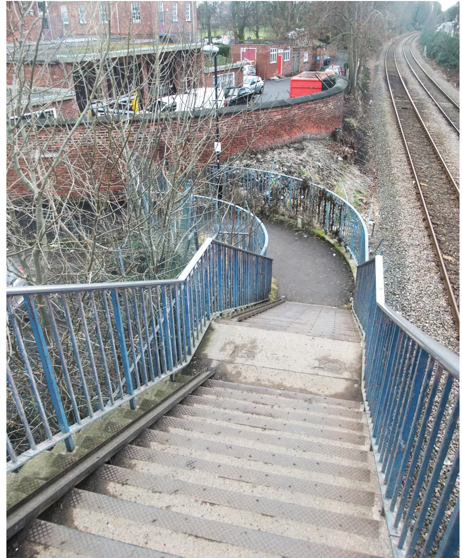
The environment surrounding the pedestrian footbridge into the hospital should be improved
