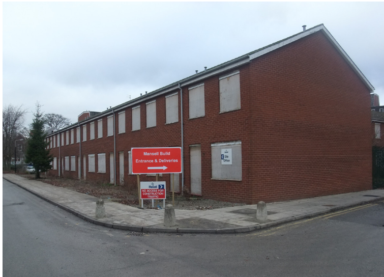
Boarded up patient accommodation is a detractor
