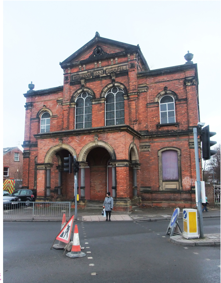
The Wesleyan Chapel is considered 'at risk'
