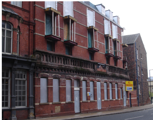
23 Clifford Street is a vacant building opposite the Magistrates' Court. The developer went into receivership.
