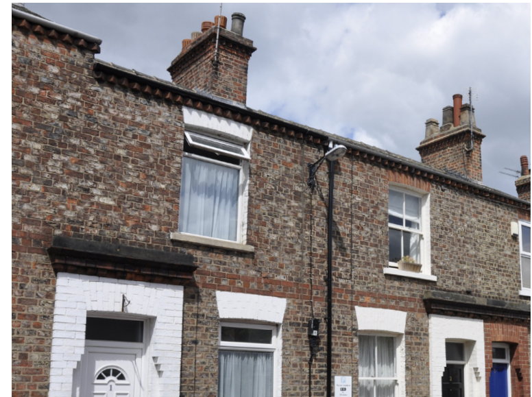
Poorly designed modern windows (left) detract from the appearance of the terrace
