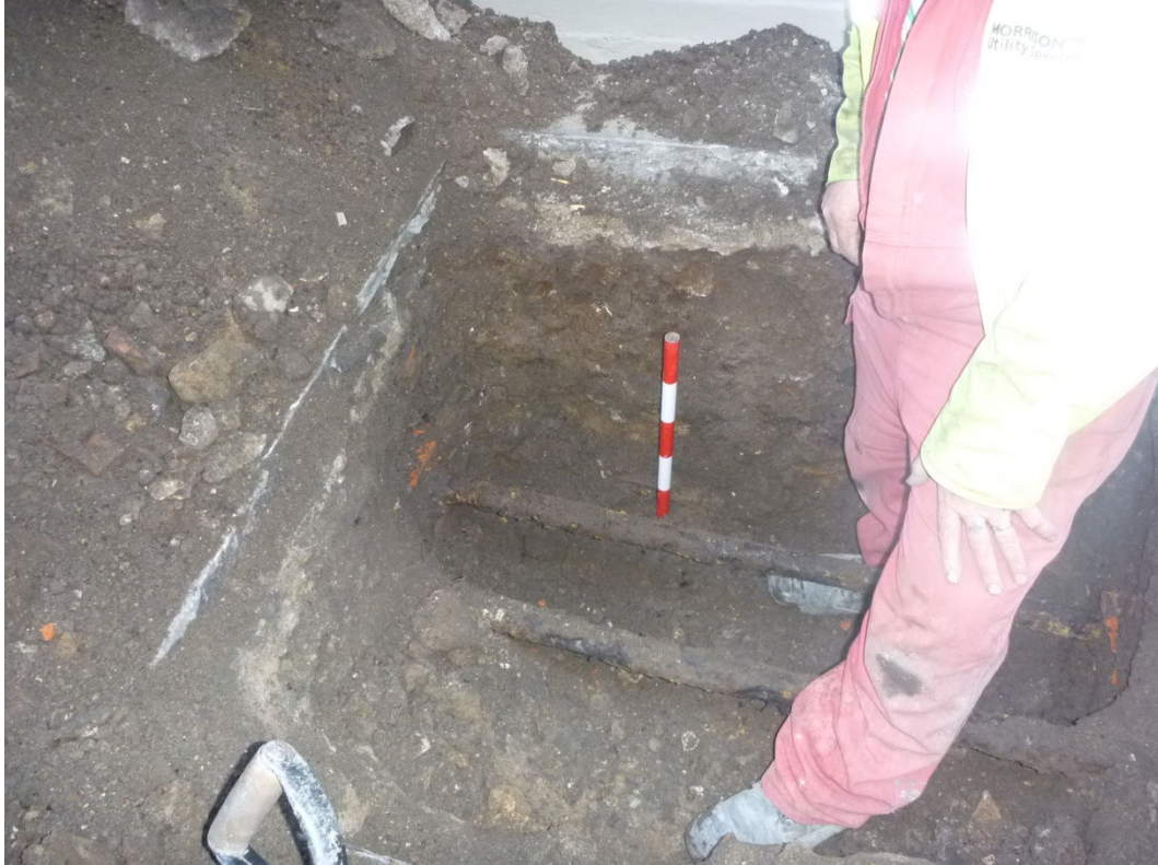
Plate 1: View of trench showing exposed armoured cables at maximum extent of excavation.
