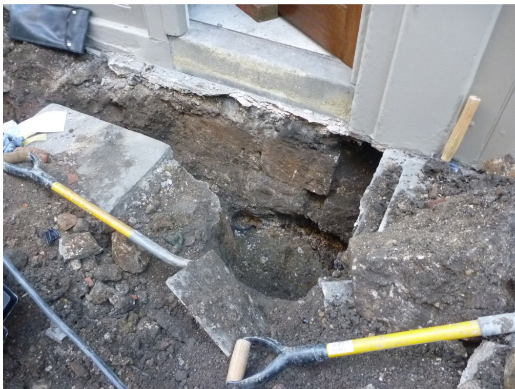
Plate 2: Exposed stone foundation of 31 The Shambles (cable access point beneath visible stone work).
