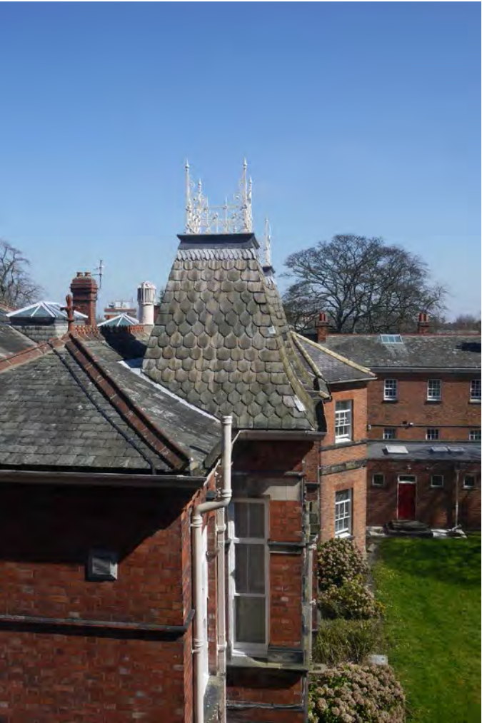
View of the eastern elevation of the link block from the principal building, 2015
