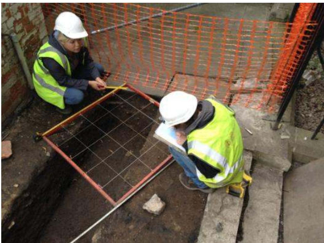
Plate 6. Recording of 19th century service cuts in a slot through Church Lane
