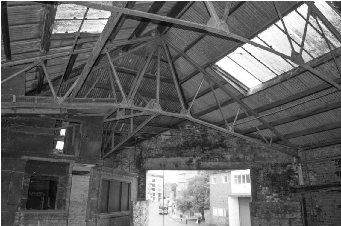
Photograph 84. Detail of the truss used to form the hipped roof and gablet of internal bay 17
