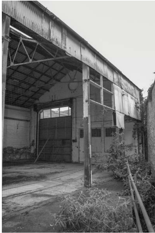
Photograph 27. The rear of the building with missing timber frame and exposed steel frame
