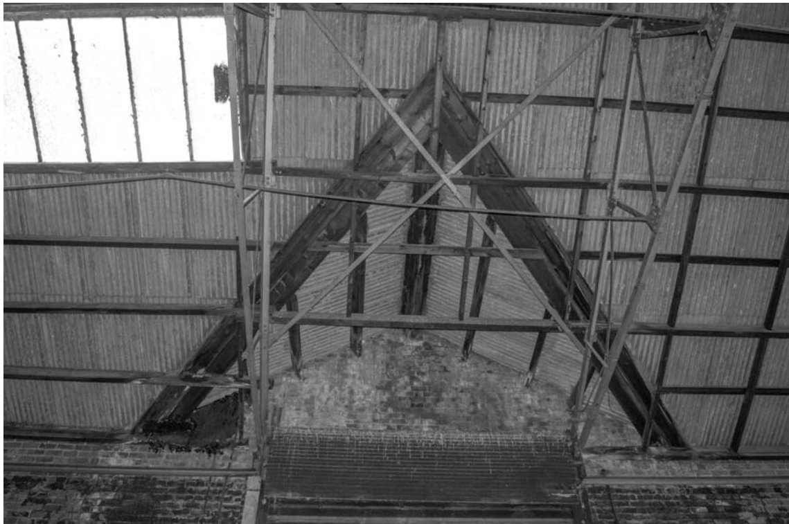
Photograph 60. The roof construction of the gablet showing timber beams attached to the steel truss
