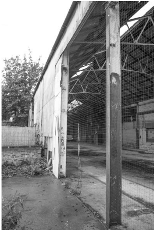
Photograph 28. The rear of the building with missing timber frame and exposed steel frame
