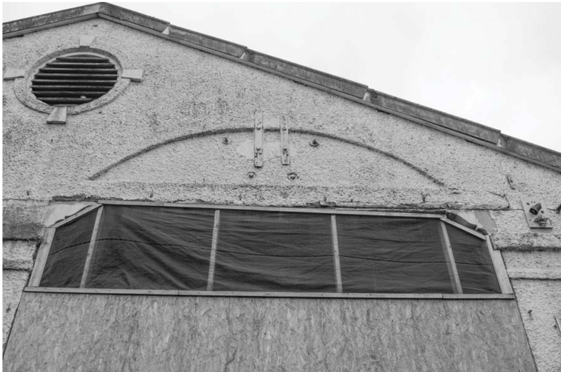
Photograph 24. Detail of recess in render denoting the location of a relieving arch
