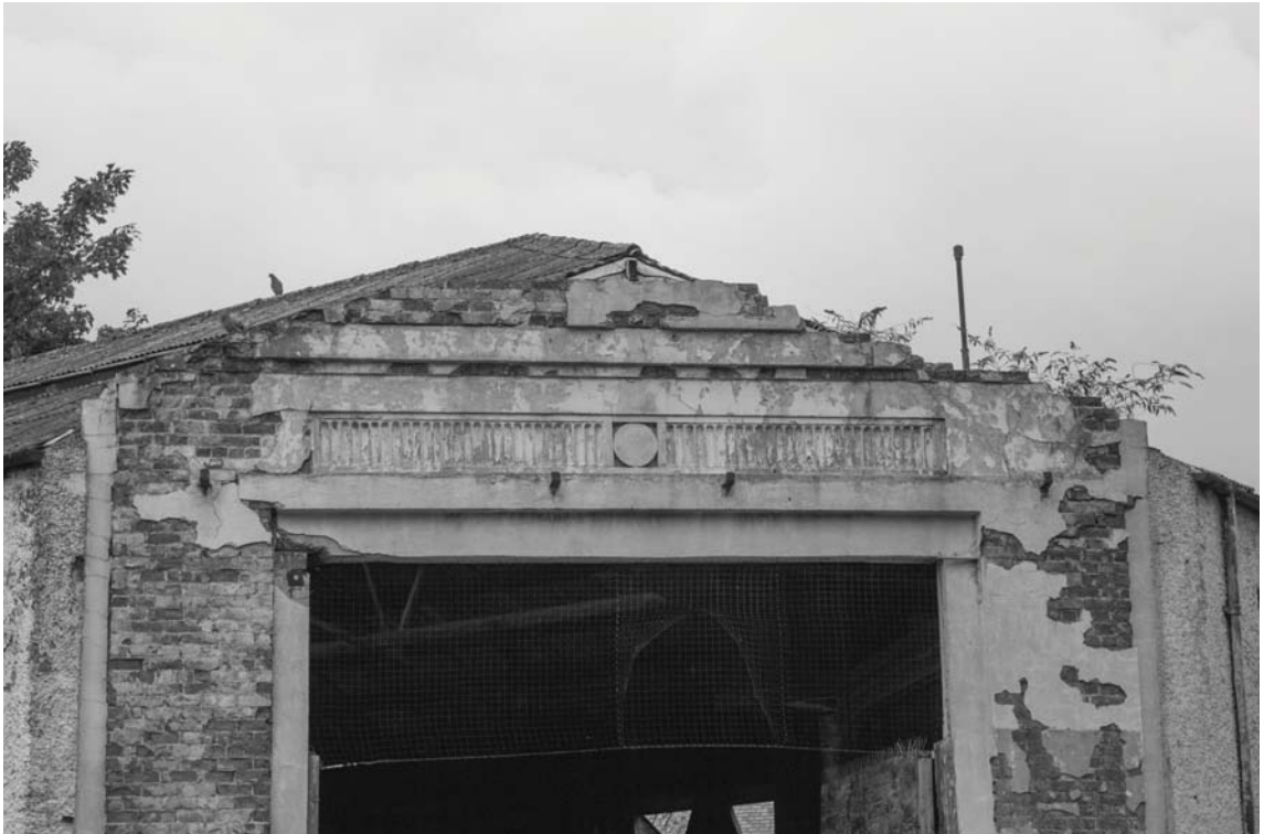
Photograph 15. Detail of the southern gable frieze and stepping towards apex with damage
