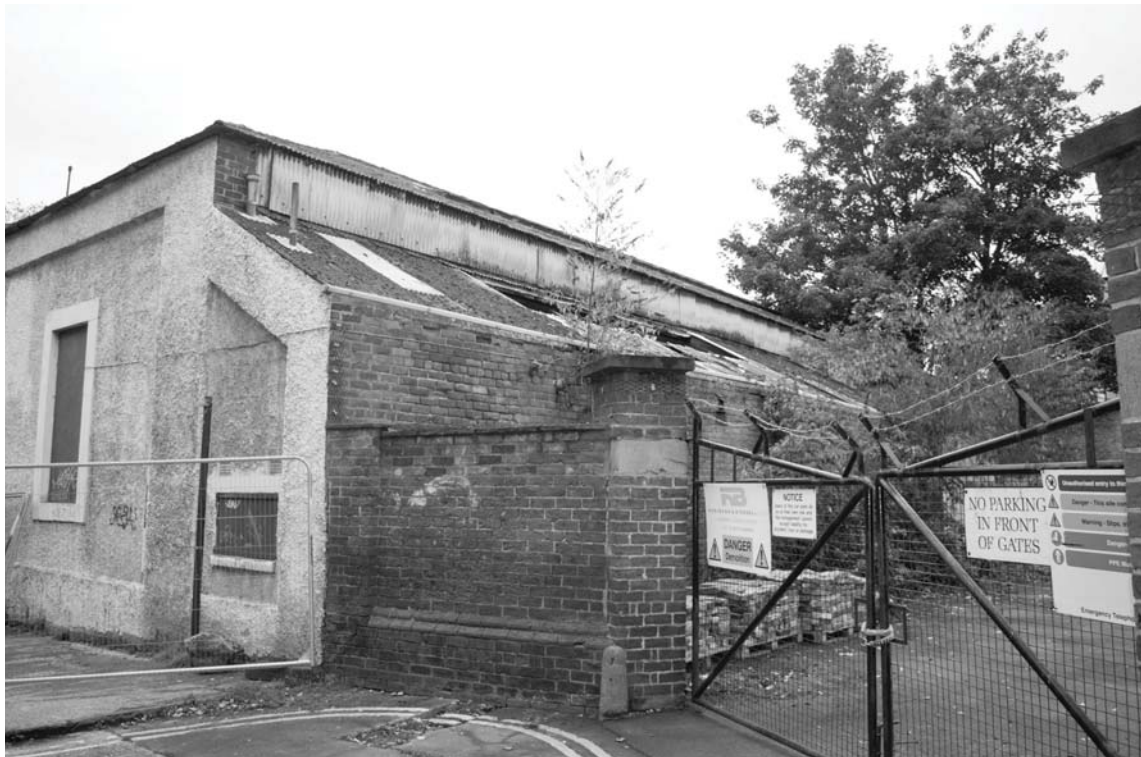
Photograph 32. The rear of the lean-to showing corrugated asbestos roof
