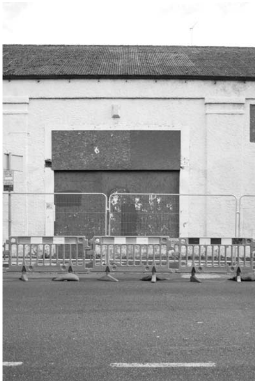
Photograph 8. The boarded-up door and window in external bay 5 with perspective control
