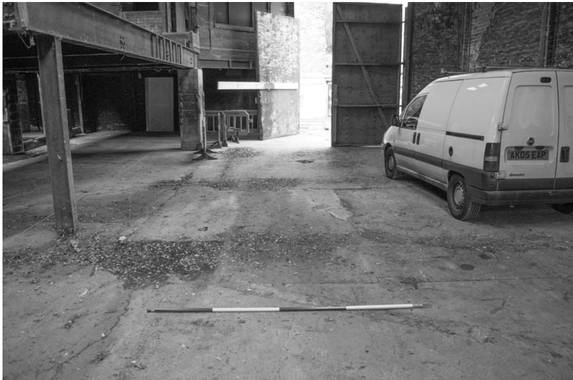
Photograph 66. Ambiguous scarring in the concrete floor
