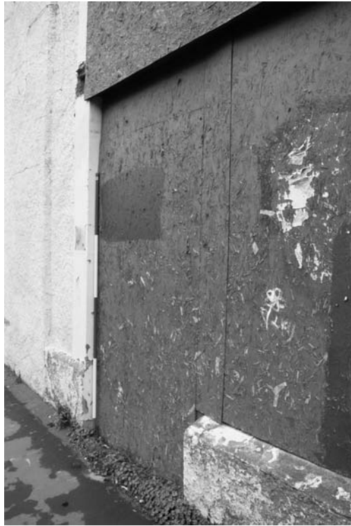
Photograph 13. Detail of where the sill band or plinth has been cut away
