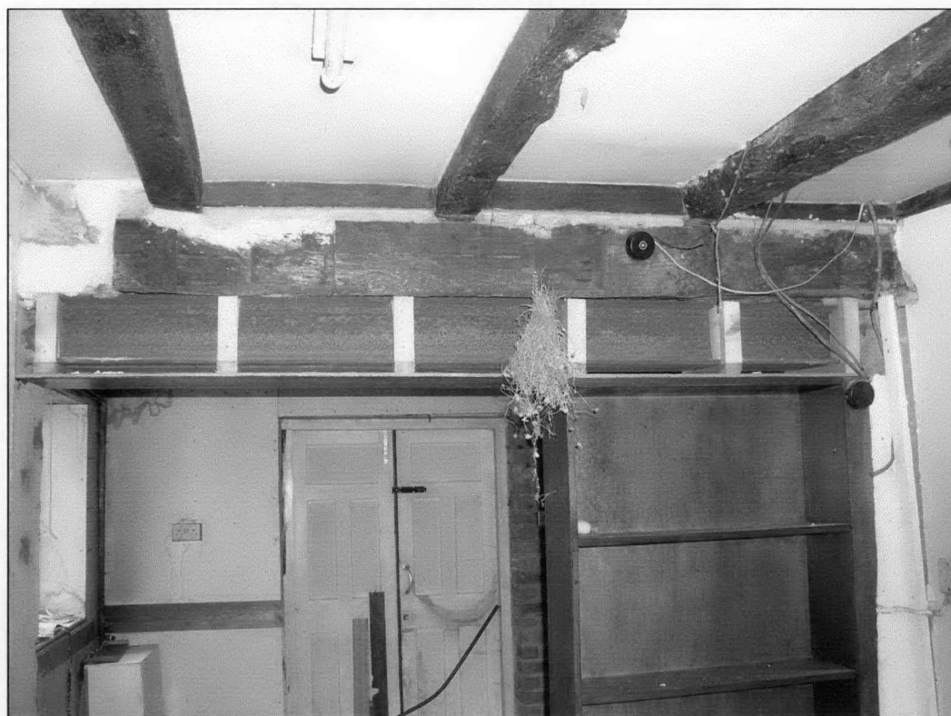
Plate 10 The Old Manor, Clifton: timber lintel inserted over doorway during construction of workshop extension, note floor joist sit above timber.
