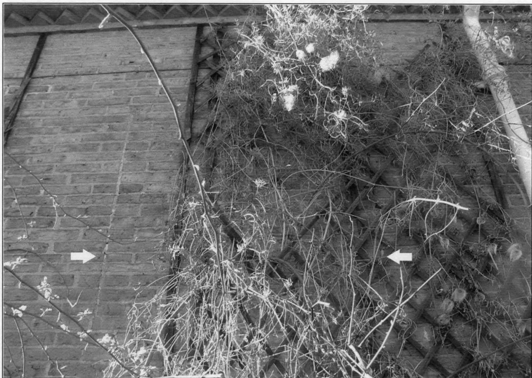
Plate 2 The Old Manor, Clifton: joint scars on north-east elevation
