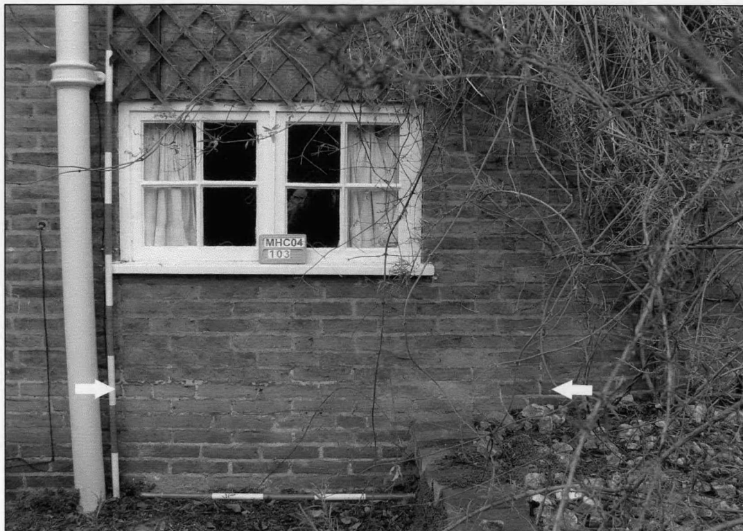
Plate 3 The Old Manor, Clifton: joint scars on south-east elevation
