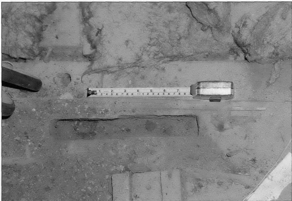
Plate 14 The Old Manor, Clifton: mortise for queen post or 'A' frame strut on rear tie beam, west attic space.
