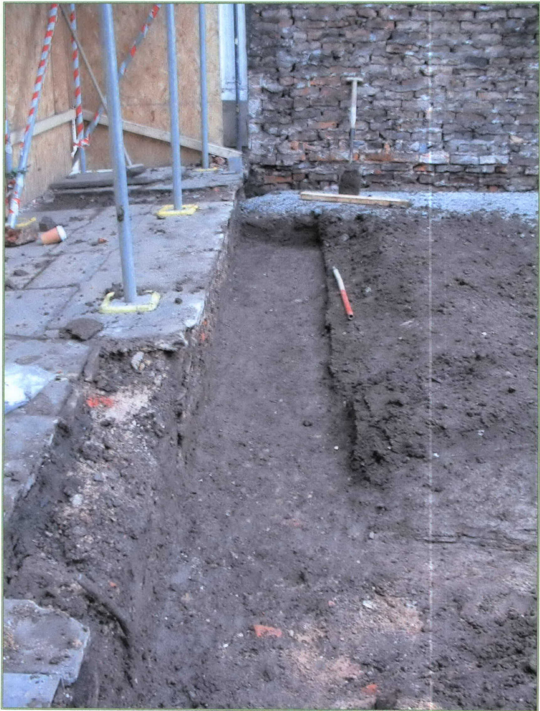
Plate 3. Showing excavated strip footing along the length of ditch [102] and its fill. (Scale of 1m).
