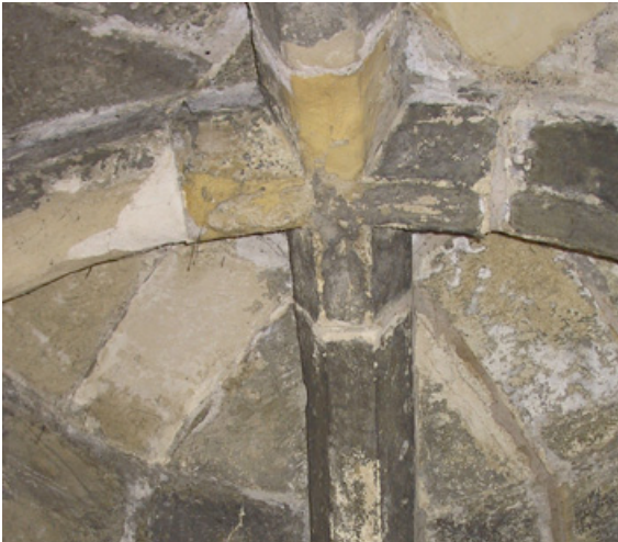
The internal stonework is subject to decay
