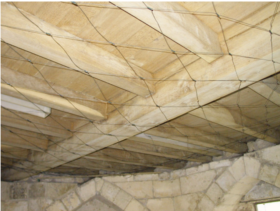
The main beam supporting the first floor flags is cracked along its length
