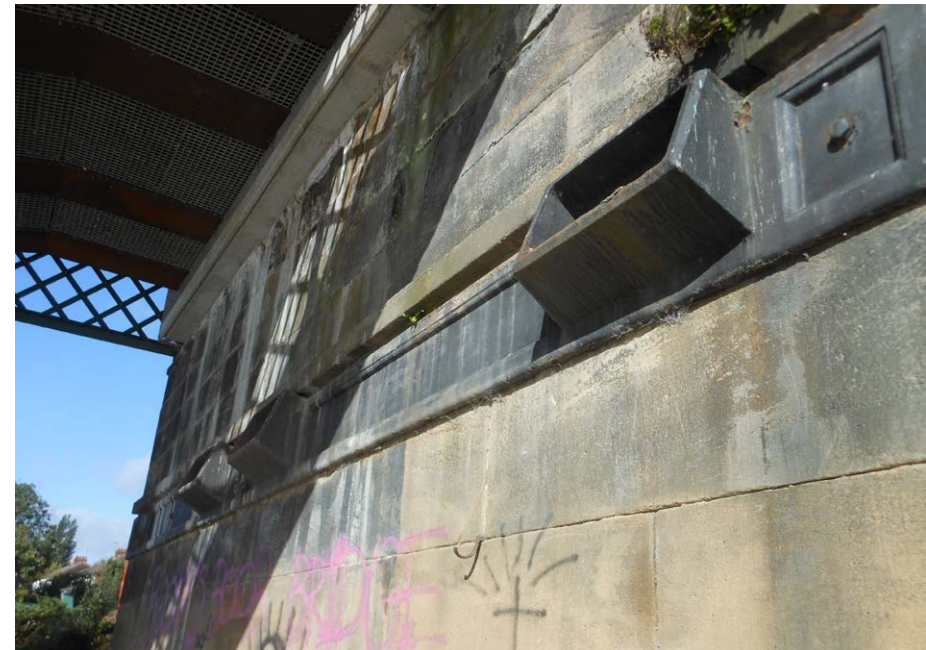
Fig. 6: One of the cast-iron beams built into the bridge to support the bracing added in 1847.
