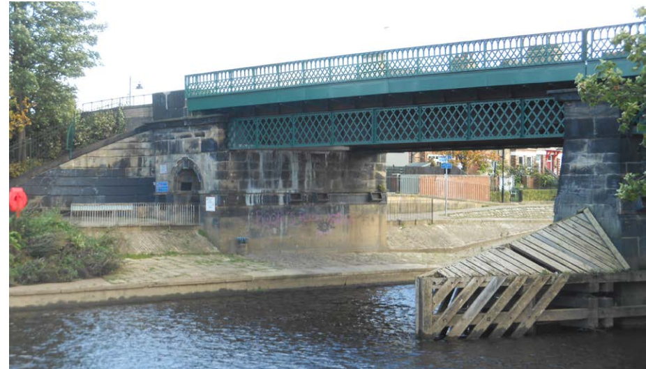
Fig. 14: The west side of the bridge after the 2015 alterations. Note the loss of stone work over the pier and northern abutment.
