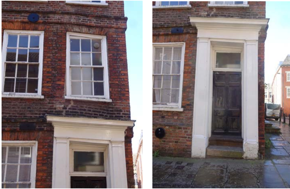
Distorted doorway and sash window to no. 12 Castlegate
