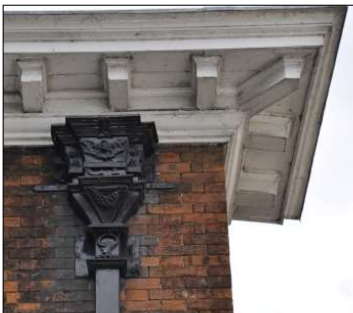
Figure 5: Original drain hopper and fall pipe detail with Bathurst crest and decorative detail with initials of the owners CFB i.e. Charles and Frances Bathurst
