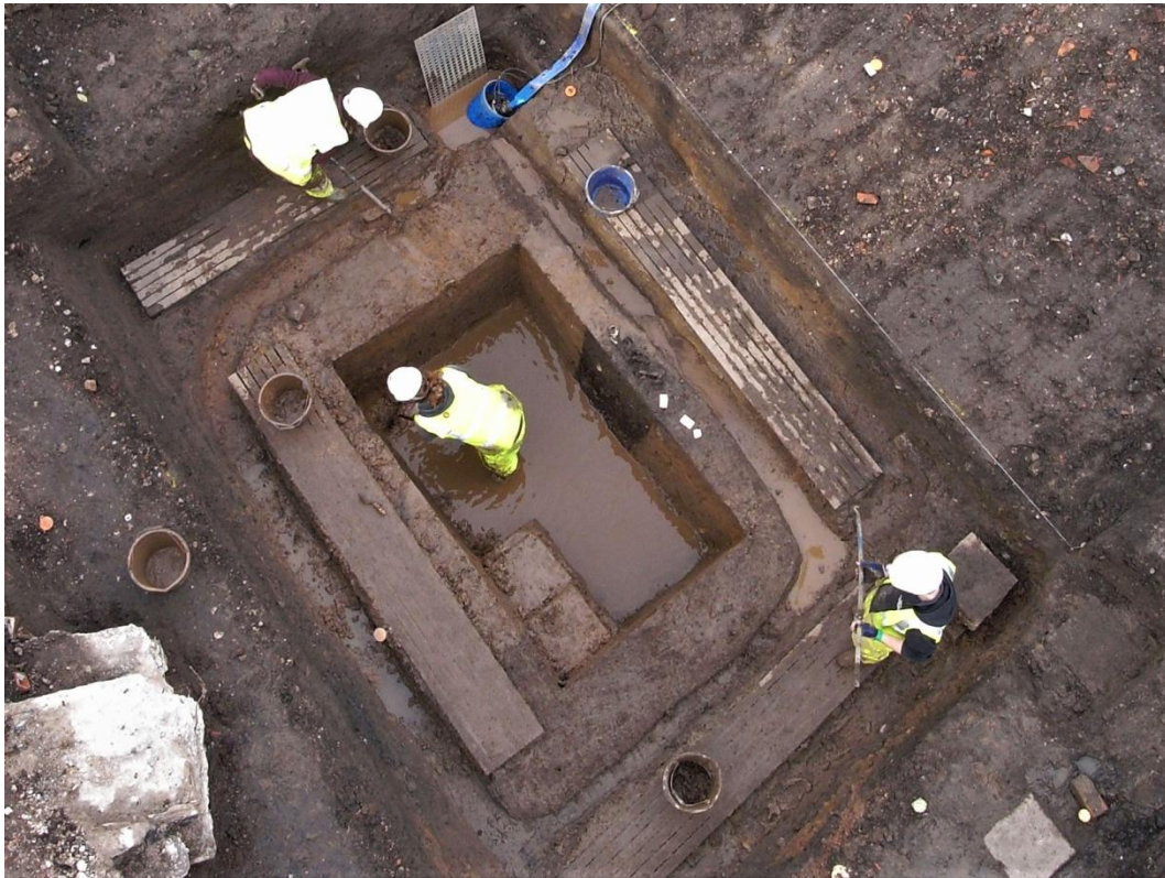
Plate 17 Aerial view of excavation in progress showing rising groundwater. Image courtesy of David Dodwell
