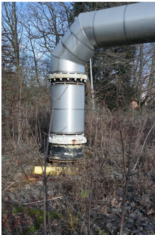
Plate 15 The northern end of the major pipeline in Zone B facing east
