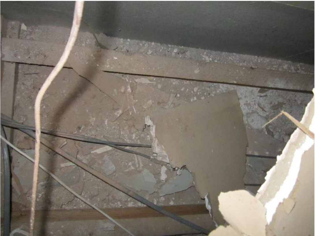
Fig 19 View from above of inserted plasterboard ground floor ceiling in former Phase I stair hall
