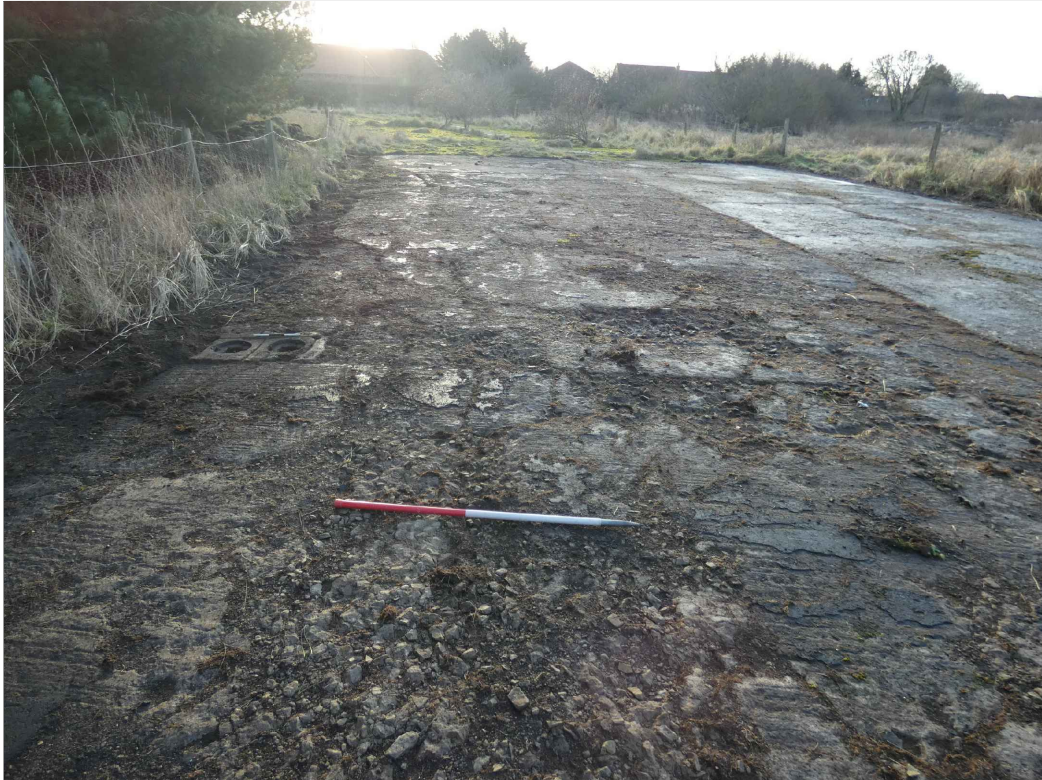
PLATE 3: West taxi-way after vegetation clearance, showing excavated double light, looking S (photo 3/489).
