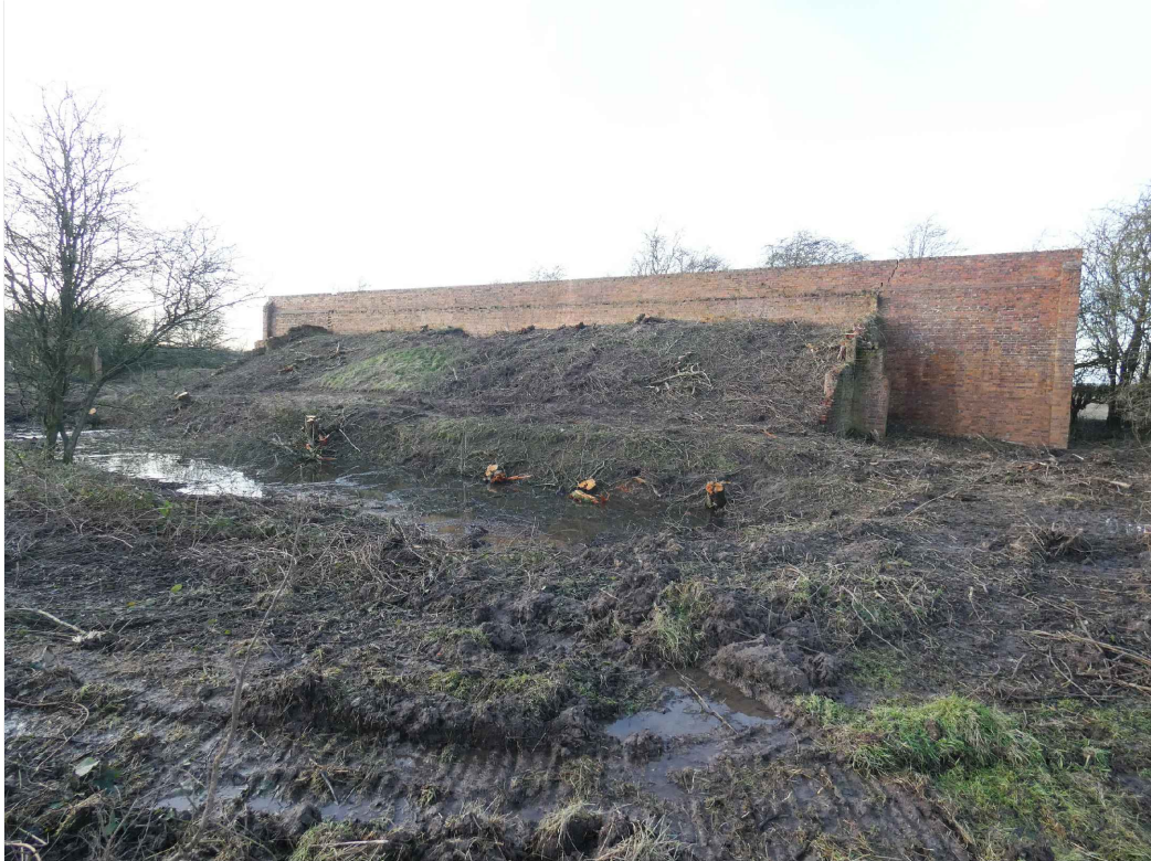
PLATE 37: Machine gun range, showing relationship of butts and catch pit, looking NW (photo 3/583).
