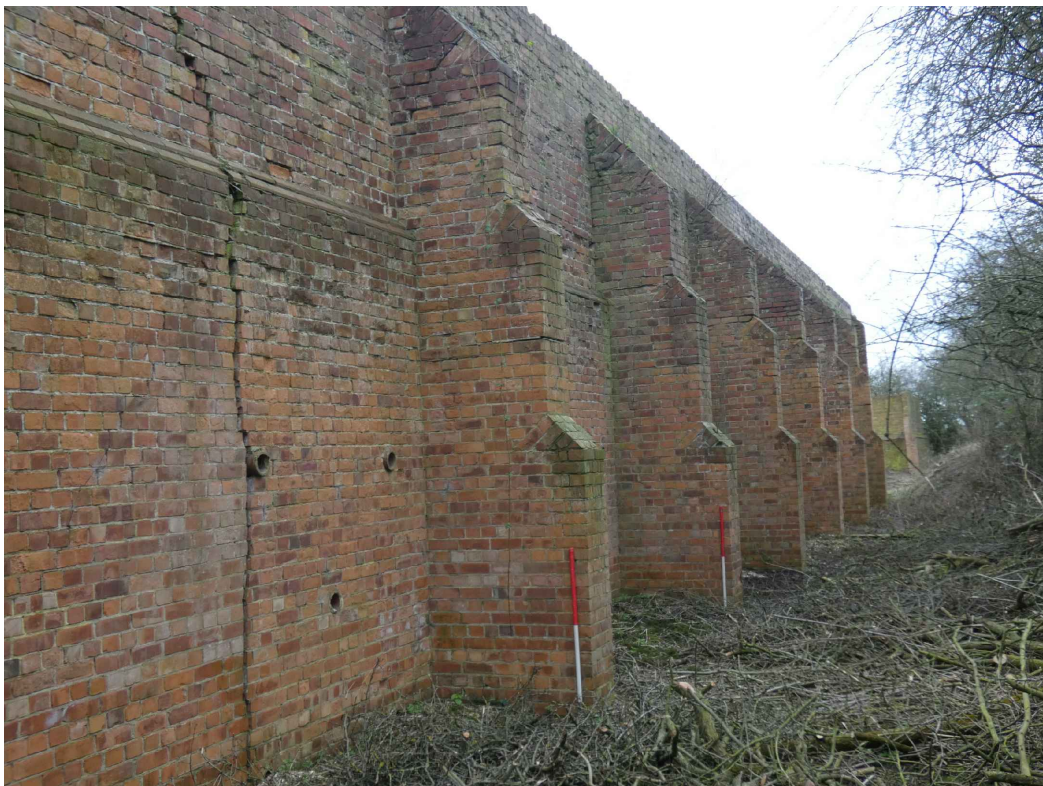
PLATE 34: Machine gun range, north wall of butts showing buttresses and drainage holes, looking SW (photo 4/739).
