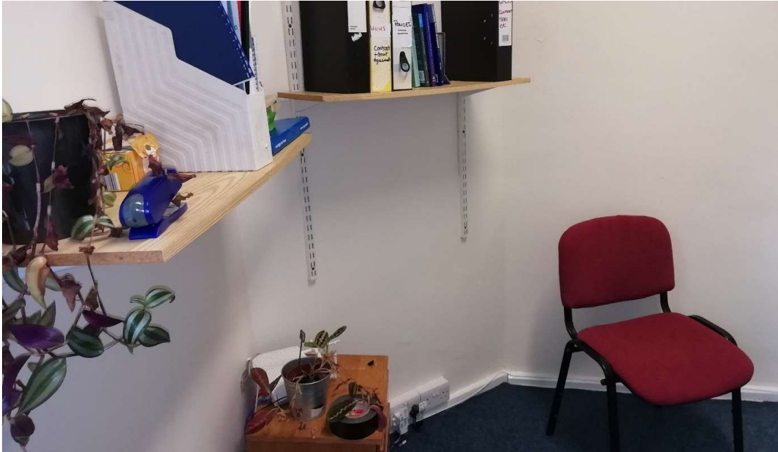
Fig 20 Blocked corner fireplace in first floor, rear, right hand room to be re-opened and fitted with reclaimed, Georgian fireplace shown at Fig IN
