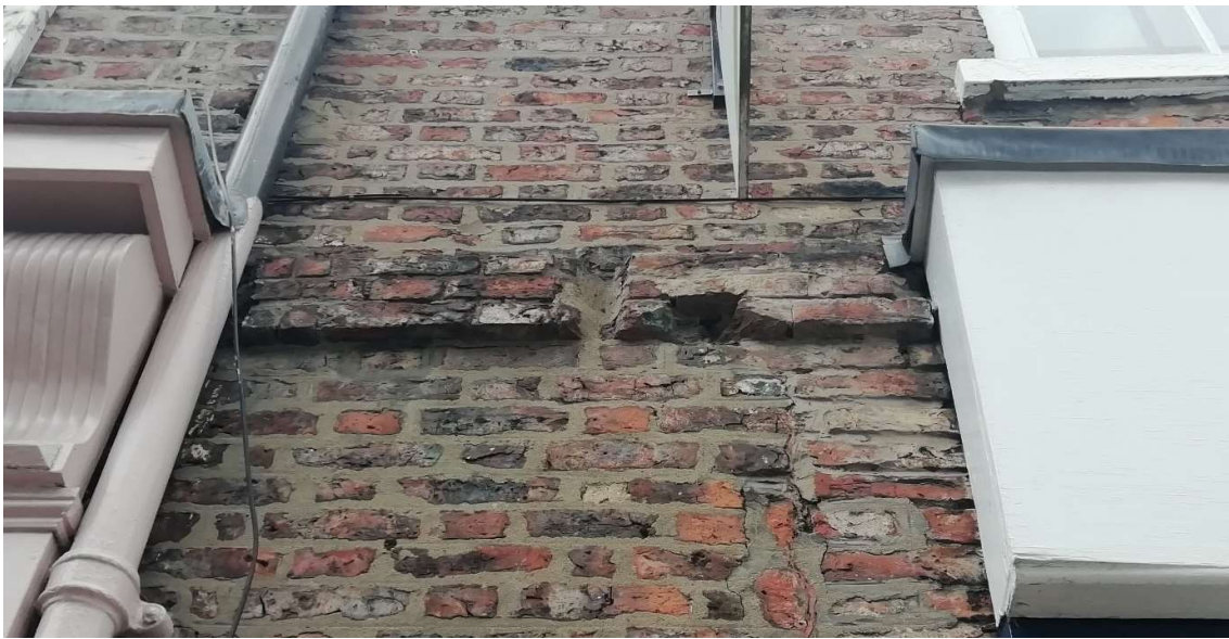
Fig 31 Brick string course above former line of first floor windows to be reinstated
