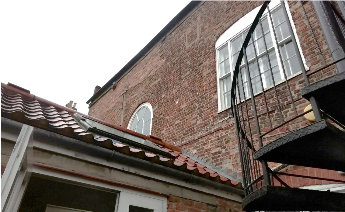
Fig 32 Rear elevation, stair window obscured by modern extension, replacement windows, fire escape and scarring to brick evidencing previous works
