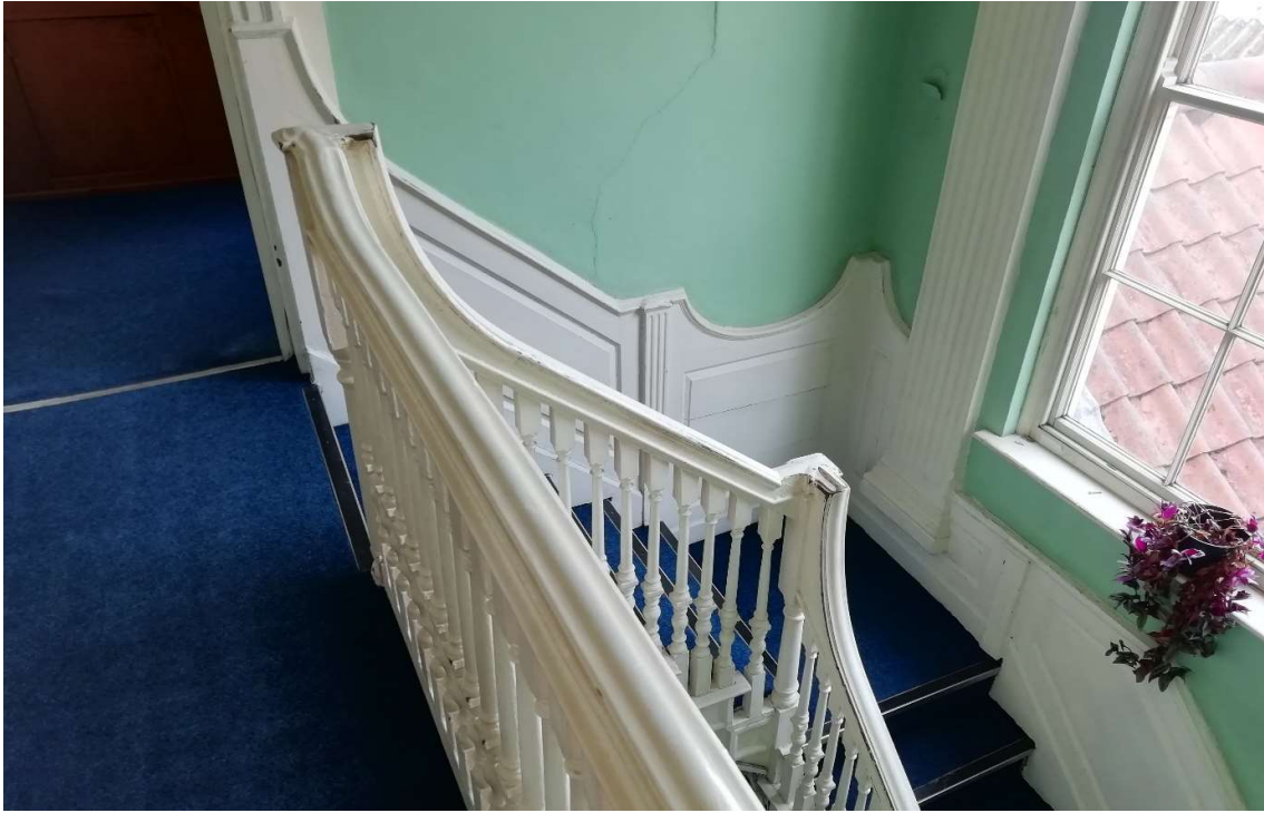
Fig 22A Stair (cracks in stair bay wall to be tied and modern doorway below infilled)
