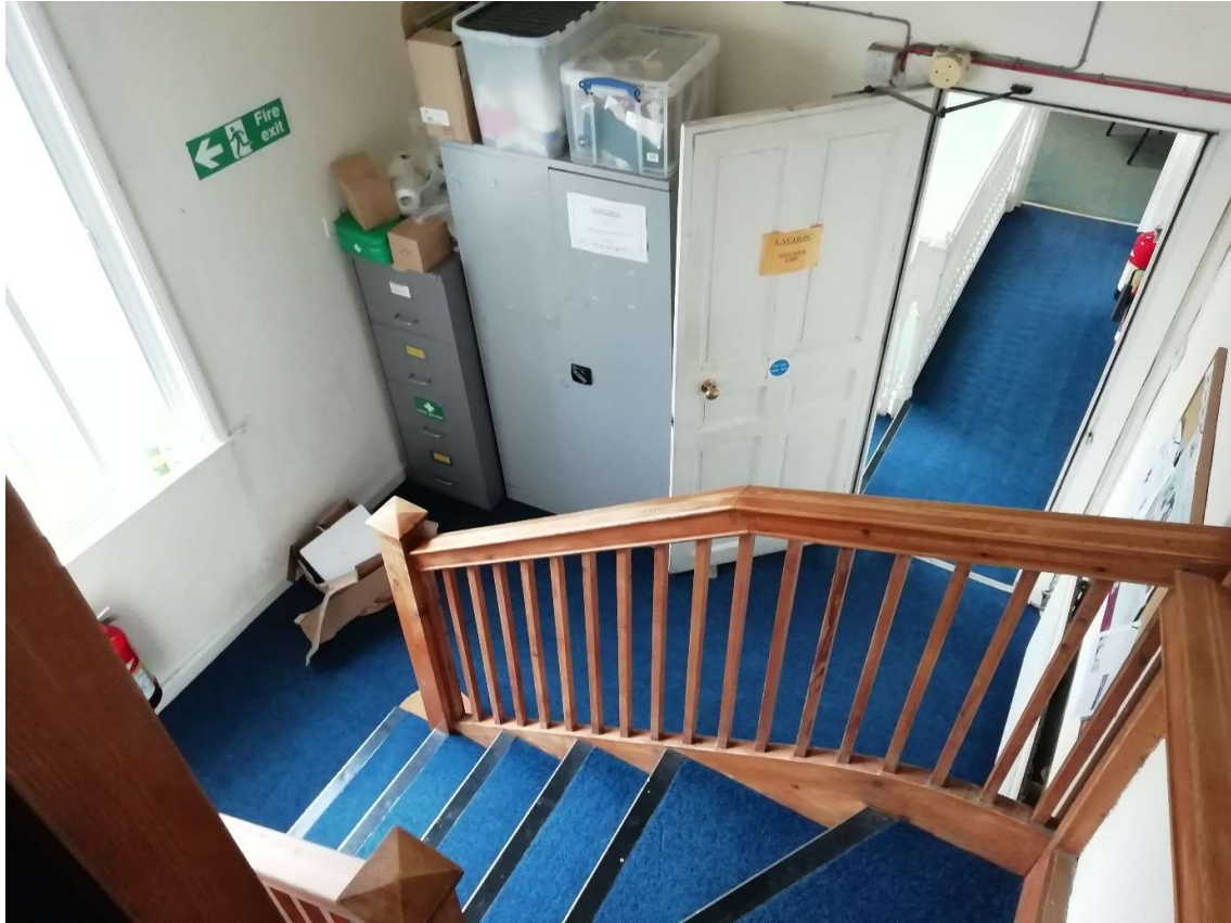
Fig 14 Second floor, left , rear room with new stair to attic and replacement window. Stair encases chimney breast and back stair.
