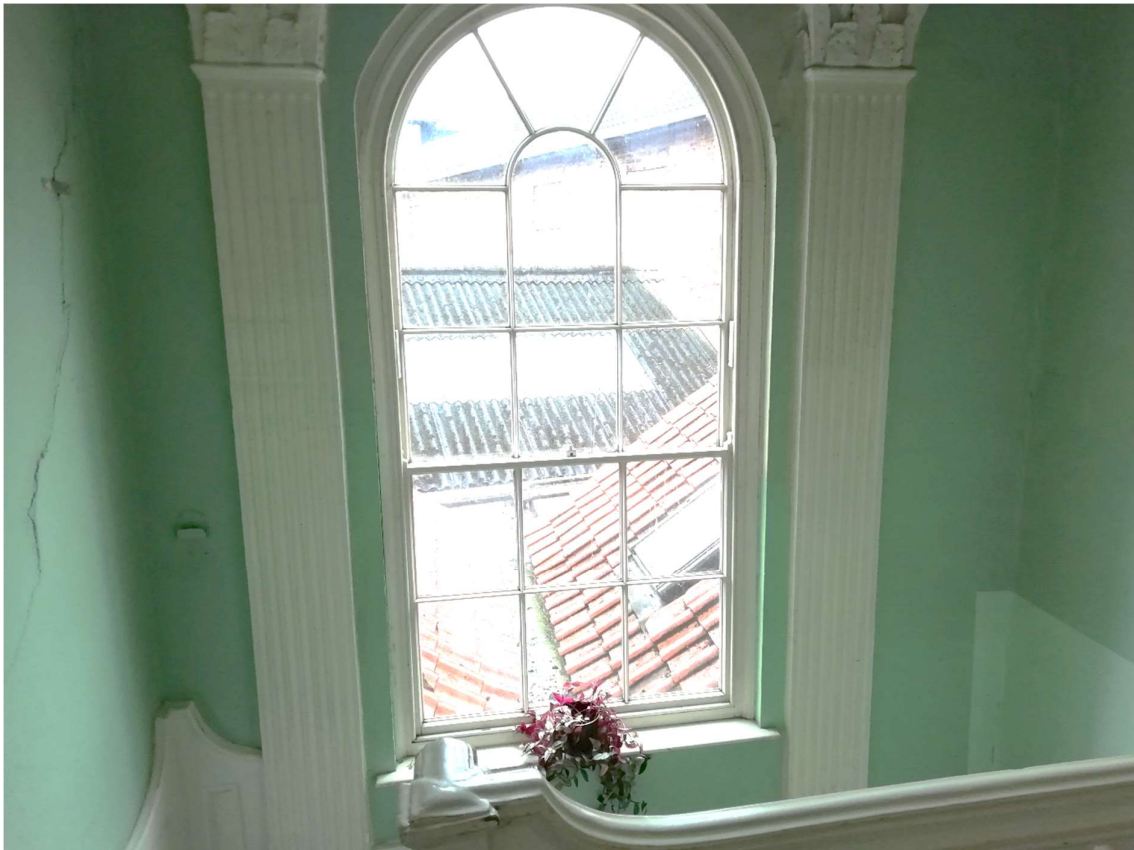
Fig 23 Elegant stair window flanked by Corinthian columns (cracks to walls to be tied and pointed)
