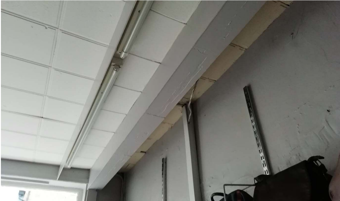
Fig 28 Modern ceilings to ground floor to be removed to expose historic floorboards behind and to better reveal the original proportions of the room
