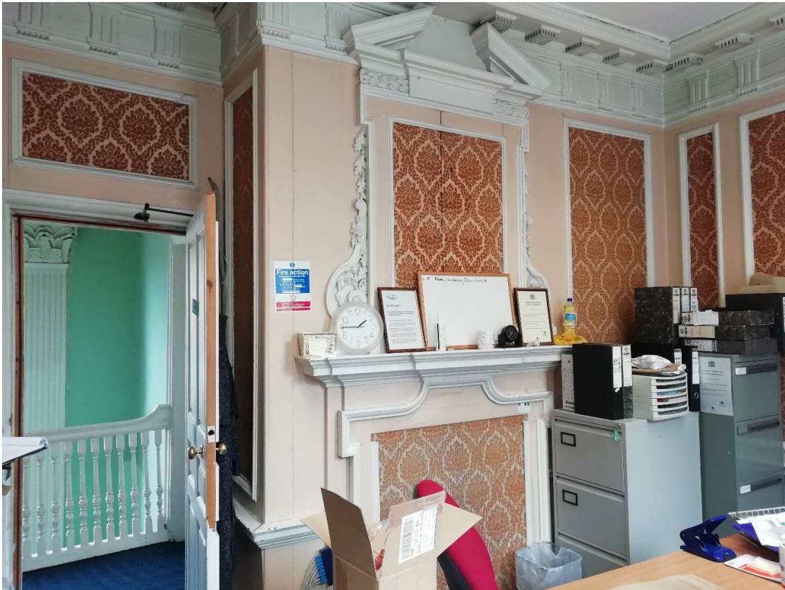
Fig 19A First floor, front, right hand room (fireplace to be re-opened & modern radiator replaced)
