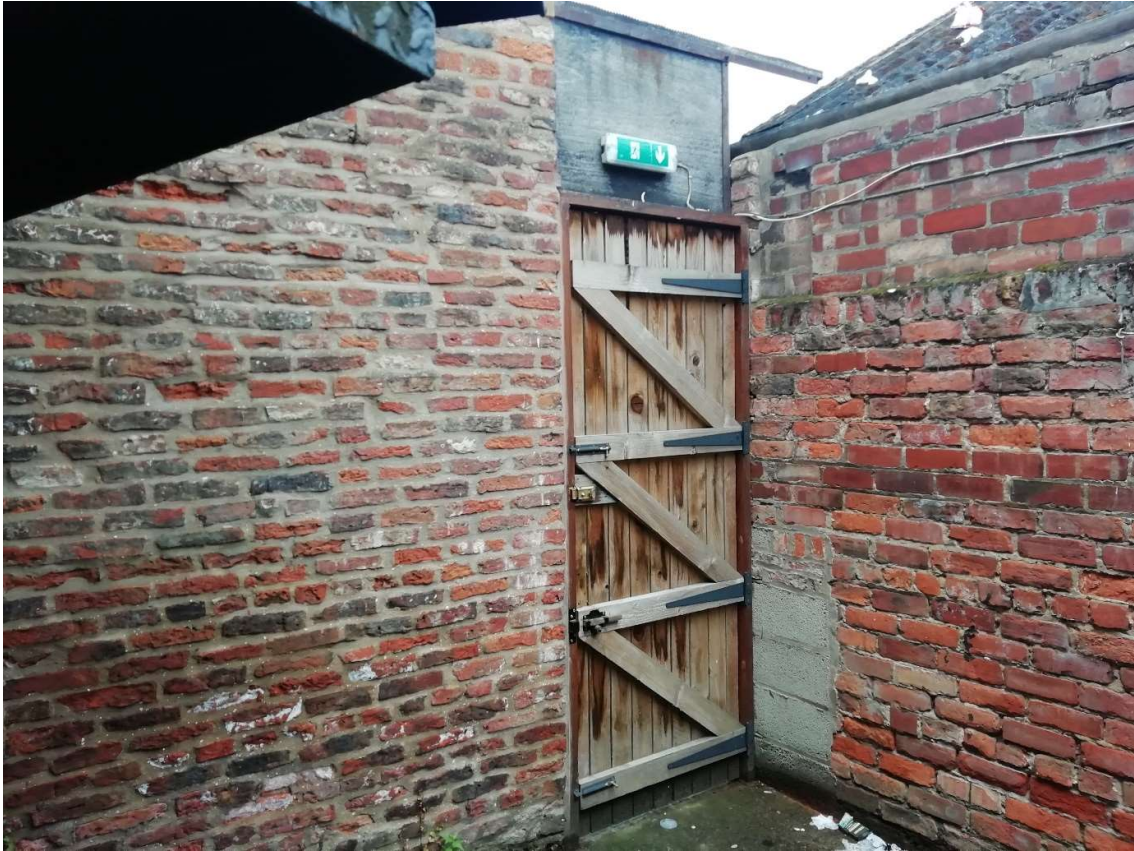
Fig 33A Barbed upper section removed, brick arch with coping to be formed over gate and gate replaced
