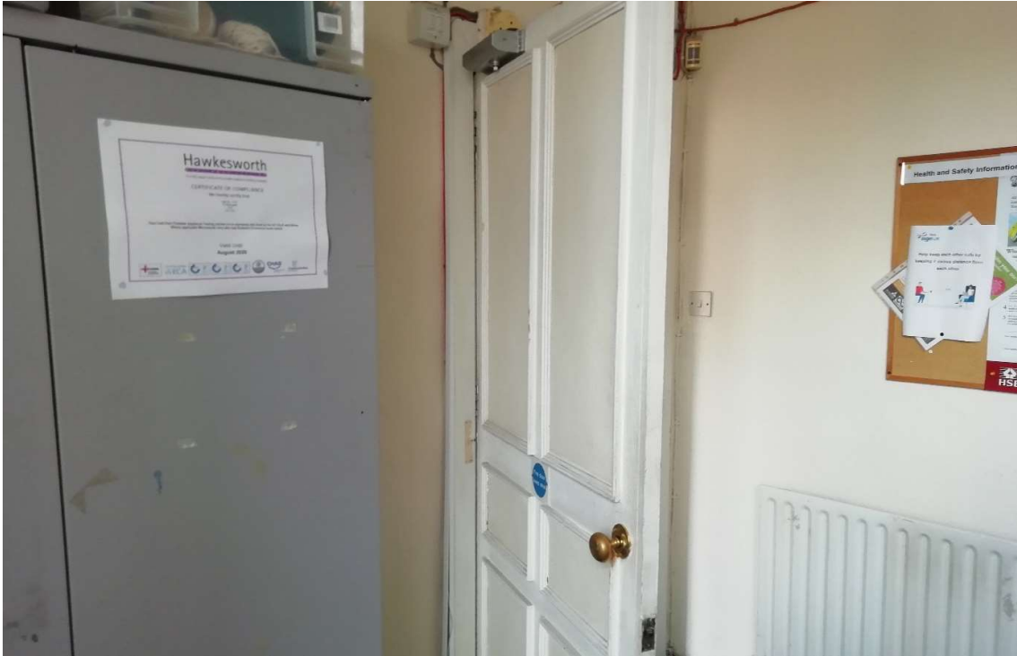
Fig 21A Applied fire panels and door closers to be removed from all first floor doors, fire resistance to be achieved using intumescent products
