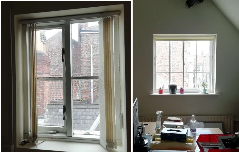
Figs 29B & C Modern, attic gable window replaced with Yorkshire sliding sash as per other gable window
