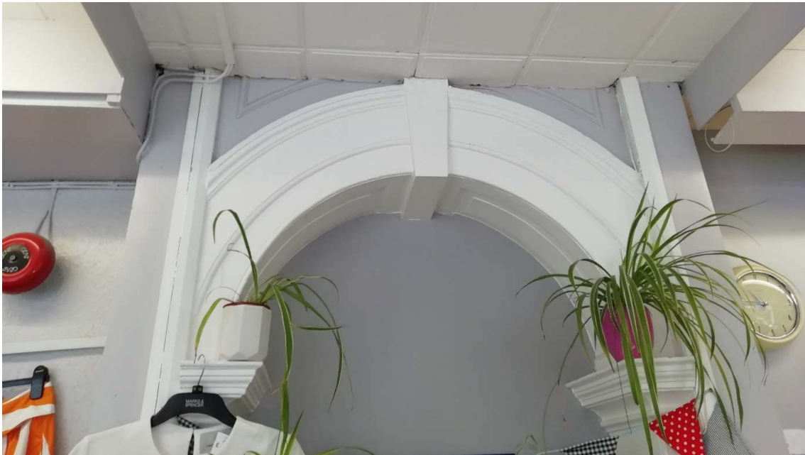
Fig 29 Ceiling tiles to shop bisect beading above blocked stair bay doorway-to be revealed
