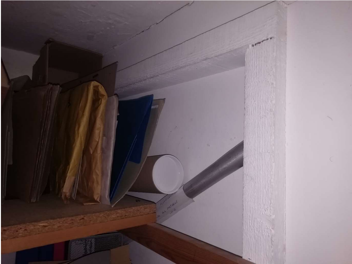
Fig 15 Blocked doorway from back stair to second floor, rear, lefthand room seen from cupboard (former back stair) off drawing room
