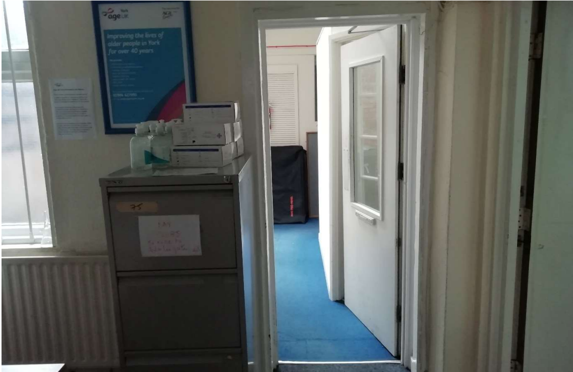
Fig 26 Ground floor, left hand, rear room. New door into rear extension and new door (to right) into stair bay to be blocked. The latter may also help address cracking in stair bay wall above
