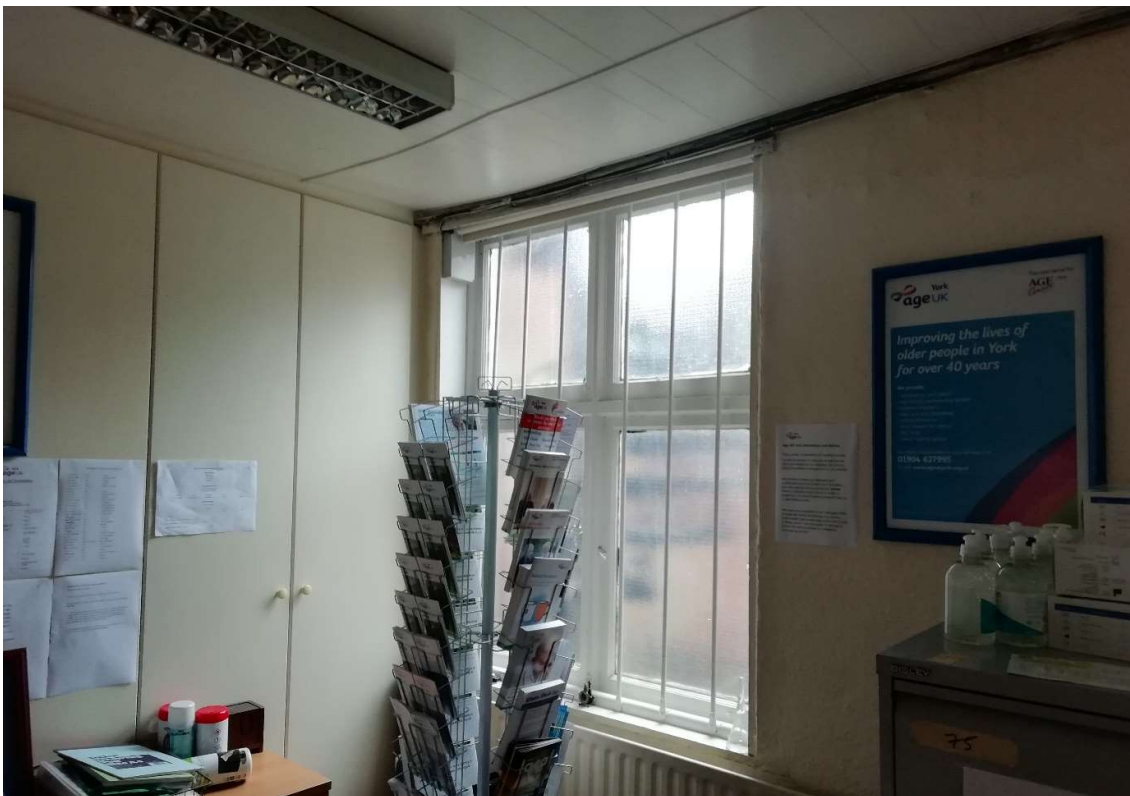
Fig 27 Ground floor, left hand, rear room. Modern cupboards, ceiling lining and window bars to be removed and window to be replaced with a vertical sliding sash window.
