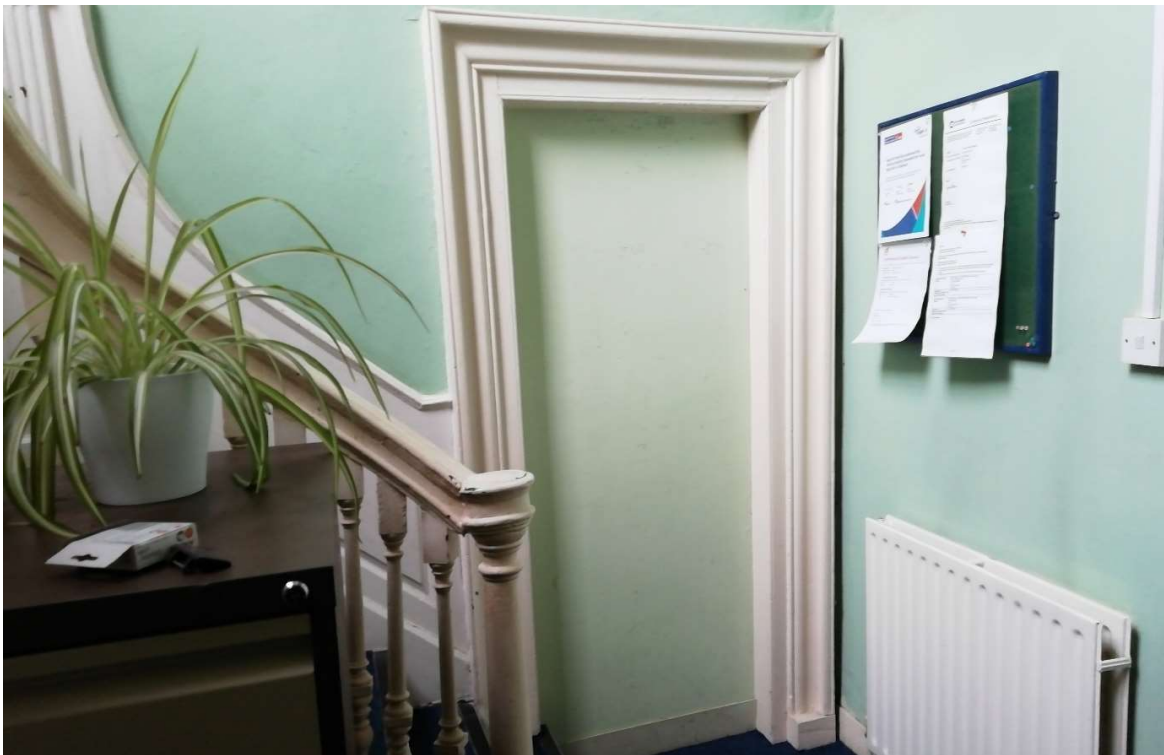
Fig 25 One of two blocked doors leading from stair bay hall to rear rooms (to be re-opened)
