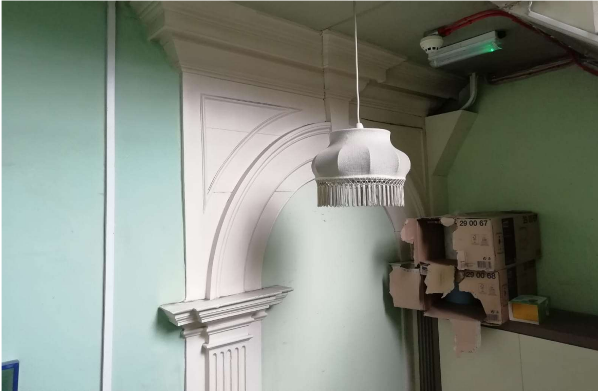
Fig 24 Looking from stair bay towards blocked doorway that originally led to a central hallway and on to the front door (door to be re-opened and trunking for electrics to be removed) Blocked door to rear, left hand room to right of this photo to be re-opened
