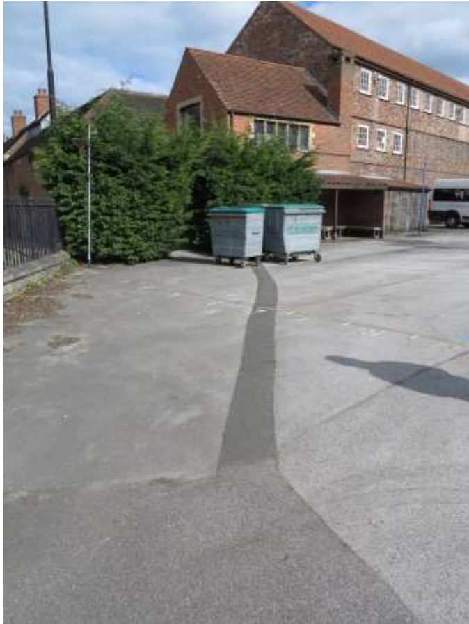
Above Fig 28: Cable trench route shown in tarmac in school yard
