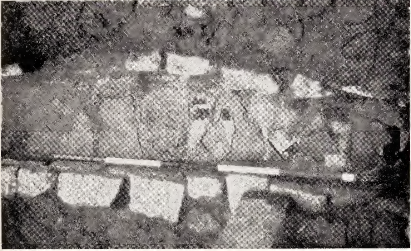
PLATE XXIX. Detail of the 'floor' of the culvert near Q1. The top end of the sur- veyor's pole lies on a tegula .
