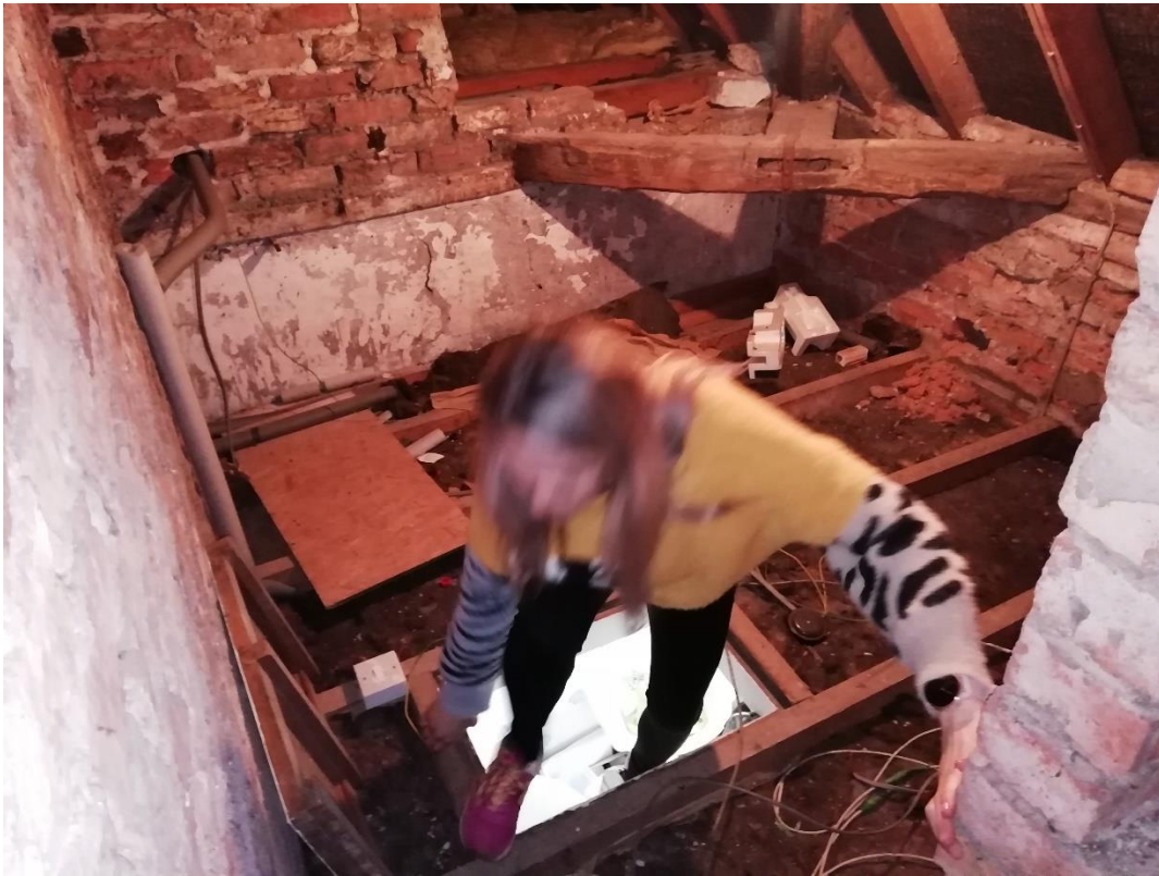
Fig 33 Plastered back stair bay with modern ceiling inserted and later, brick gable to the replacement service wing beyond
