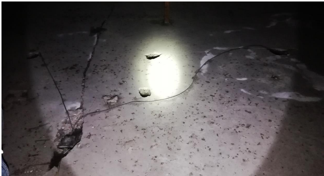
Fig 34 Limecrete floor referred to in original plans (Appendix D) to be conserved in situ
