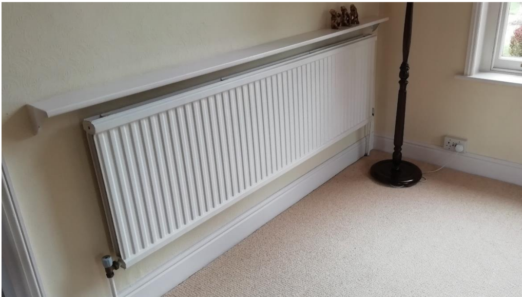
Fig 42 Modern radiators to be replaced with cast iron
