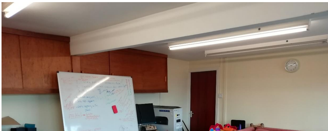
Fig 39 Downstand in northern range in location of proposed, internal wall
