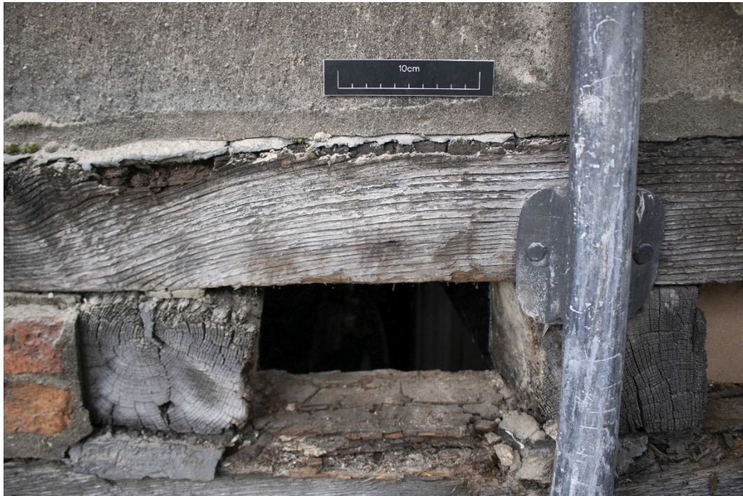
Plate 4 Void behind re-set brickwork between joists at 2 nd floor level, facing north-west, 0.1m scale
