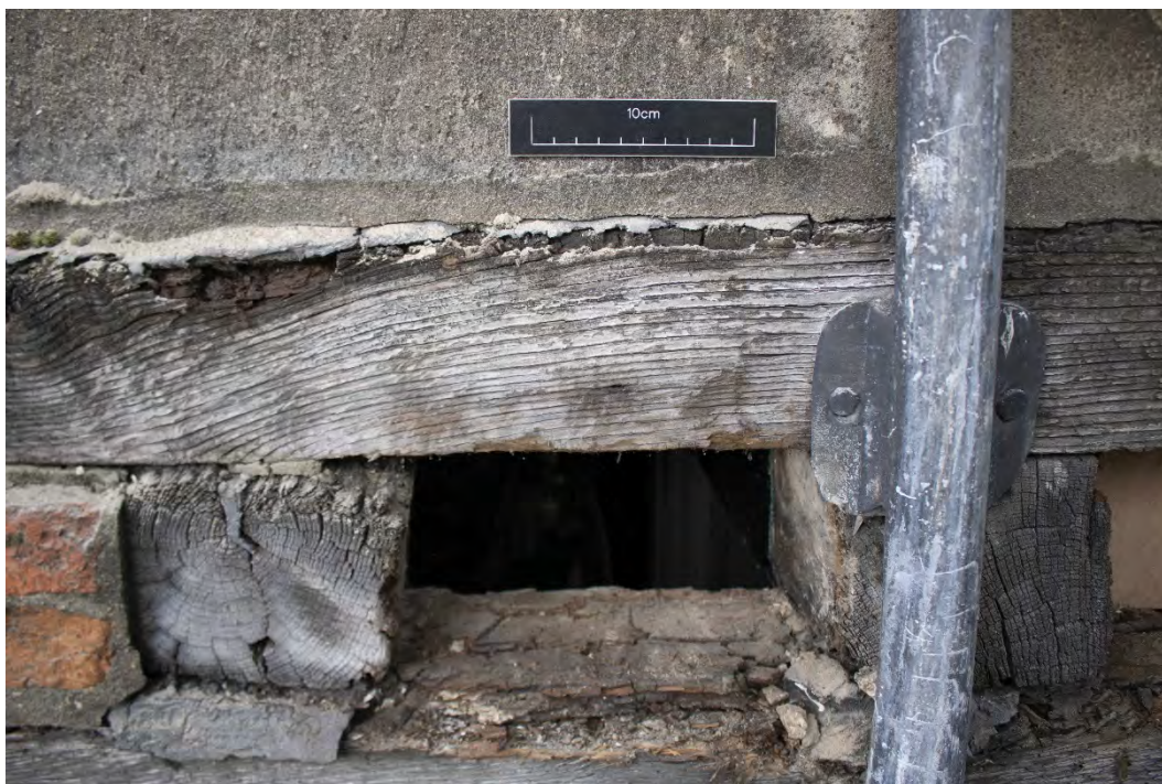
Plate 4 Void behind re-set brickwork between joists at 2 nd floor level, facing north-west, 0.1m scale
