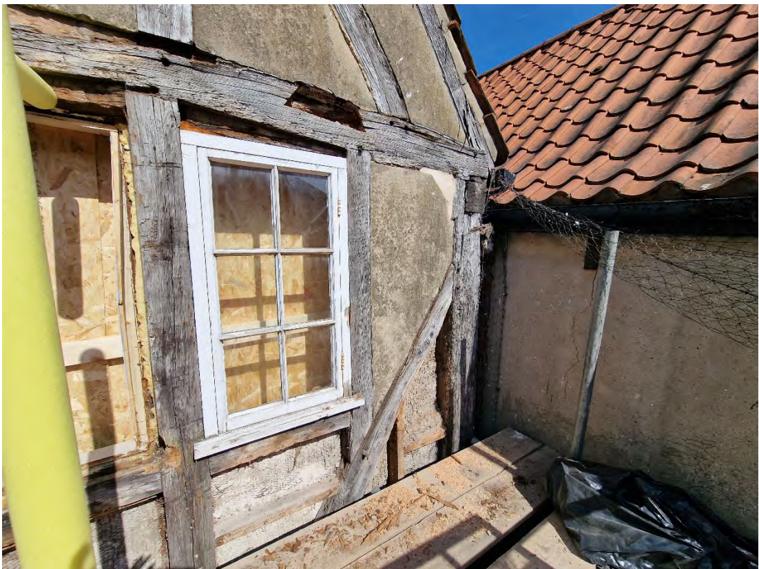
Plate 12: Northeastern side of the second floor during the partial removal of infill panels
