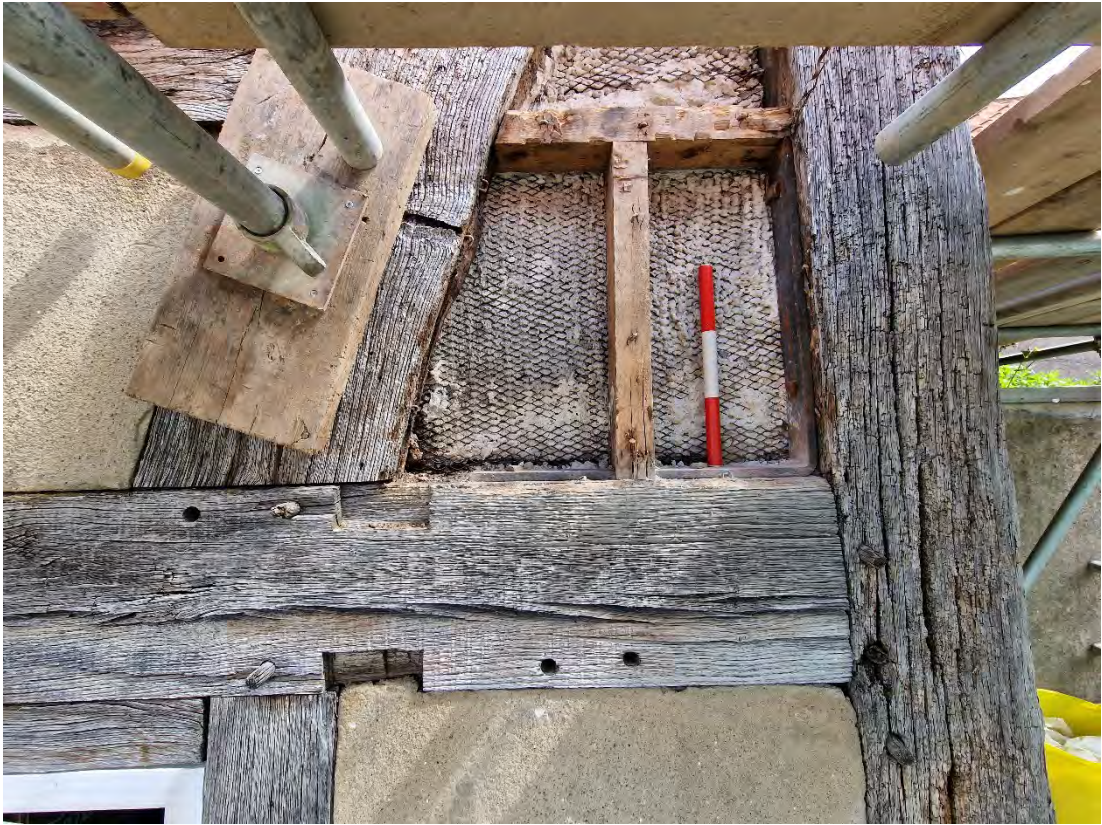
Plate 43: Partial removed infill panel within the southwest elevation with iron bracket
