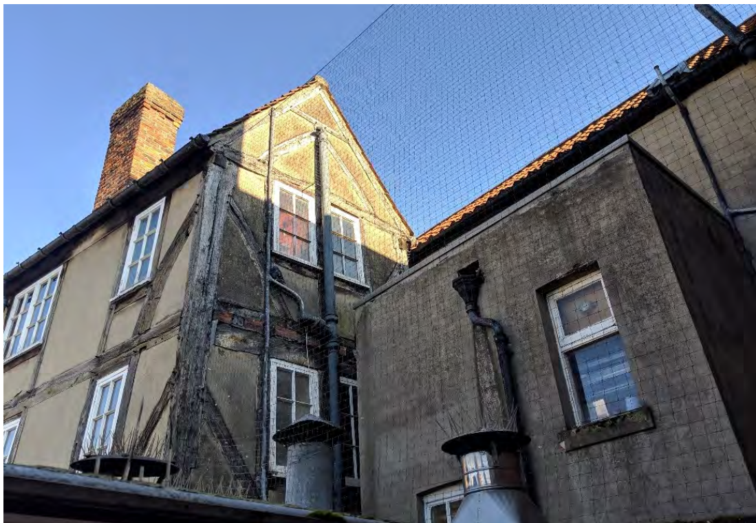
Plate 2: Rear elevation photographed in 2019 prior to the repair work (courtesy of Mason Clark Associates)
