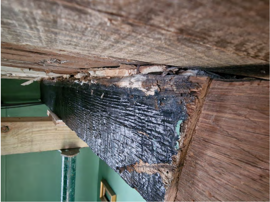
Plate 41: Additional view of ceiling joist inside the first floor with plaster ceiling over it
