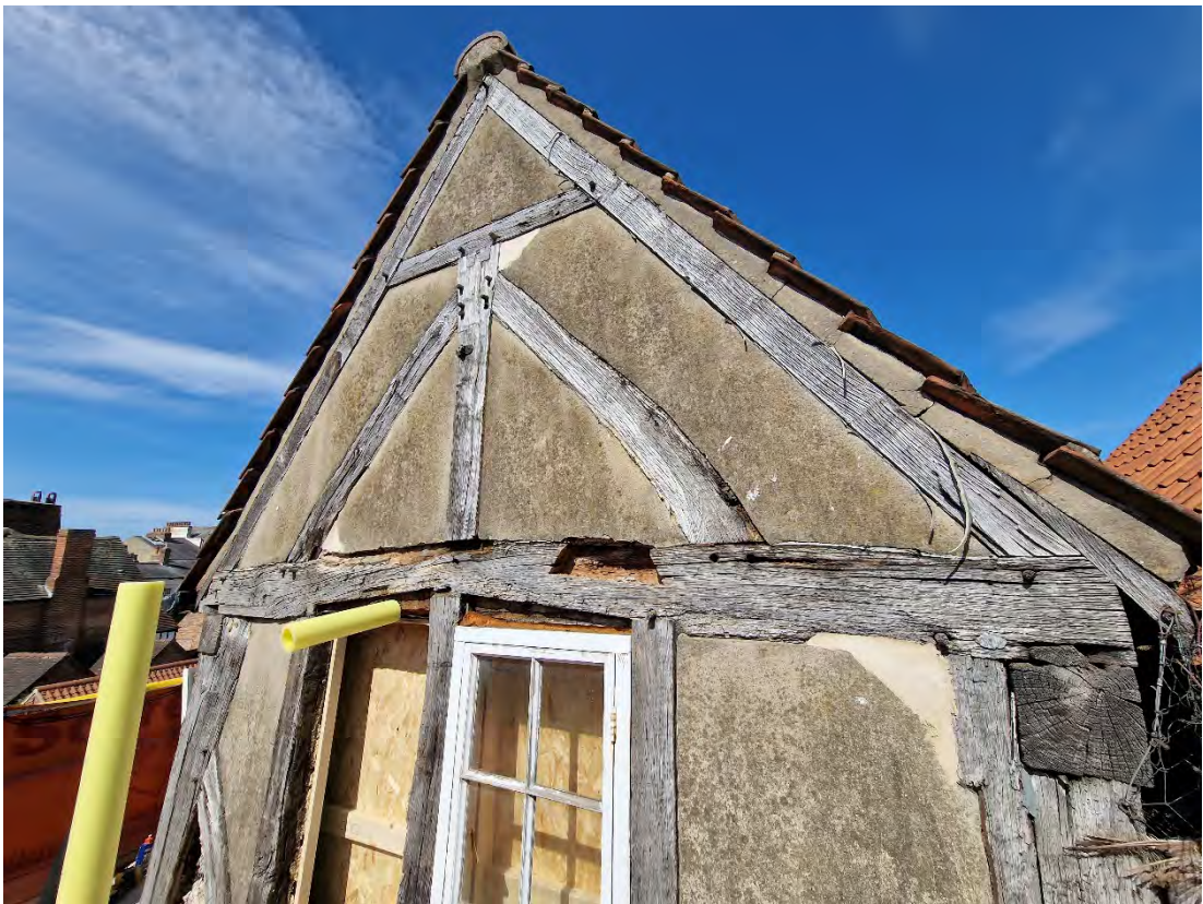
Plate 10: Joint between the tie-beam 5 and principal post 2 to the northeast end of the rear elevation
