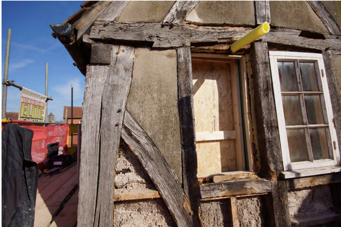
Plate 13: General view of the southwestern side of the second floor during the repair work
