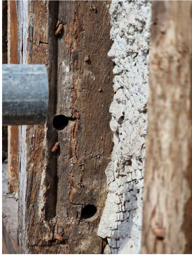
Plate 31: Detail of empty peg holes of former crown brace
