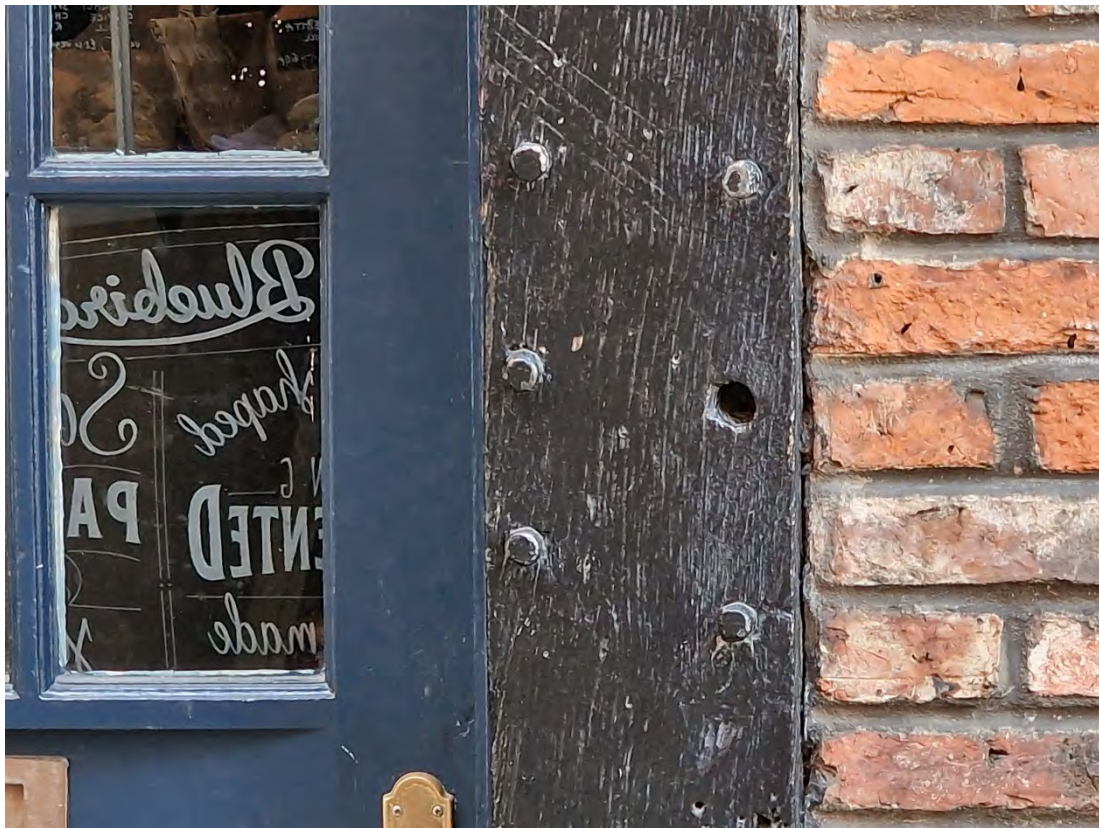
Plate 4: Detail of carpenter assembly's mark above the obsolete mortice joints with pegs and an empty hole
