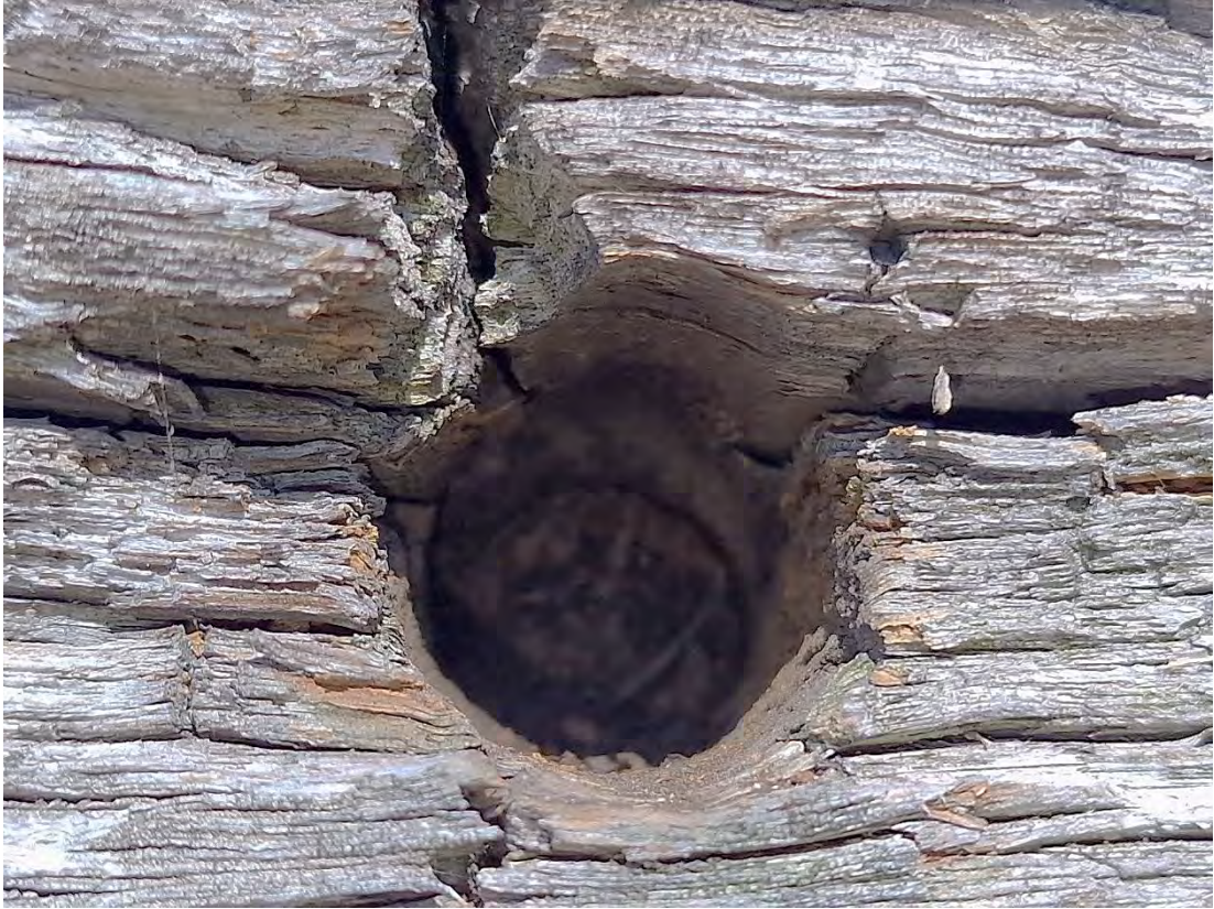
Plate 9: Detail of peg hole which does not pierce the tie-beam or extends through to a mortice
