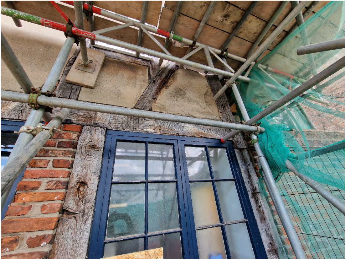
Plate 47: Southwest side elevation with truncated post 1 below the girding beam
