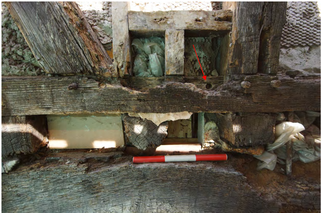
Plate 18: Central area of beam 6 with an empty peg hole and mortice (arrow)
