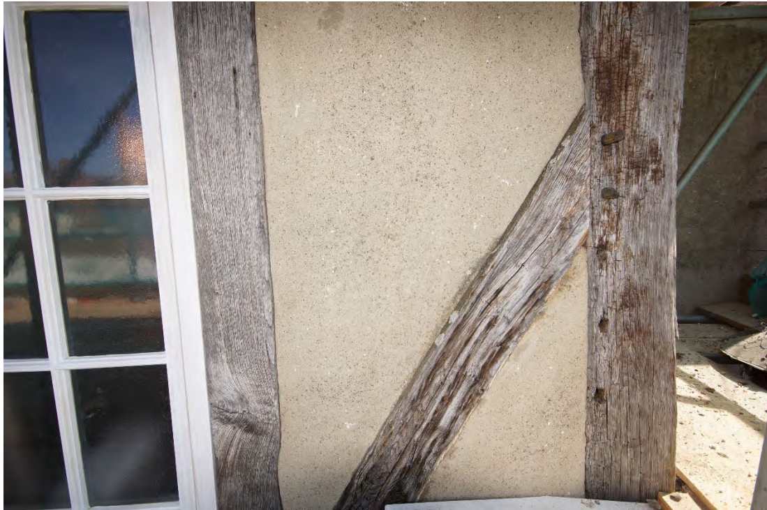
Plate 23: Southwest face of post 1 with empty peg holes of a vacant mortice
