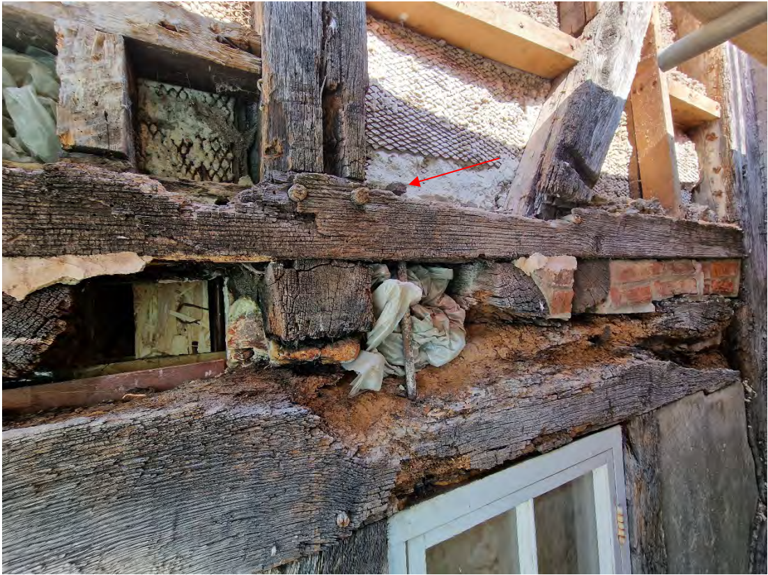
Plate 19: Later iron bolted rod securing beams 6 and 7 to the right of stud 17 (arrow)
