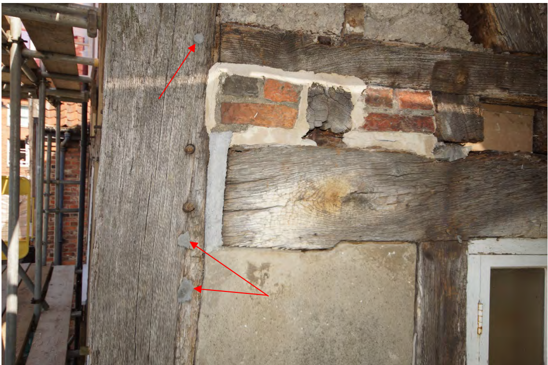
Plate 16: Peg holes filled with lead within post 1 (arrows)
