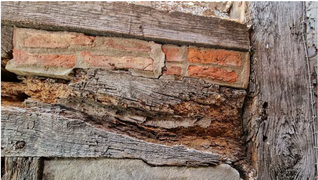
Plate 20: Chamfered northeastern end of beam 7 and empty peg holes within post 2
