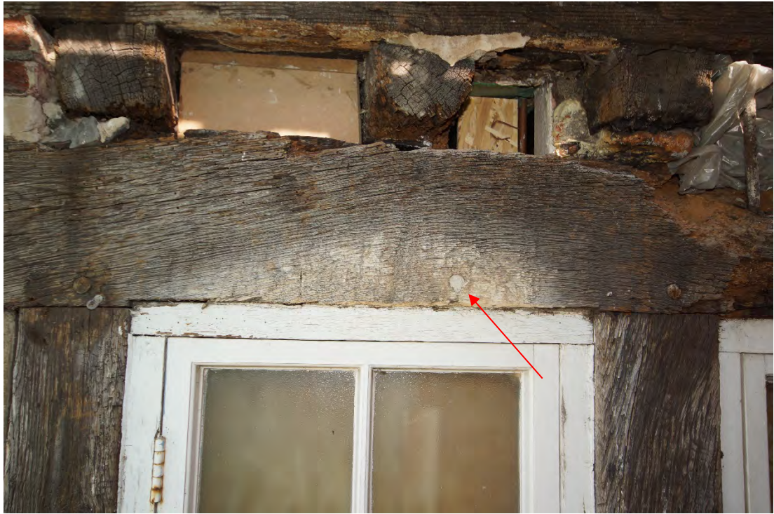
Plate 17: Beam 7 with vacant peg hole filled with lead (arrow)
