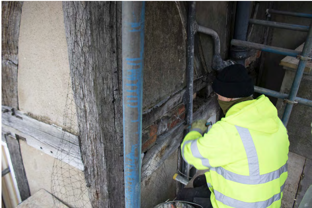
Plate 2 Removal of re-set brickwork between 2 nd floor joists and upper and lower rails, facing north
