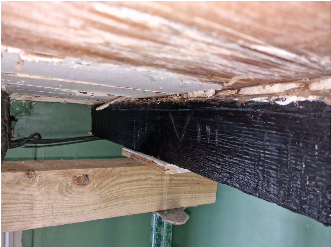
Plate 42: Ceiling joist with carpenter's mark VIII and plaster ceiling directly above it
