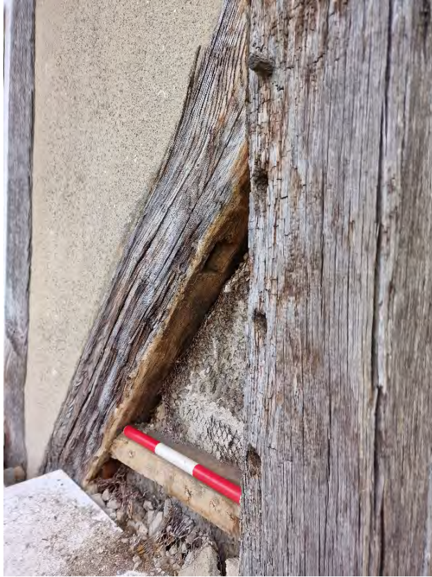
Plate 45: Empty small mortice within brace on the southwest elevation to post 1
