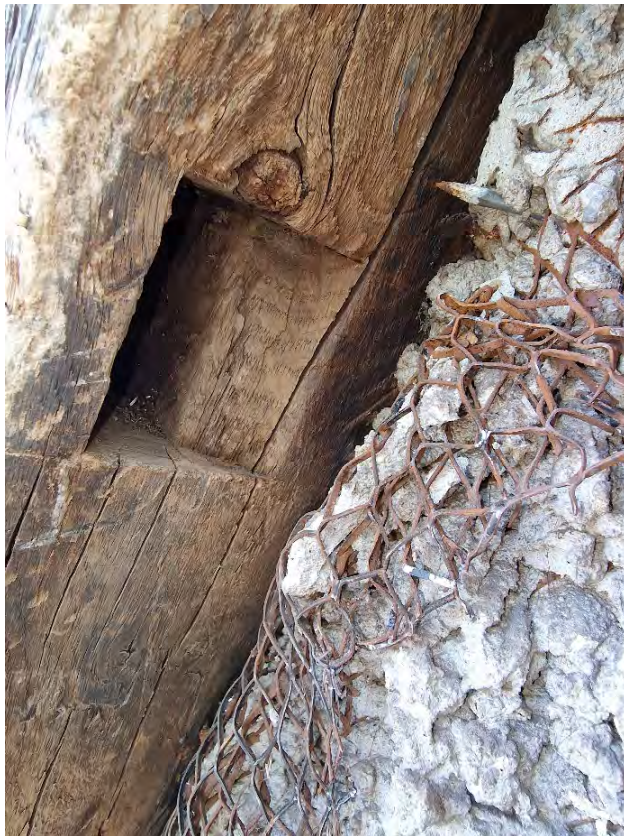
Plate 46: Detail of mortice within the underside of brace to the southwest face of post 1
