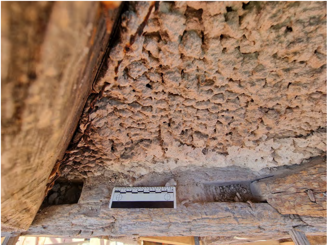
Plate 32: Tie-beam with partial empty mortice for rafter 3 and crudely incised housing for gable brace 9
