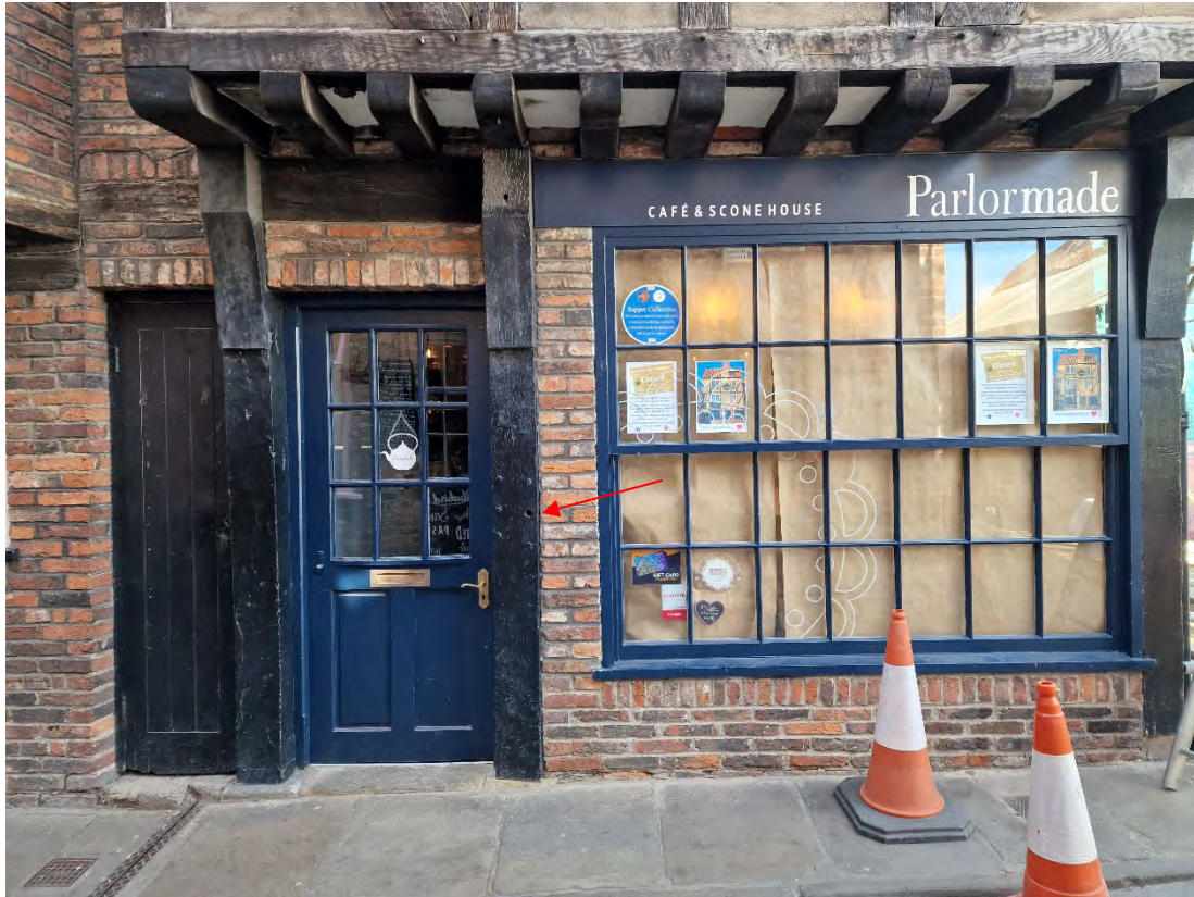
Plate 3: Shopfront with reused post comprising an obsolete mortice with pegs and an empty hole (arrow)
