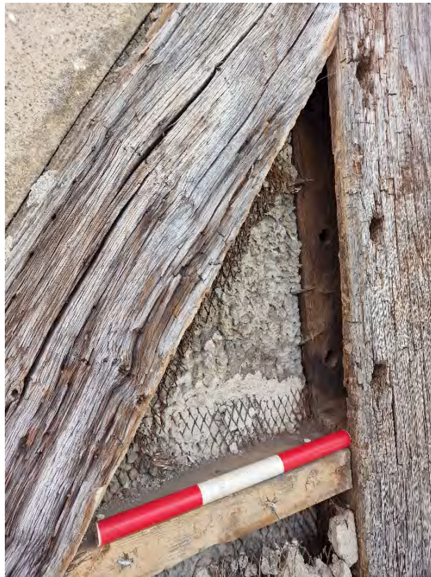
Plate 44: Detail of empty mortise within the southwest face of post 1
