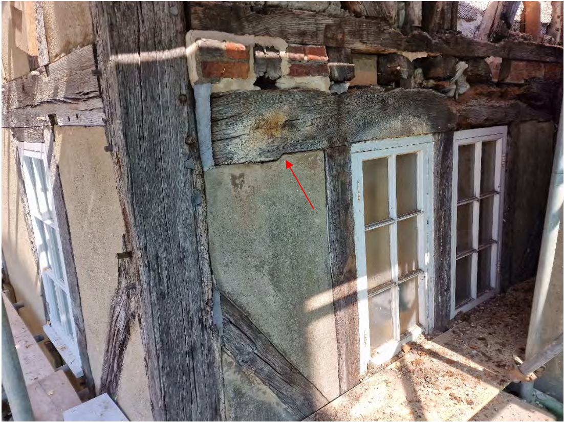
Plate 15: Chamfered edge within the southwestern end of beam 7 (arrow) adjacent to post 1
