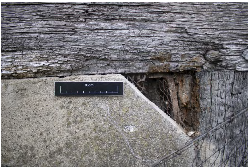
Plate 3 View of inspection cut-away in mid-20 th century render infill panel, facing north, 0.1m scale
