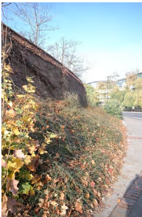
Plate 15 The brick wall at the northern end of the south-eastern side of Plot A, facing north-west
