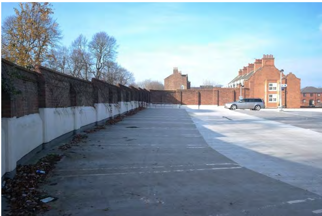
Plate 70 The brick wall surrounding the south-western side of the upper storey of the three-storey car park, facing north-west
