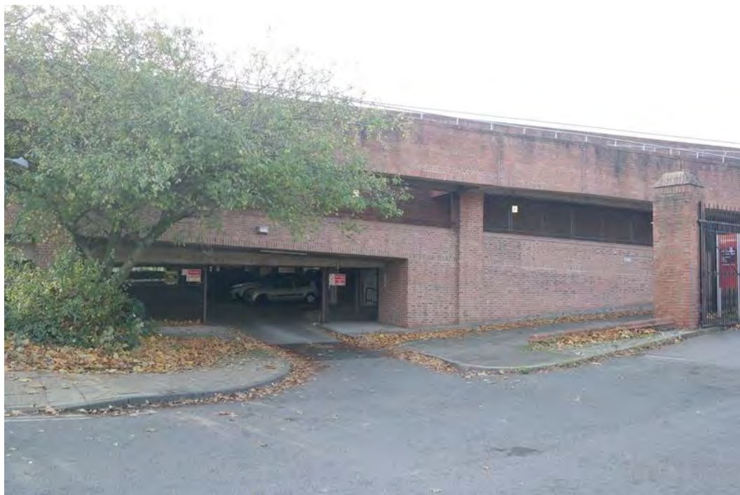
Plate 58 The north-western side of the multi-storey car park showing the exit, facing south-west
