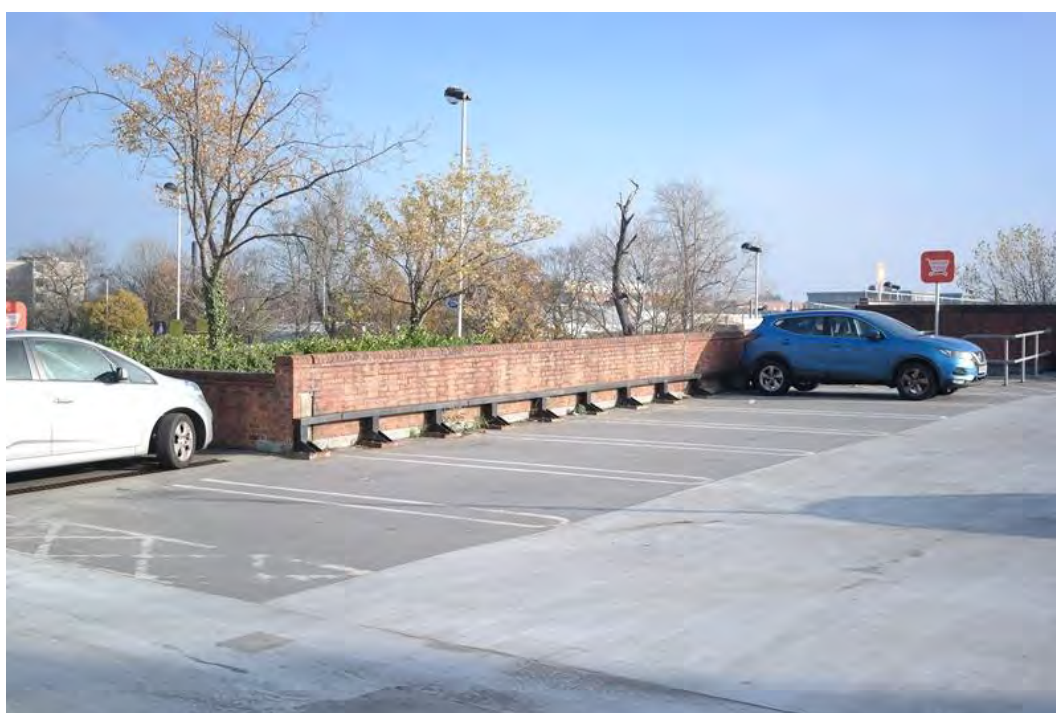
Plate 83 The brick wall around the north-eastern side of the upper floor of the two-storey car park to the east of the ramp leading into the Sainsbury's car park, facing east
