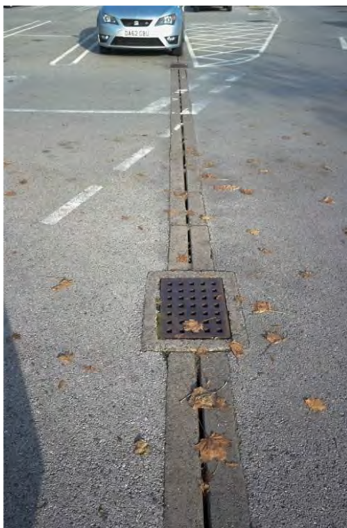
Plate 43 A drain and associated grid in the car park of Plot A, facing south-west
