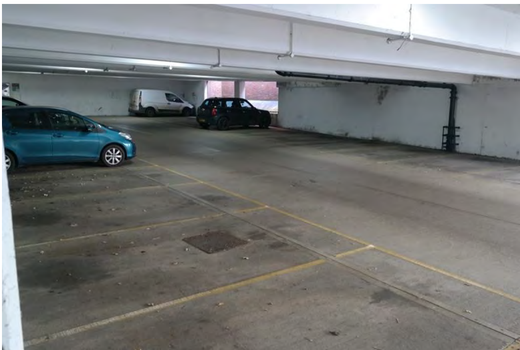
Plate 79 The north-eastern portion of the ground floor of the two-storey car park, facing north-west
