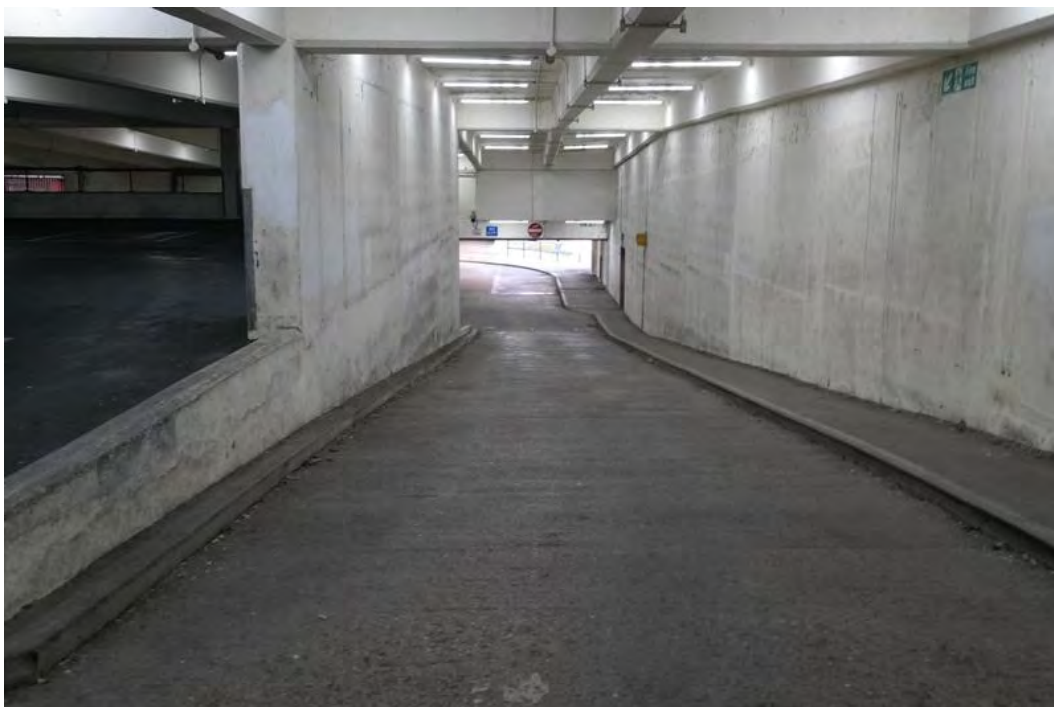
Plate 64 The access ramp down from the first floor to ground floor of the three-storey car park, facing north-west
