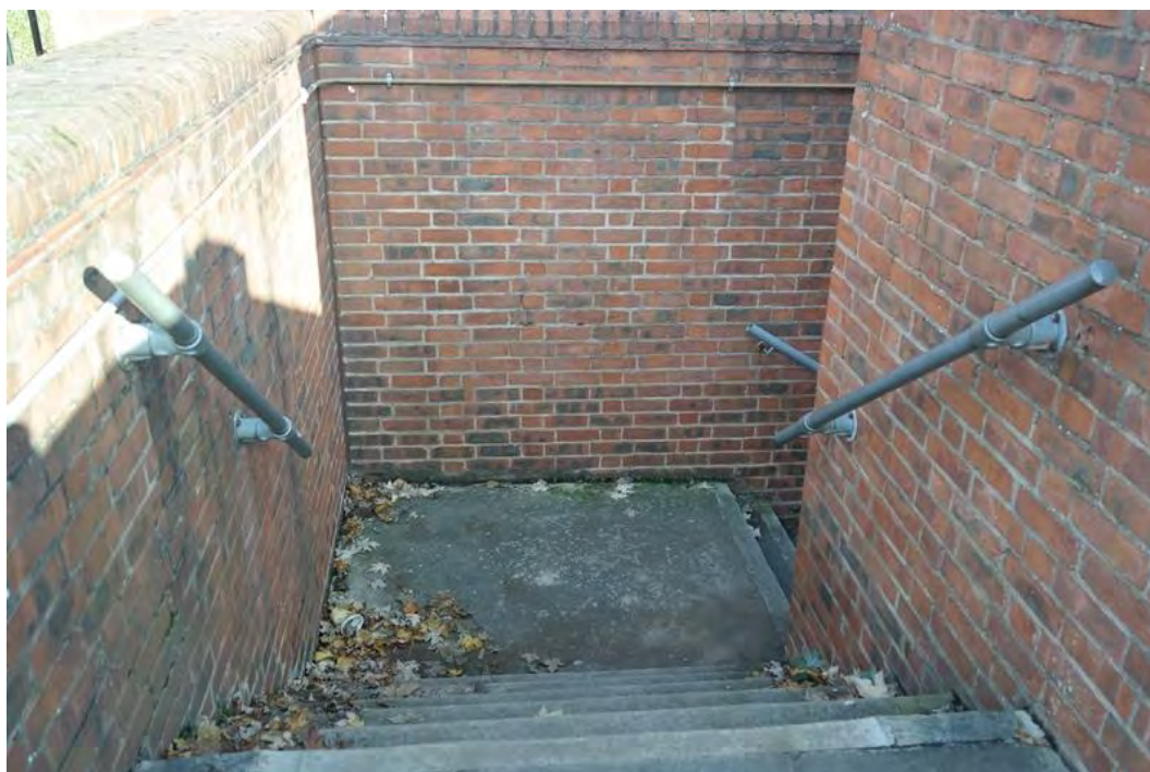
Plate 74 The upper part of the pedestrian access into the ground floor of the car park on the north-western side, facing north-east
