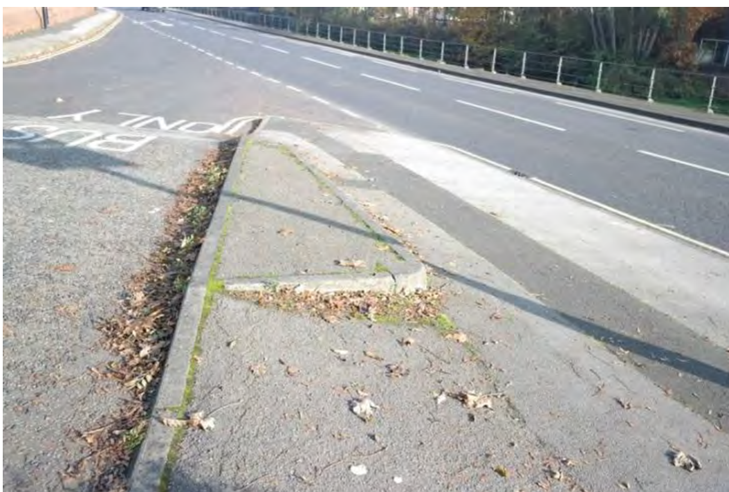
Plate 49 The uneven pavement adjacent to the bus layby entrance, facing north-east
