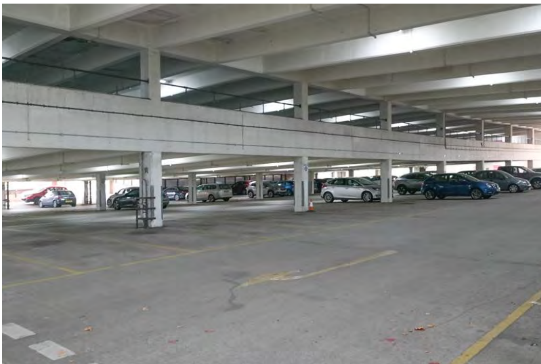
Plate 66 The north-eastern wall of the first floor of the three-storey portion of the car park, facing south-east
