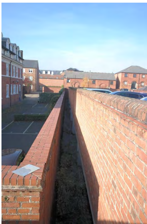
Plate 73 The property boundary wall to the north-east of Feversham House with the adjacent car park wall, facing north-west
