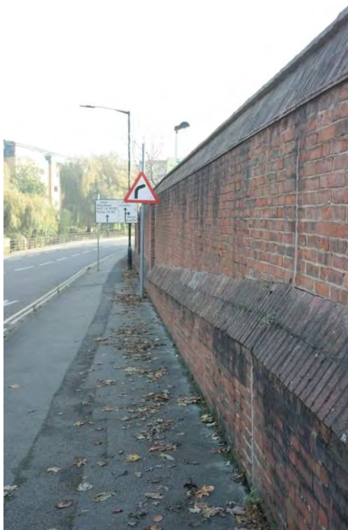
Plate 14 The brick wall between the north-eastern side of the site and Foss Bank, facing south-east
