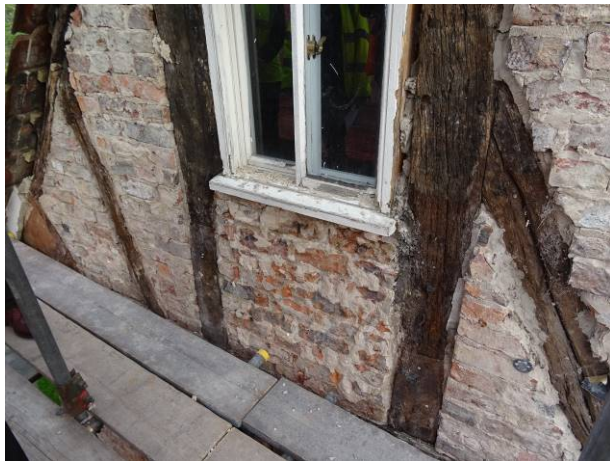
35 - Degraded structural timbers at LHS elevation and window
