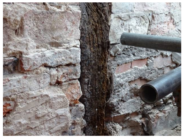
22 - Degraded structural timbers at LHS elevation
