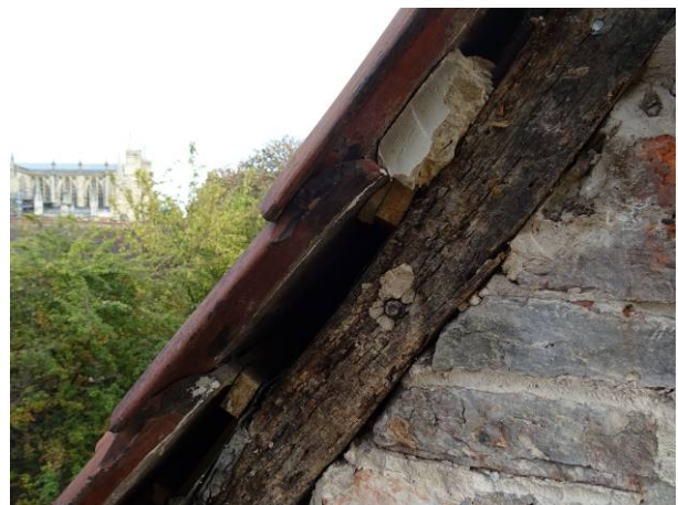
40 - LHS elevation – degraded timbers
