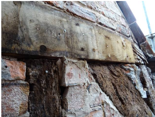
108 - LHS elevation – previous timber repairs
