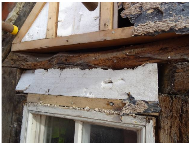
37 - LHS elevation – degraded timbers, window, gable timbers and polystyrene infill
