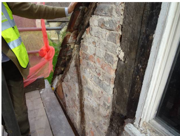
39 - LHS elevation – degraded timbers and infill brickwork
