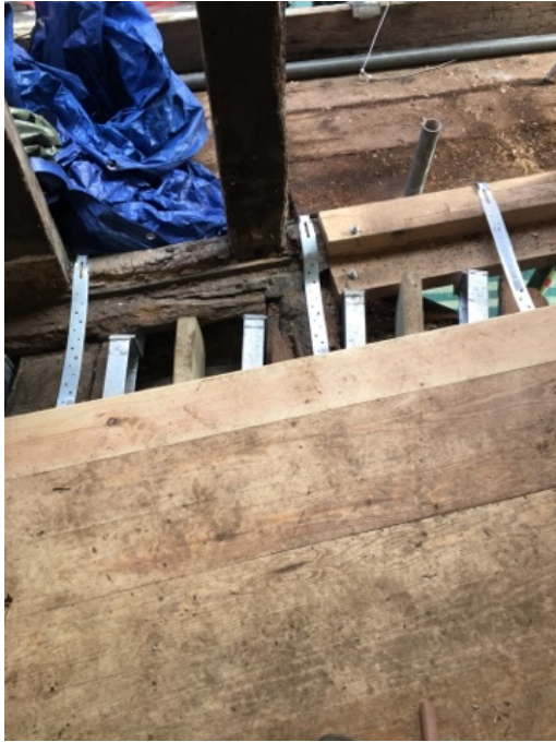
168 - New straps installed to the front of the property to tie into the structure
