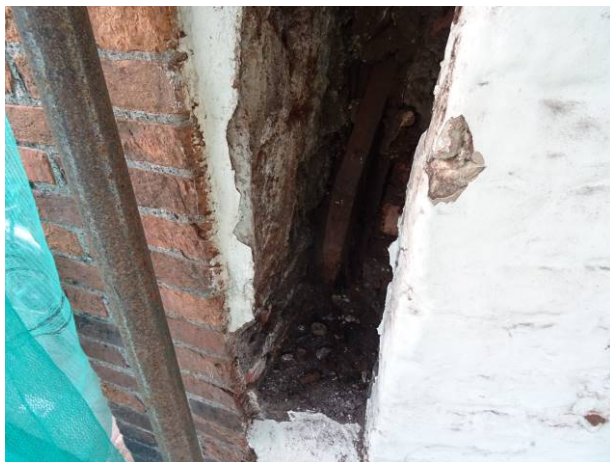
162 - Void remaining following the removal of the corner post at front LHS corner
