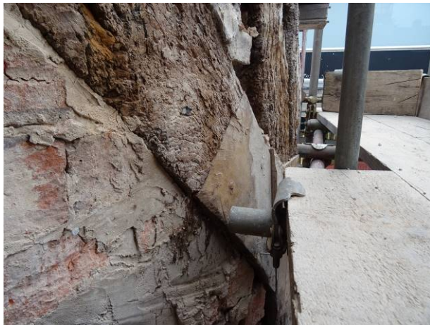
29 - Degraded structural timbers and previous repairs at LHS elevation
