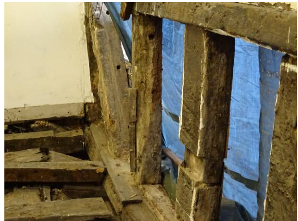
83 - Internals – snapped joist ends at jettied structure at first floor level and exposed timbers
