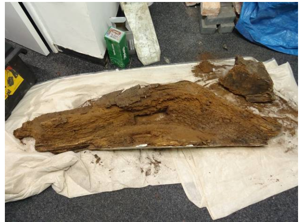
149 - Decayed corner post
