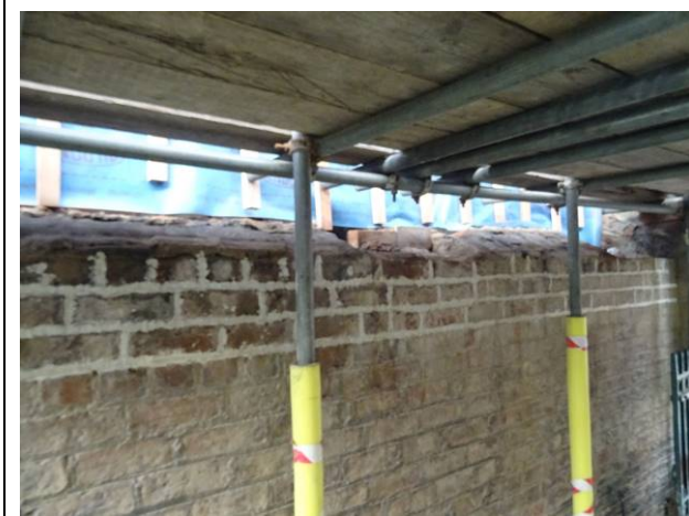
186 - Top 3 courses of brick work installed, new breather membrane and timber battens installed
