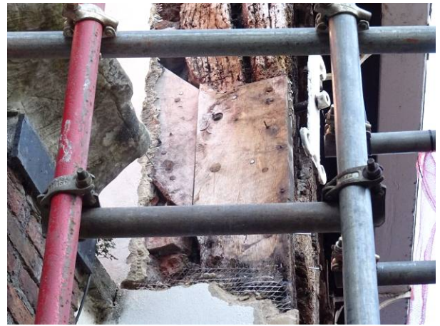
12 - LHS corner showing previous repairs
