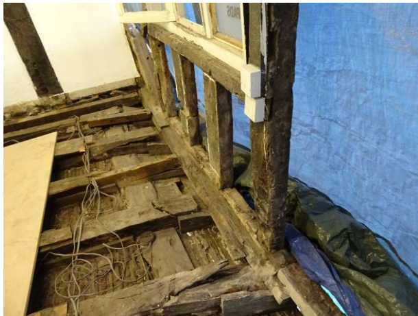
82 - Internals – snapped joist ends at jettied structure at first floor level
