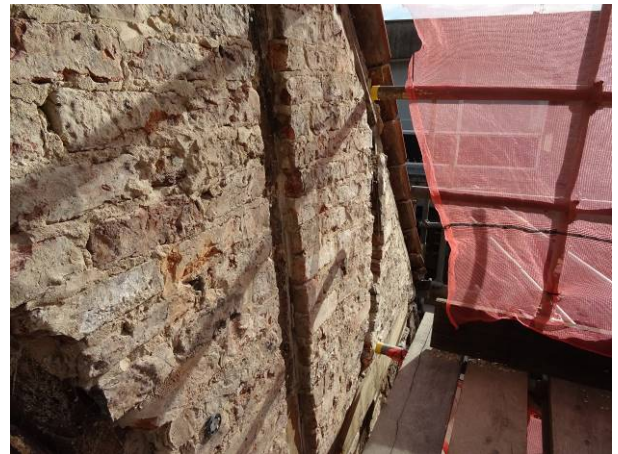
48 - LHS elevation – degraded timbers and infill brickwork
