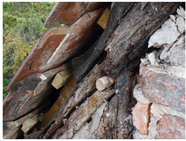
42 - LHS elevation – degraded timbers
