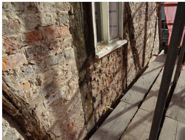
45 - LHS elevation – window, degraded timbers and infill brickwork
