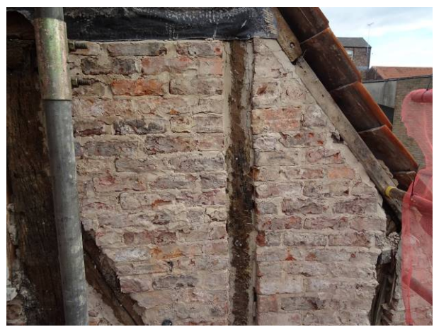
32 - Degraded structural timbers and previous repairs at LHS elevation
