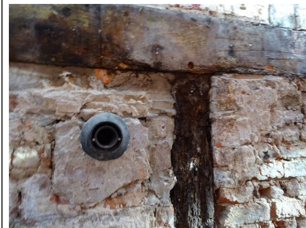
21 - Degraded structural timbers at LHS elevation
