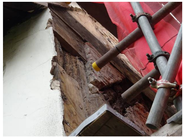
18 - Timbers at LHS elevation with previous repairs
