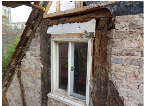
36 - Degraded structural timbers at LHS elevation and window
