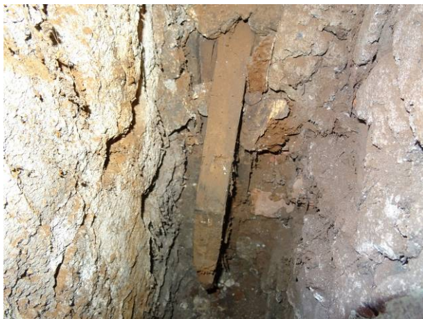
164 - Void remaining following the removal of the corner post at front LHS corner
