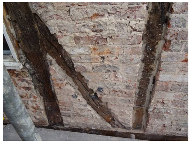
34 - Degraded structural timbers at LHS elevation
