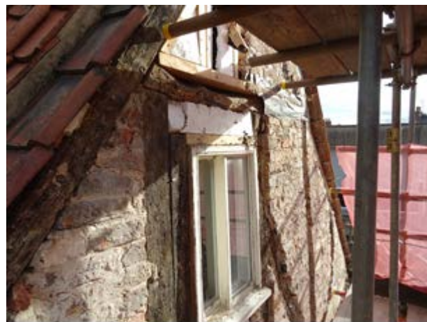
46 - LHS elevation – window, degraded timbers and infill brickwork
