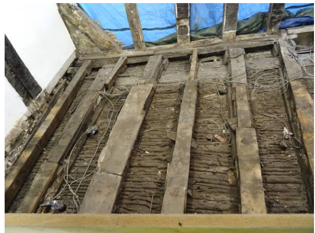
87 - Internals – snapped joist ends at jettied structure at first floor level and exposed joists and timbers
