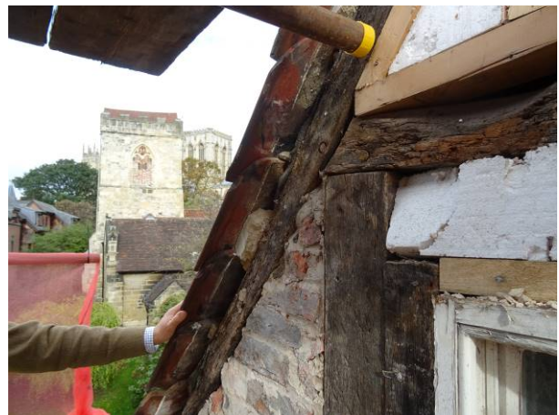
38 - LHS elevation – degraded timbers, window, gable timbers and polystyrene infill
