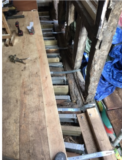
169 - New straps installed to the front of the property to tie into the structure
