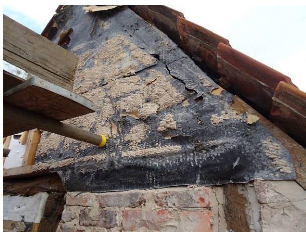
31 - LHS elevation with assumed builder's paper and bitumen paint from previous repair
