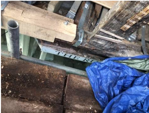
170 - New straps installed to the front of the property to tie into the structure
