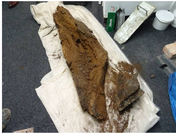
148 - Decayed corner post
