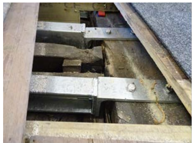
152 - Steel channels tied into the central beam (at the centre of the property).
