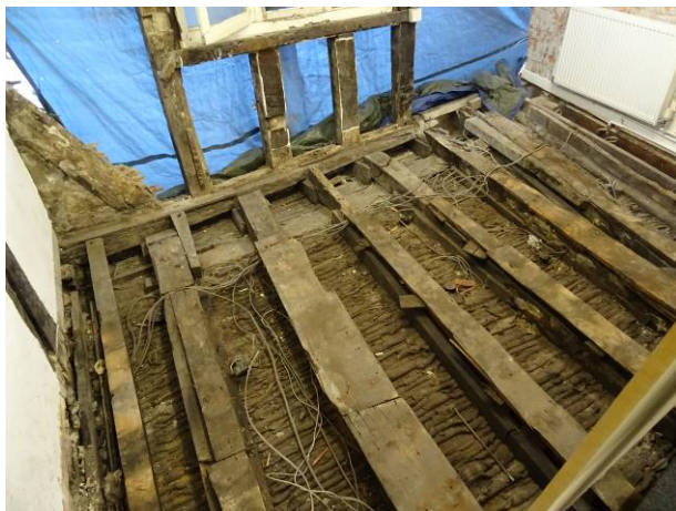
86 - Internals – snapped joist ends at jettied structure at first floor level and exposed joists and timbers
