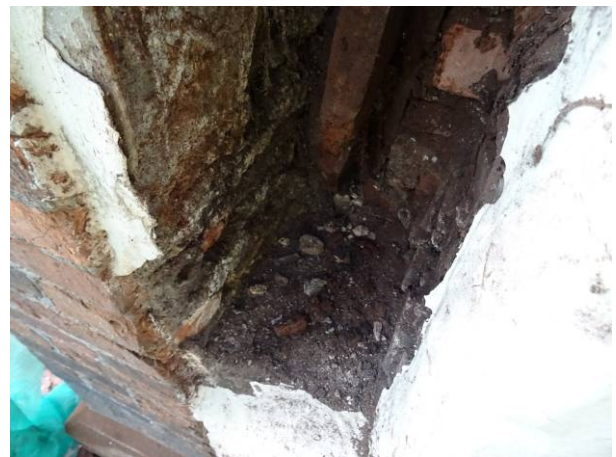
163 - Void remaining following the removal of the corner post at front LHS corner
