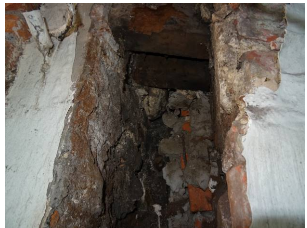
165 - Void remaining following the removal of the corner post at front LHS corner
