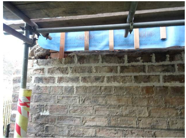
185 - Top 3 courses of brick work installed, new breather membrane and timber battens installed
