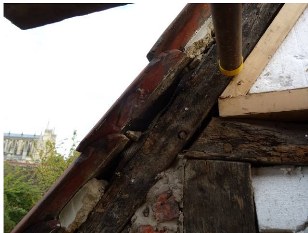
41 - LHS elevation – degraded timbers
