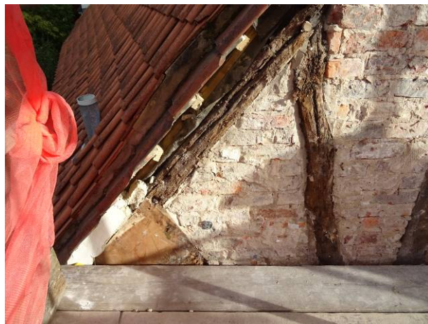
43 - LHS elevation – degraded timbers and infill brickwork
