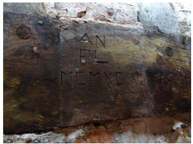
20 - Structural timbers at LHS elevation (previous repairs dated)
