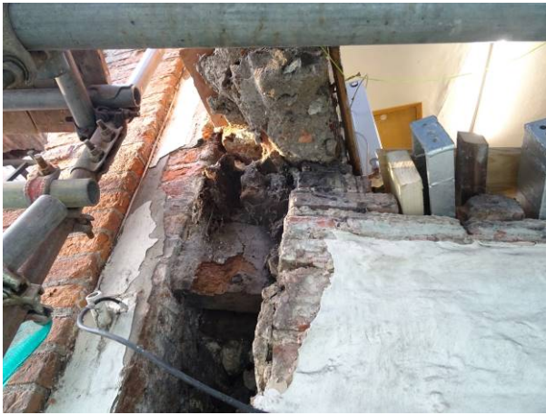
182 - Void remaining following the removal of the corner post at front LHS corner and underside of the jetty structure
