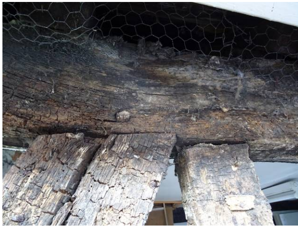
05 - Front elevation – degraded timbers
