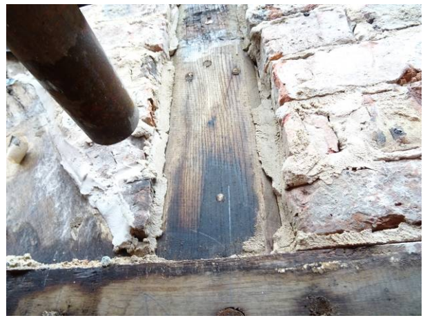
111 - LHS elevation – previous timber repairs
