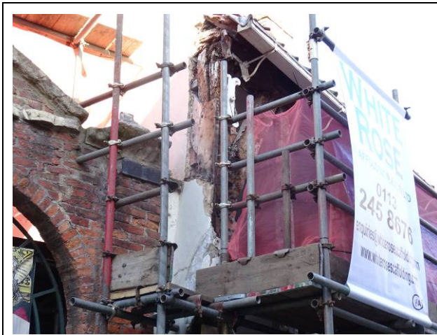
11 - LHS corner of property with previous repairs
