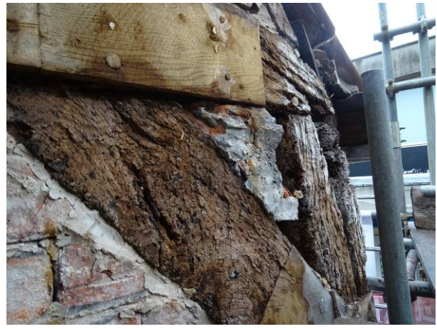
109 - LHS elevation – previous timber repairs
