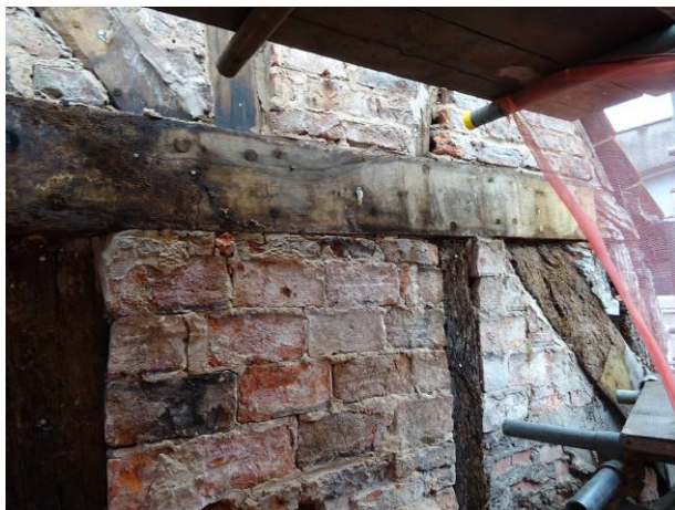
110 - LHS elevation – previous timber repairs
