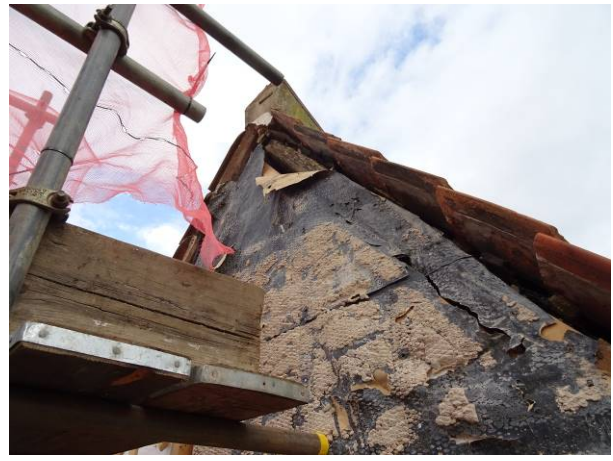
30 - LHS elevation with assumed builder's paper and bitumen paint from previous repair
