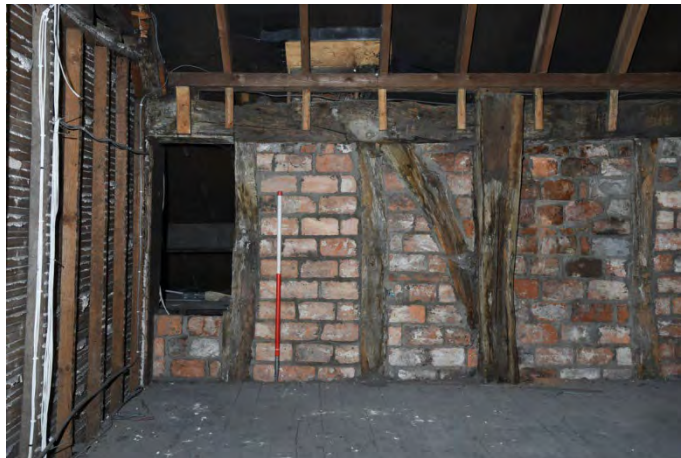
YCY042 Interior second floor looking northwest showing brace, wall plate, studs and post G (2m scale)
