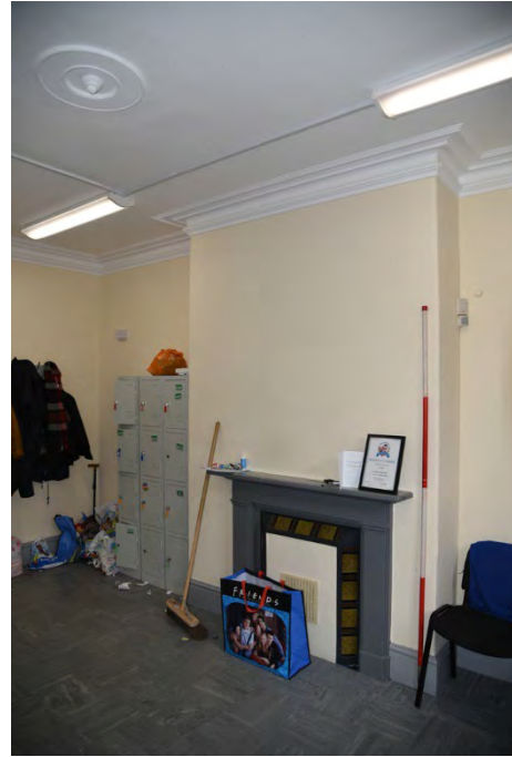
YCY028 Interior first floor looking north showing stack position and end wall (2m scale)
