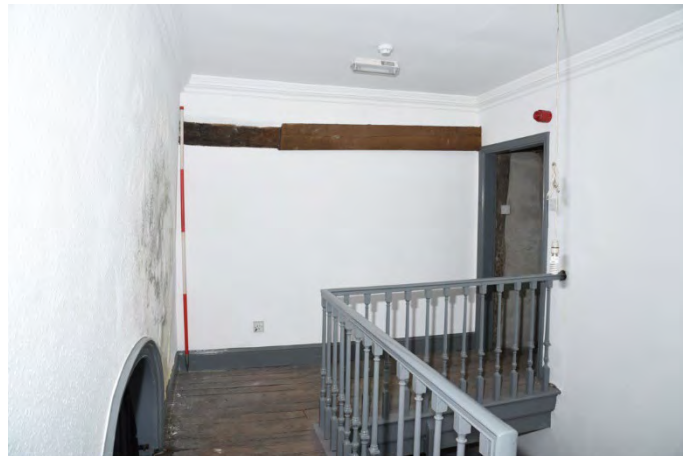
YCY029 Interior second floor looking northwest showing wall plate with replaced section (right) (2m scale)
