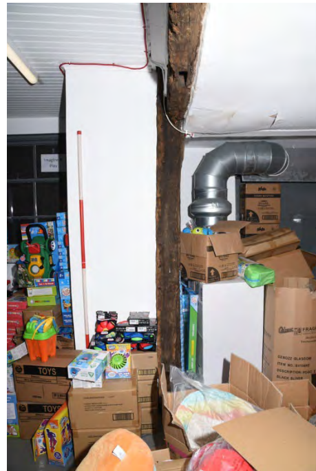
YCY016 Interior first floor looking north east showing post B and wall plate (2m scale)
