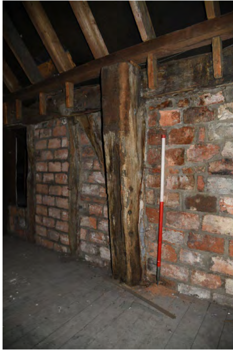
YCY048 Interior second floor looking west showing wall plate, arch brace, studs and post G (1m scale)
