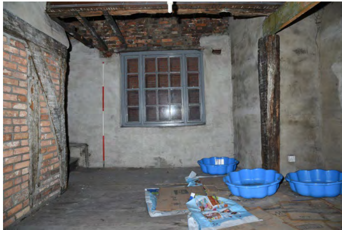
YCY032 Interior second floor looking northeast showing wall plate, arch brace and post D (left) and post F (right) (2m scale)
