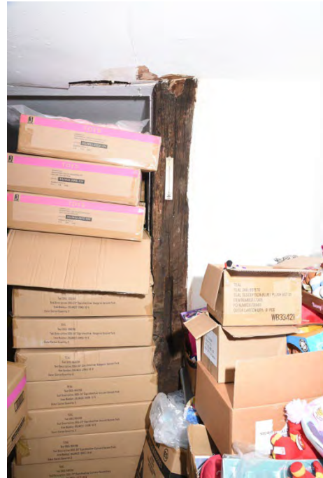
YCY020 Interior first floor looking northeast showing post C and wall plate
