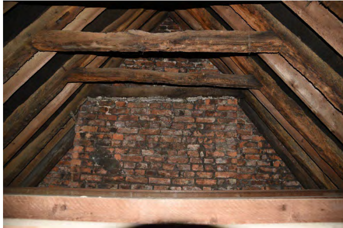
YCY049 Interior second floor looking south west showing southwest wall and collar roof trusses
