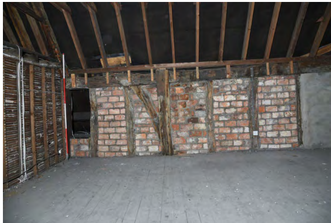
YCY041 Interior second floor looking northwest showing brace, wall plate, studs and post G (2m scale)
