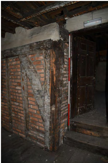
YCY038 Interior second floor looking west showing brace, wall plate and post E (2m scale)
