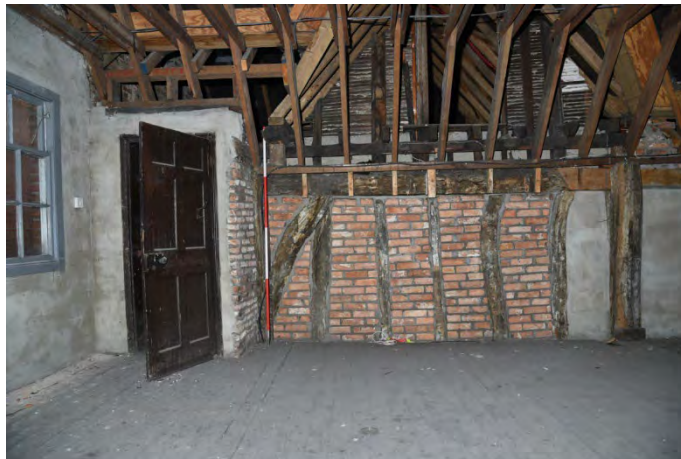
YCY044 Interior second floor looking southeast showing brace, wall plate, studs and posts E (left) and D (right) (2m scale)
