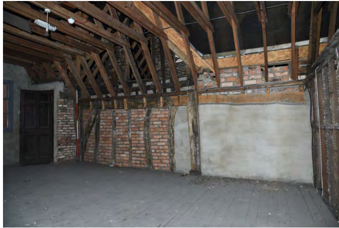
YCY045 Interior second floor looking east showing brace, wall plate, studs and posts E (left) and D (right) (2m scale)
