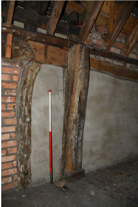
YCY047 Interior second floor looking south showing wall plate, stud and post D (1m scale)
