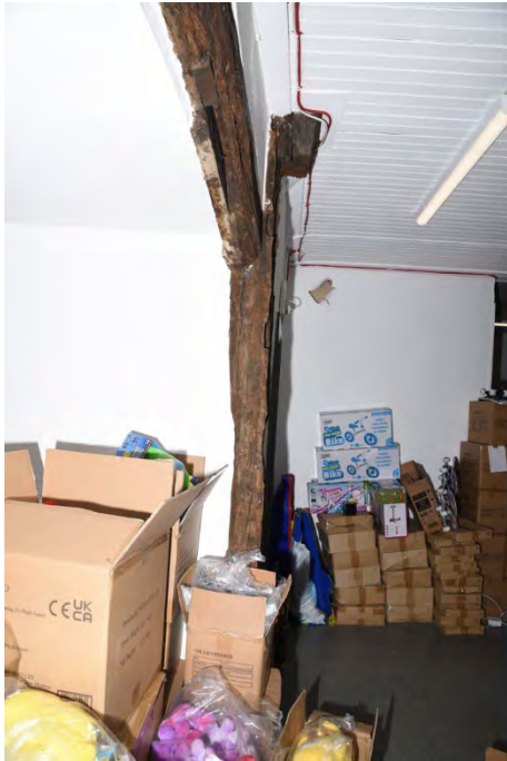
YCY019 Interior first floor looking southwest showing post A and wall plate
