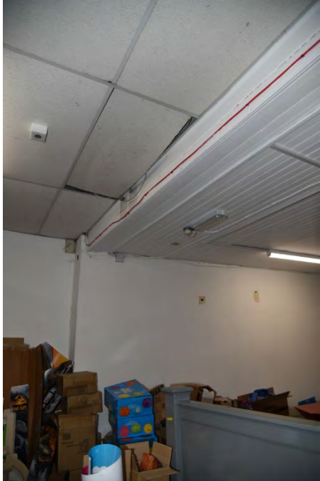
YCY023 Interior first floor looking north showing post position and boxed replacement bridging beam
