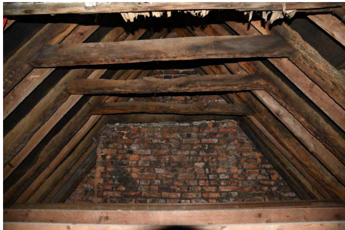
YCY050 Interior second floor looking southwest showing southwest wall and collar roof trusses
