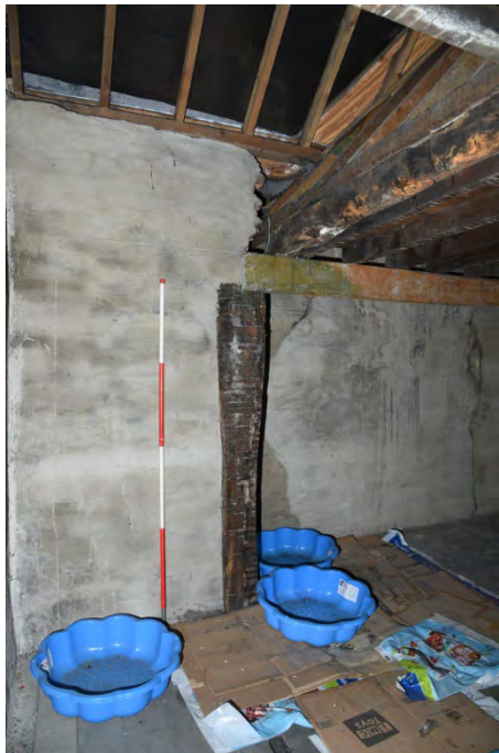
YCY033 Interior second floor looking south showing and post F (2m scale)
