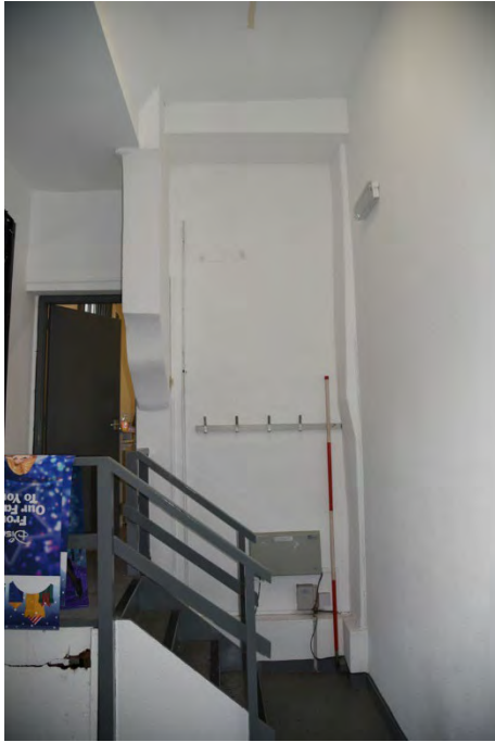
YCY027 Interior first floor looking southwest showing moulded bracket with small section of post above (2m scale)
