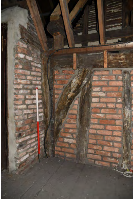
YCY046 Interior second floor looking east showing brace, wall plate, studs and posts E (1m scale)
