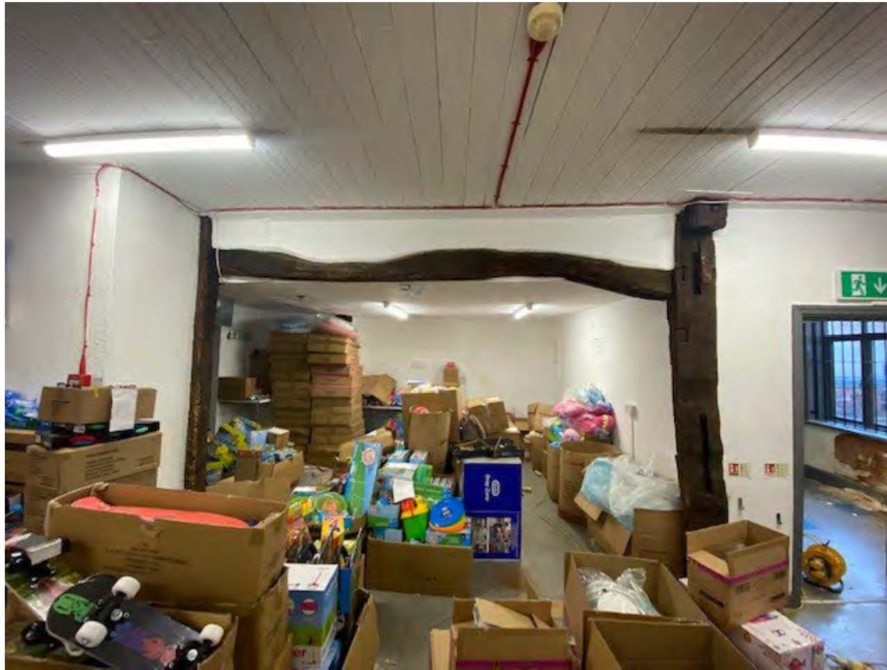
Figure 3: Posts and bridging beam at first-floor level, photograph taken from the north
