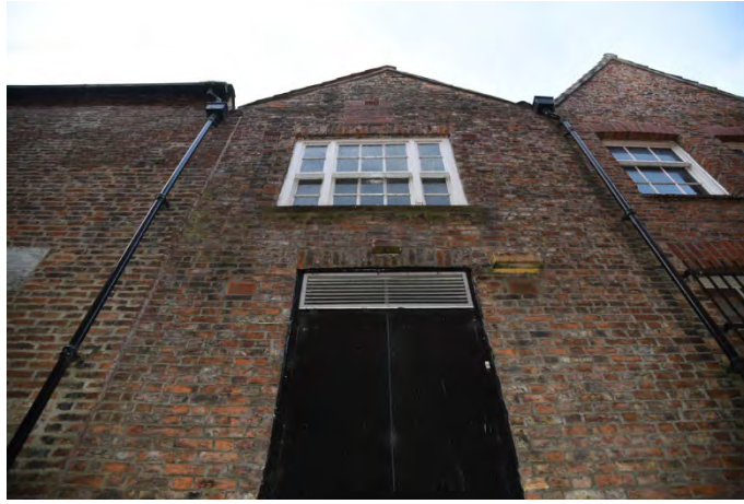
YCY008 Upper part of northeast elevation with taking in door at first floor level
