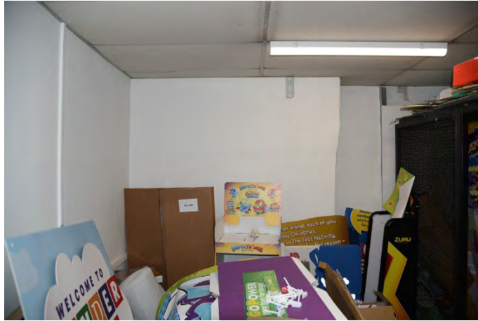
YCY024 Interior first floor looking southwest showing stack position and end wall
