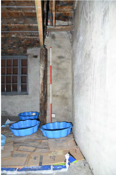
YCY035 Interior second floor looking northeast showing and post F (2m scale)
