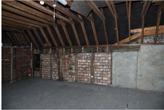
YCY040 Interior second floor looking west showing brace, wall plate, studs and post G (2m scale)
