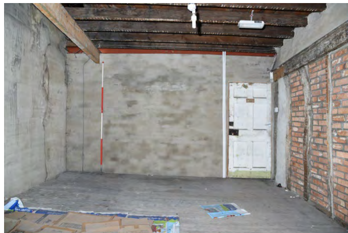
YCY030 Interior second floor looking southwest showing wall plate and studs (right) (2m scale)
