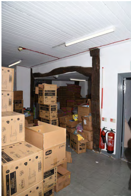
YCY015 Interior first floor looking east showing posts A and B and wall plate (2m scale)
