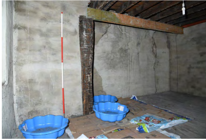
YCY034 Interior second floor looking south showing and post F (2m scale)
