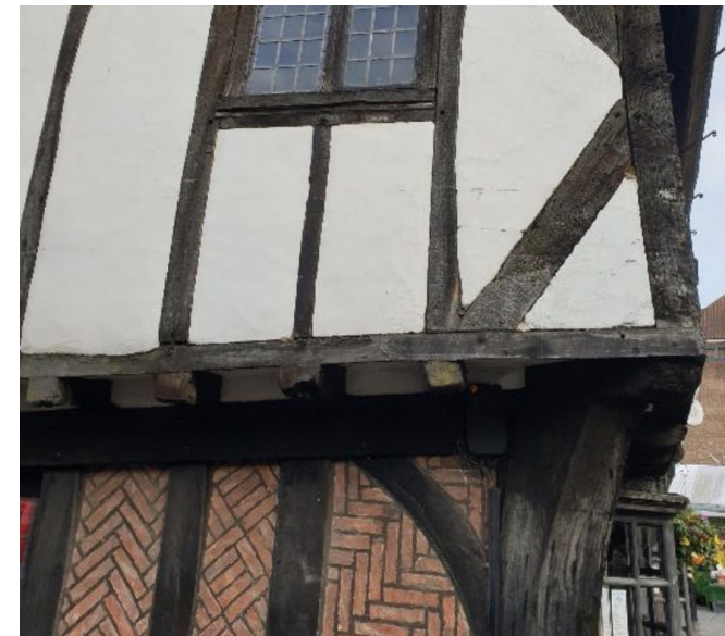
Figure 25 The present roof covering (& possibly later infill panel material) has overloaded the historic jetties, causing ongoing strain to the supporting joists.
