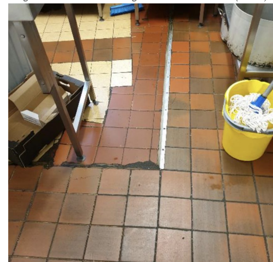
Figure 30 Poor quality floor tiles on concrete slab in the c.1960 kitchen.
