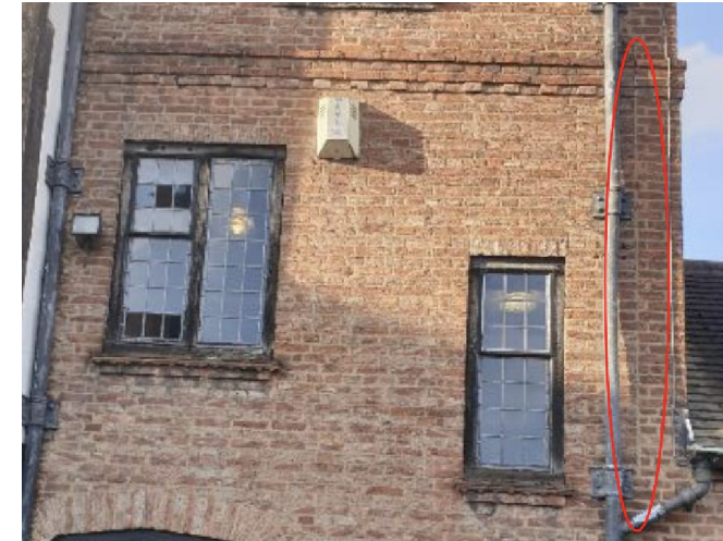
Figure 22 Building break to corner of Wall 2 (red ellipse) requiring brick anchors.
