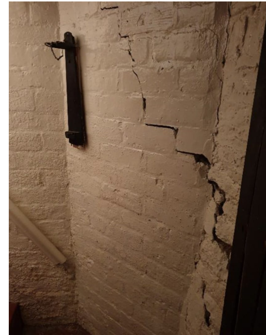
Figure 29 Structural cracking to wall cellar staircase (stair 3).
