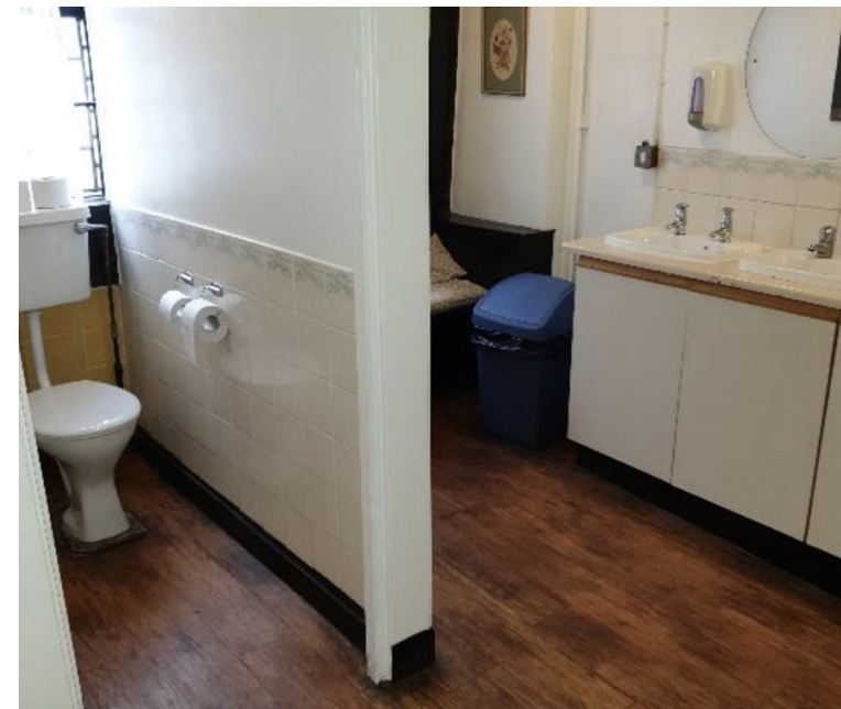
Figure 28 Poor quality later C20th plumbing in the ladies lavatory.
