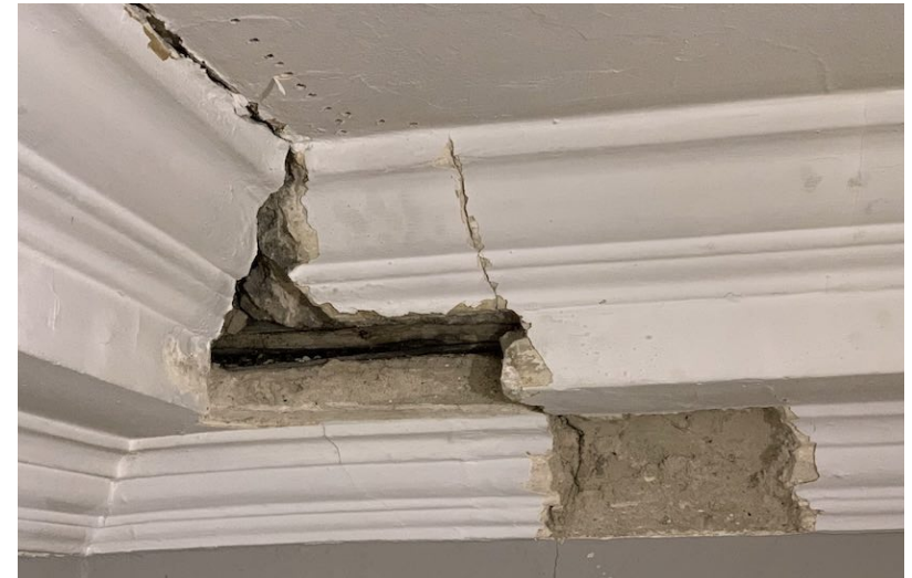
REPAIRS Example of plasterwork repairs to the North Anteroom cornice and ceiling in the Assembly Rooms. Damage has been raked out ready to hand run new lime hair plaster.
