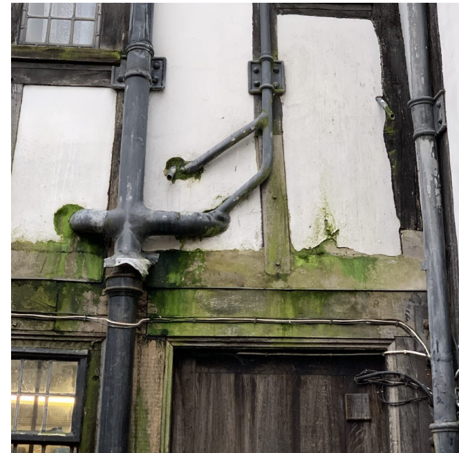
Figure 23 Detail of poor quality repairs and ongoing waterlogging damage to Wall 13 caused by the wall's 5 degree lean. Note also the blocked D3 and quantity of pipework across this wall (see I.13).
