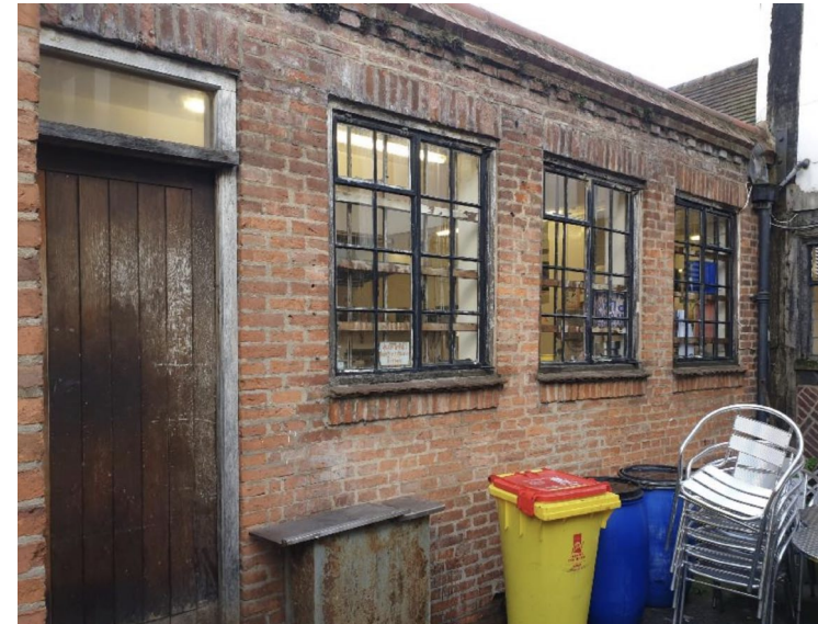
Figure 24 Kitchen viewed from the courtyard - note the salt staining around the lintels, indicative of waterlogging from roof runoff. It is further proposed to raise the height of these walls by ~450mm, retraining the existing corbelled parapet (1.05).
