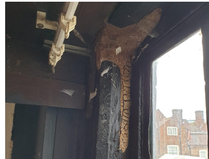
Figure 27 Example of oak rot to a window frame.
