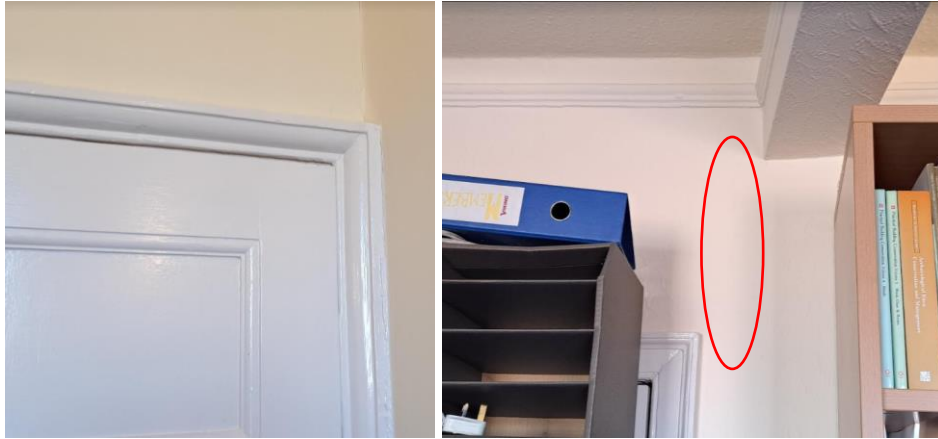
Fig 28 FF wall built up to architrave Fig 29 Gap between sf wall & architrave above
