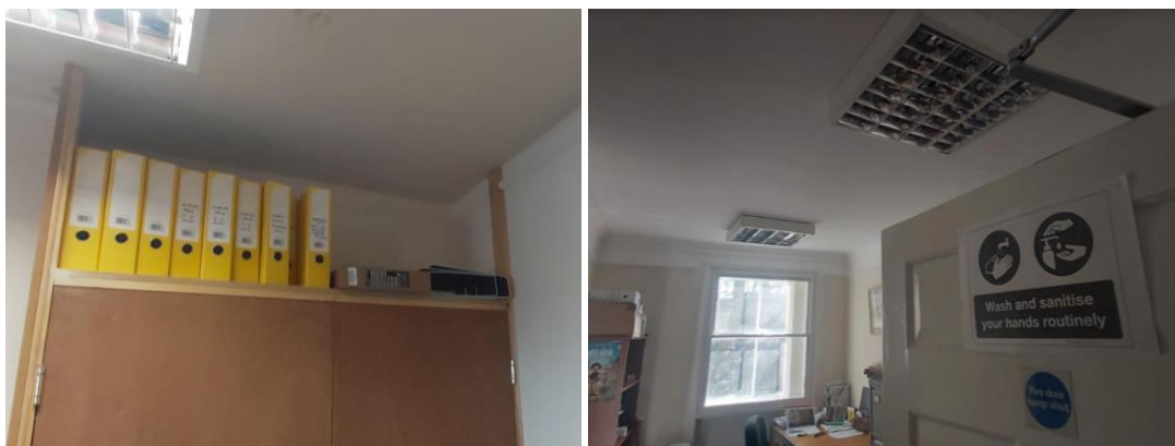
Figs 59 & 60 Commercial fittings, lights, signage & furniture to be removed
