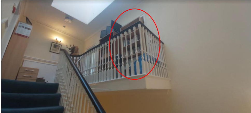
Fig 71 Functioning but blocked doorway to be reinstated
