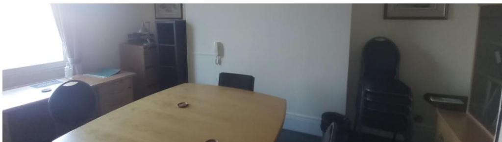
Fig 70 Missing fireplace to first floor, rear room to be reinstated
