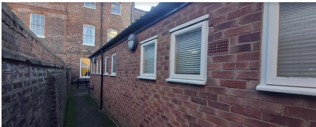
Fig 78 Unattractive rear extension to be rendered and windows and lights replaced
