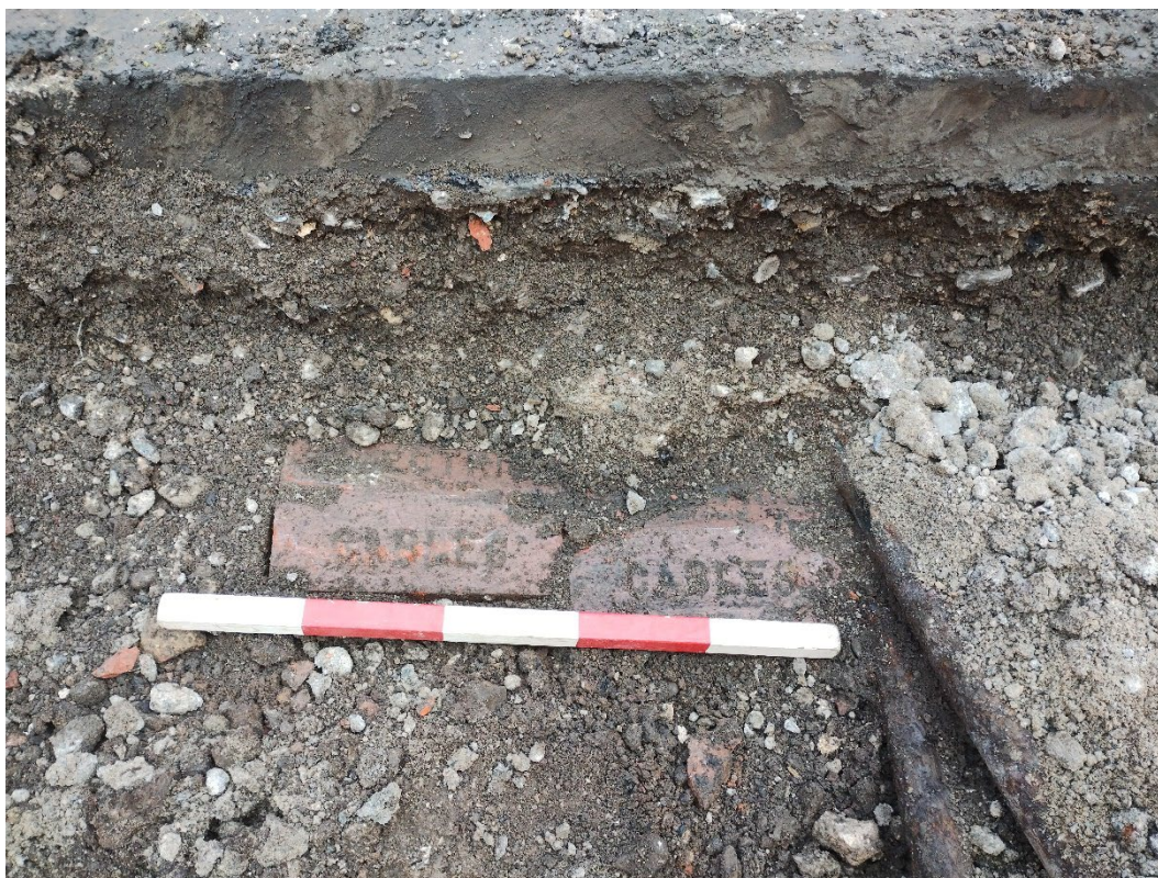
Plate 3: Ceramic Tiles covering Electric Cable
