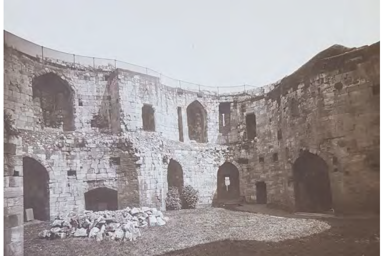
Plate 81 View of the east lobe interior dated 1913 showing late repair to first-floor window opening
