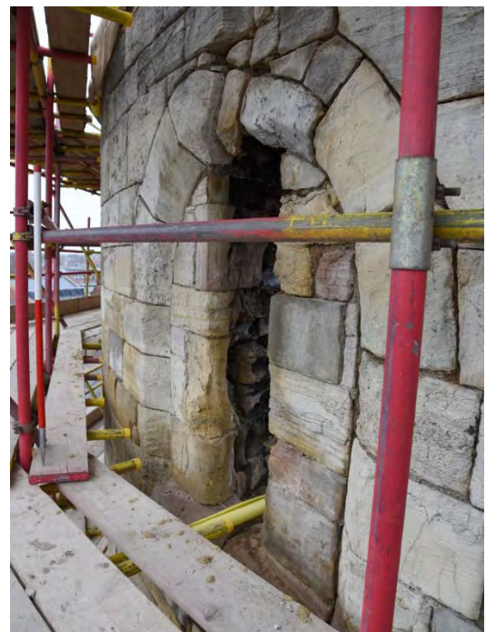
Plate 60 Upper part of partially blocked window, first floor, south lobe (Scale 0.5m)
