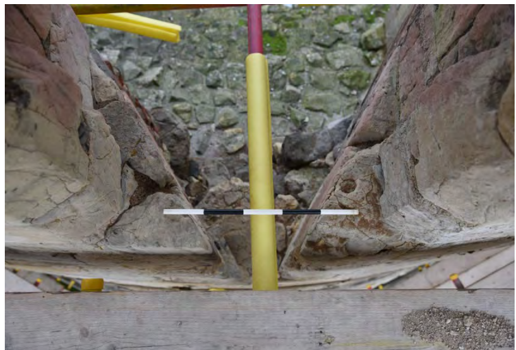
Plate 64 Sill detail of the upper part of first floor window on the west lobe (Scale 0.5m)
