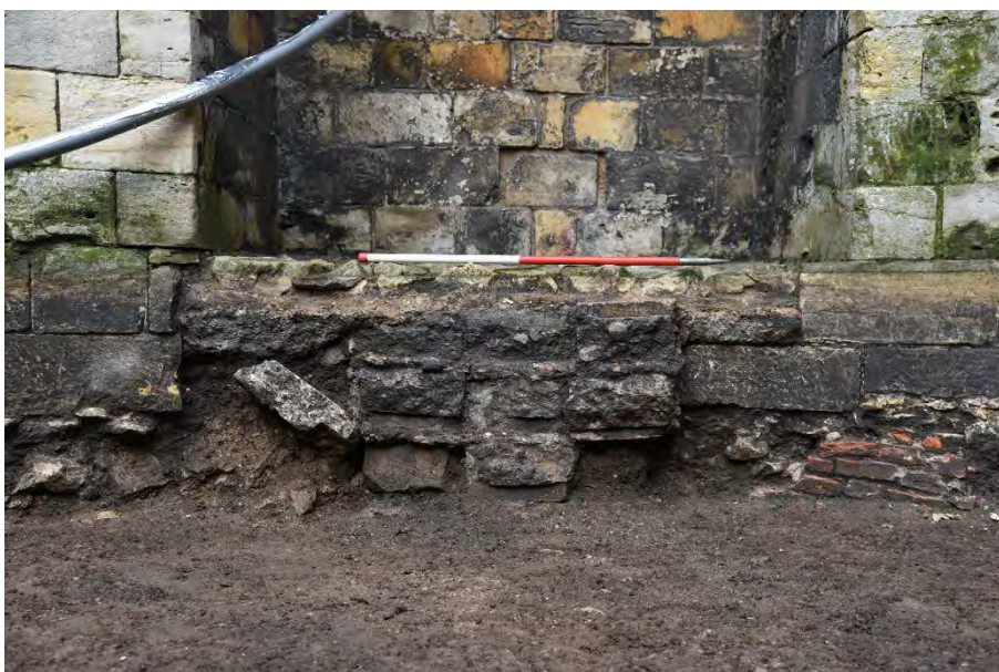
Plate 30 Concrete blocks in the north lobe west embrasure, corresponding with F62 (Scale 1.0m)
