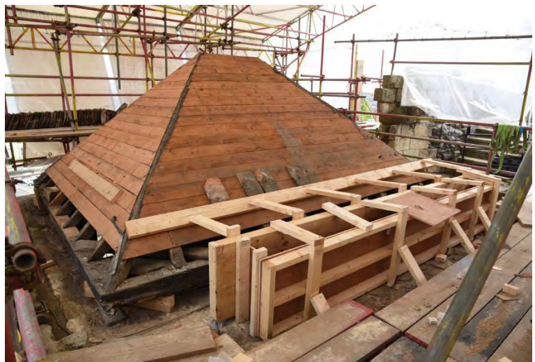
Plate 55 The roof structure on the forebuilding in the process of being re-covered
