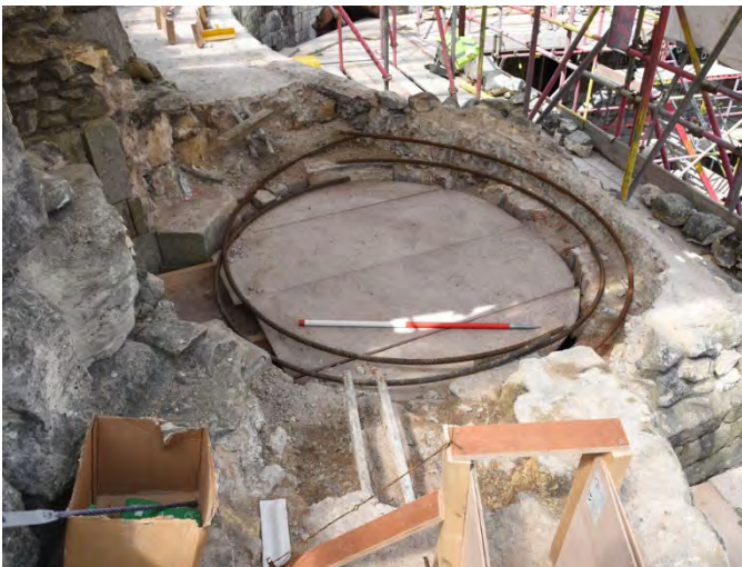
Plate 89 Upper part of bartizan stair during removal of early 20th century concrete and ironwork (Scale 1.0m)
