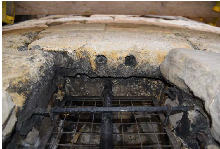
Plate 59 Ground-floor opening on the south lobe showing fixings for ironwork in the top of the enlarged opening
