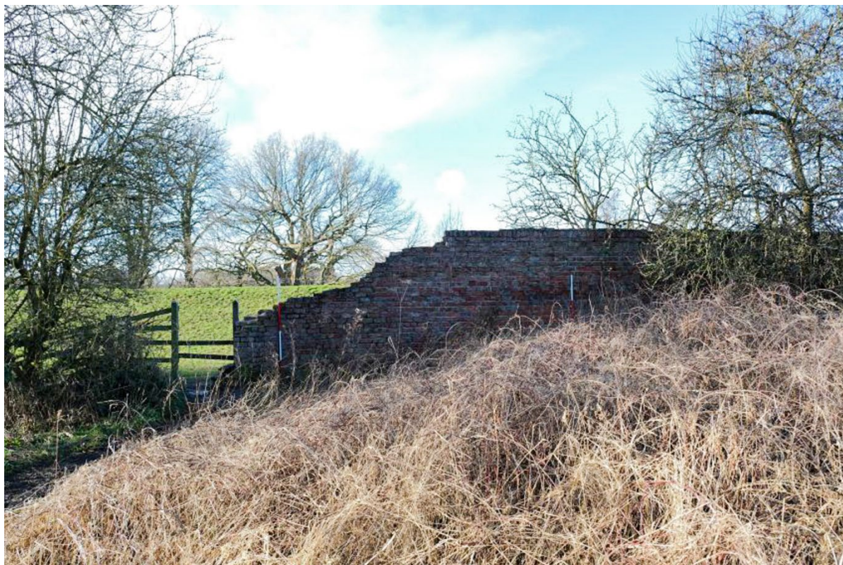
Plate 32: The partially collapsed south-eastern end of wall B, facing south-west, scale unit 0.5m.
