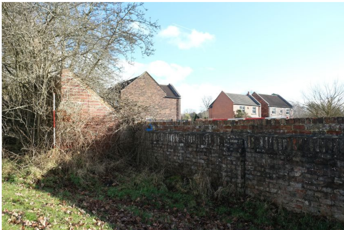
Plate 20: The higher walling at the northern end of the north-eastern elevation of Wall A, facing north-east, scale unit 0.5m.
