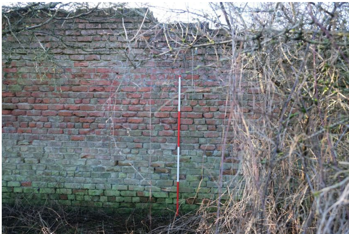
Plate 33: The partially collapsed upper portion wall B, facing north-east, scale unit 0.5m.
