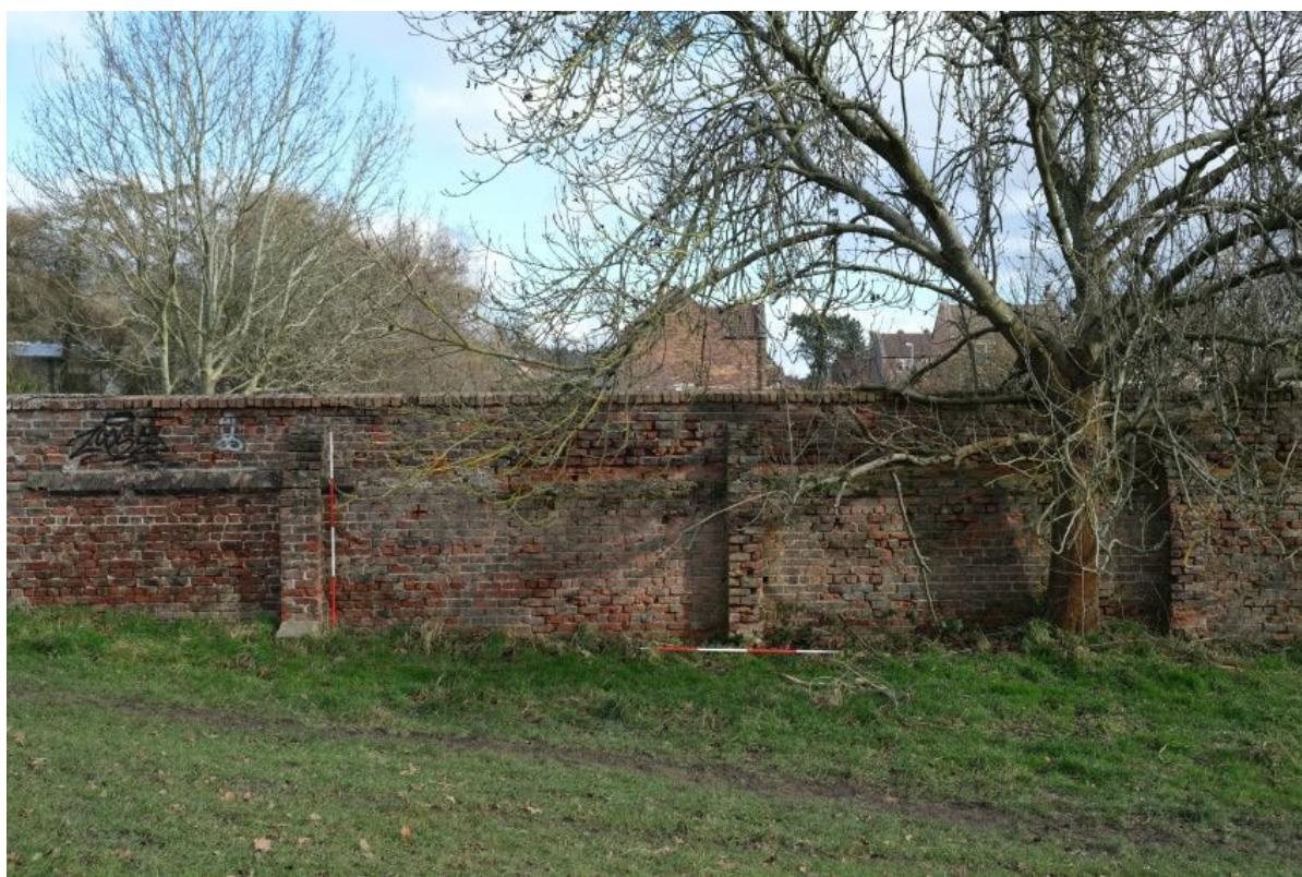
Plate 37: The north-western end of the south-western elevation of Wall B, facing north-east, scale unit 0.5m.
