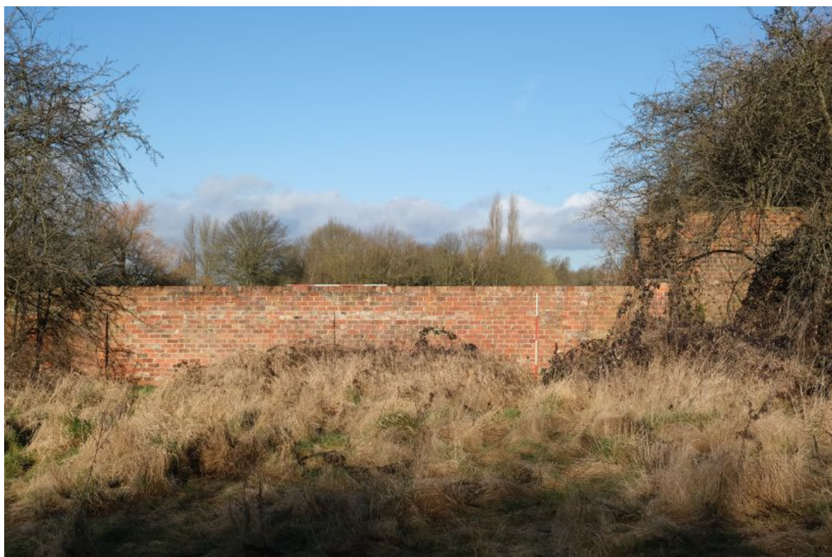
Plate 27: The north-eastern end of the south-eastern elevation of wall A, facing north-west, scale unit 0.5m.
