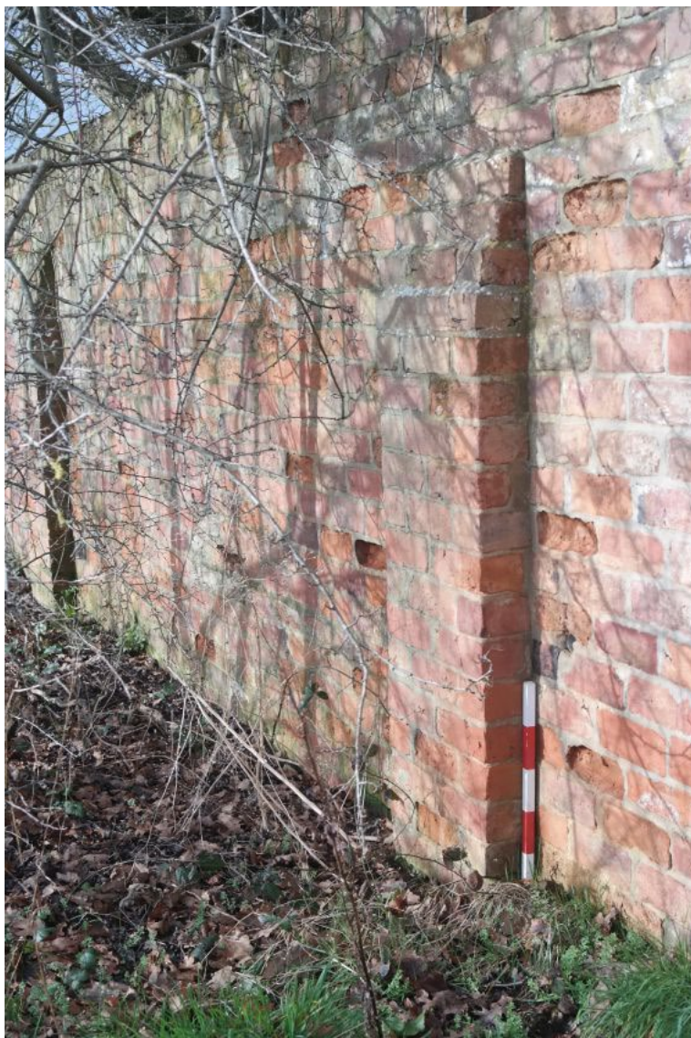
Plate 31: A buttress on the south-eastern elevation of wall A, facing south-west, scale unit 0.1m.
