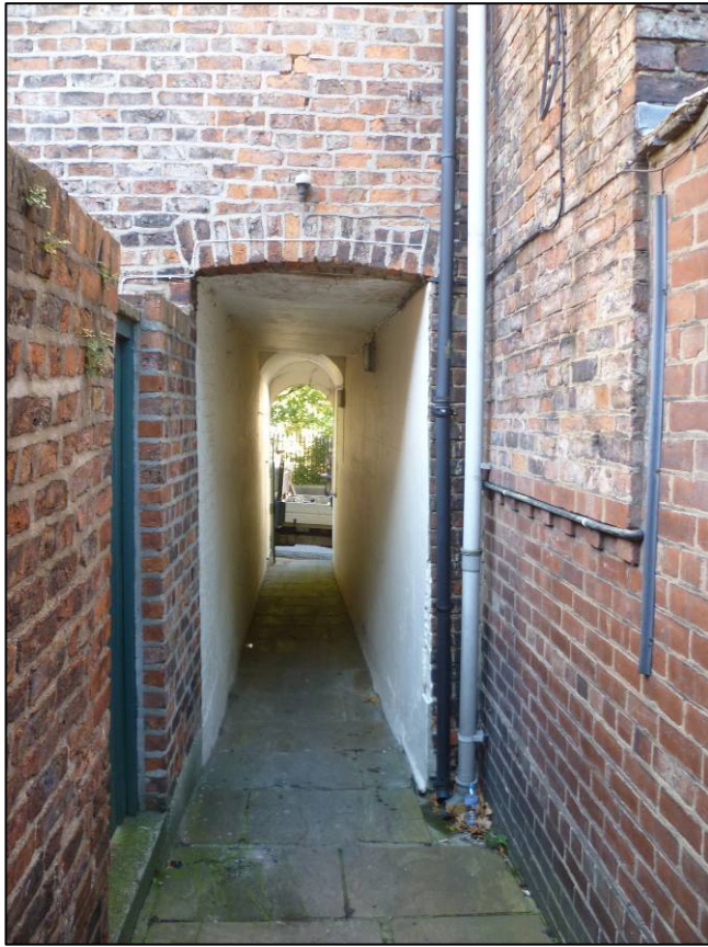
Plate 4: Pedestrian access showing external west wall of passage GF3, looking NW (photo 1/991).
