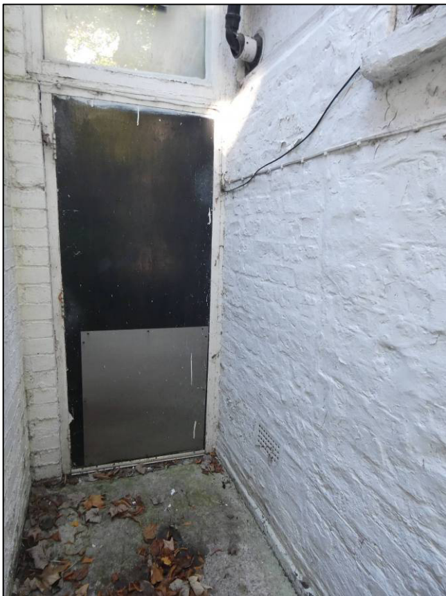
Plate 6: Exit from internal passage GF3, showing west elevation of room GF5, looking NW (photo 1/826).
