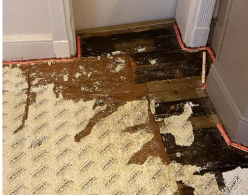
Figure 11 Chipboard and pine boards beneath carpet on first floor
