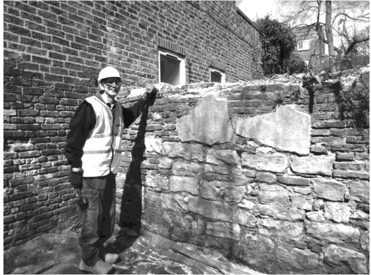
Figure 1 A member of the FCAP excavation team works on the careful demolition of the garden wall.
