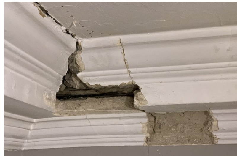
REPAIRS Example of plasterwork repairs to the North Anteroom cornice and ceiling in the Assembly Rooms. Damage has been raked out ready to hand run new lime hair plaster.
