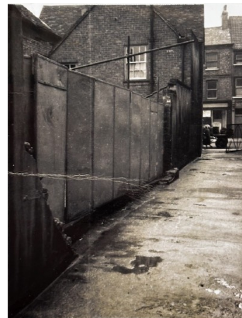
Figure 10 Photograph from June 1965 showing the side boundary wall showing the metal gate which was replaced by the existing brick wall. Photo labelled “Wall to be repaired”.
