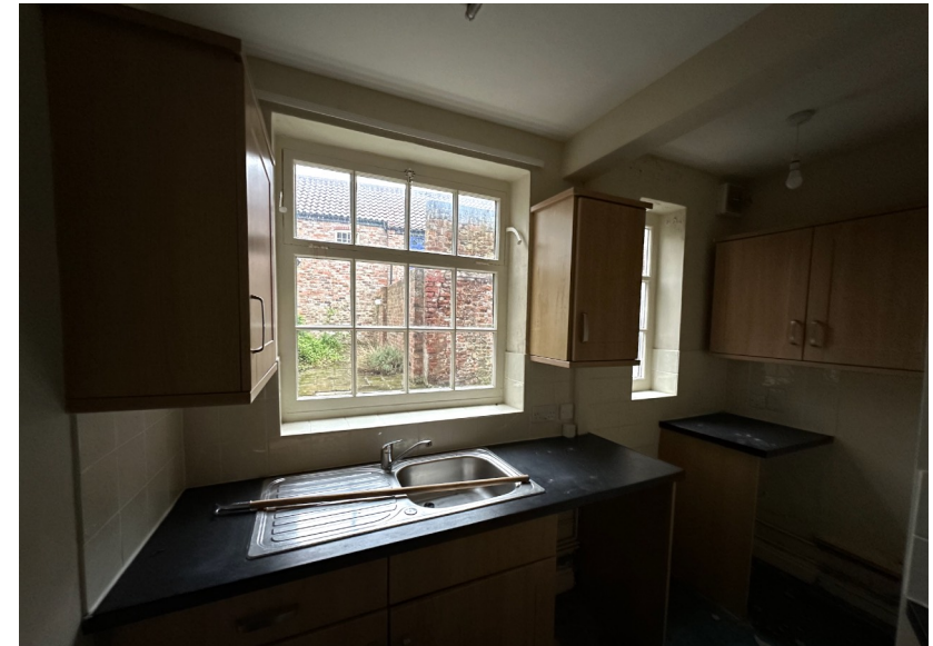
Figure 19 Present GF kitchen and 1930s windows in rear elevation proposed for removal.
