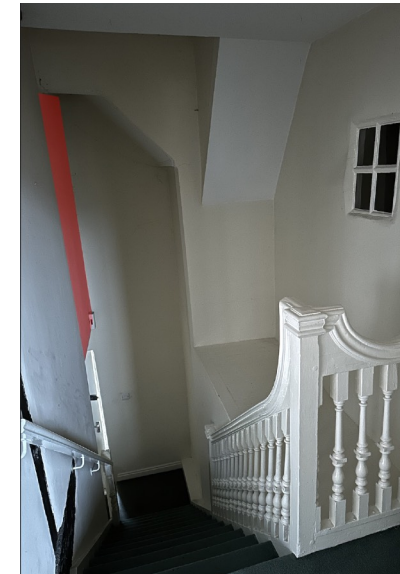
Bathroom extension over historic stairs (highlighted in red) - inserted in 1980 and proposed for removal to reinstate full height of stairwell.
