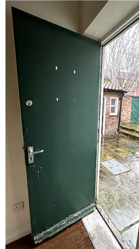
A poor-quality and inappropriate flush panel door installed in 1980.
