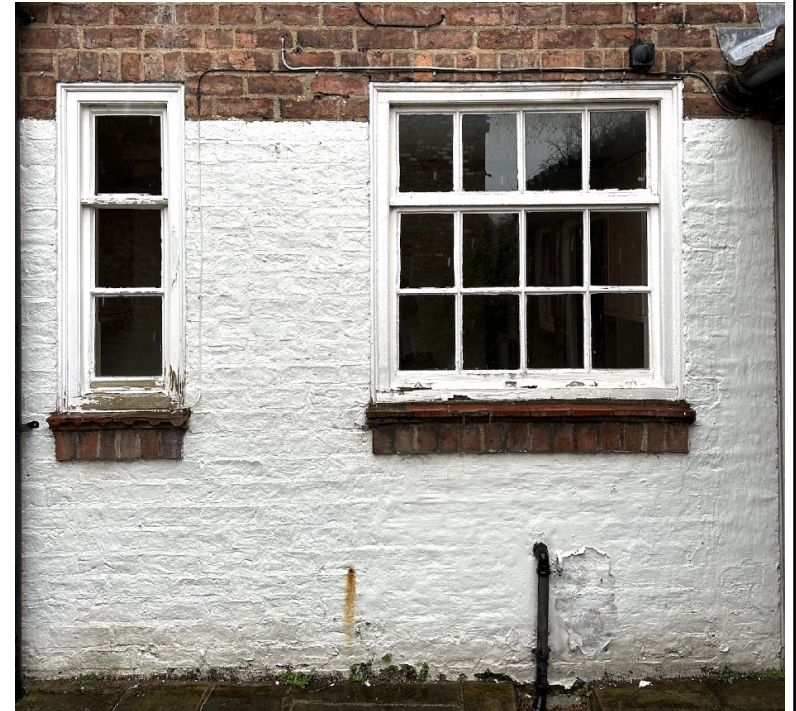
The 1935-36 rear cavity brick wall with deteriorating GF casement window.
