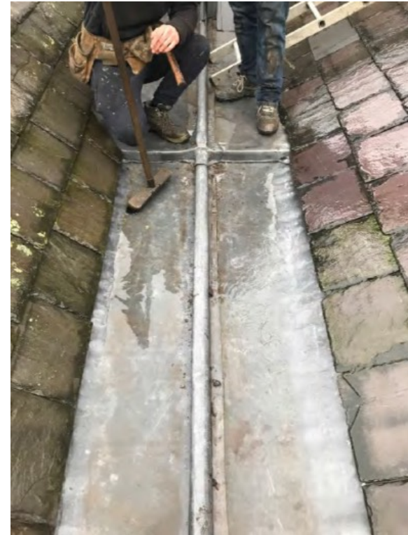
MAINTENANCE Example of valley gutter cleaning at York Theatre Royal, this needs to be undertaken on a 3-month cycle.
