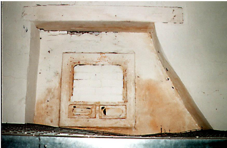
Plate 20 Engine House - Wall Box
