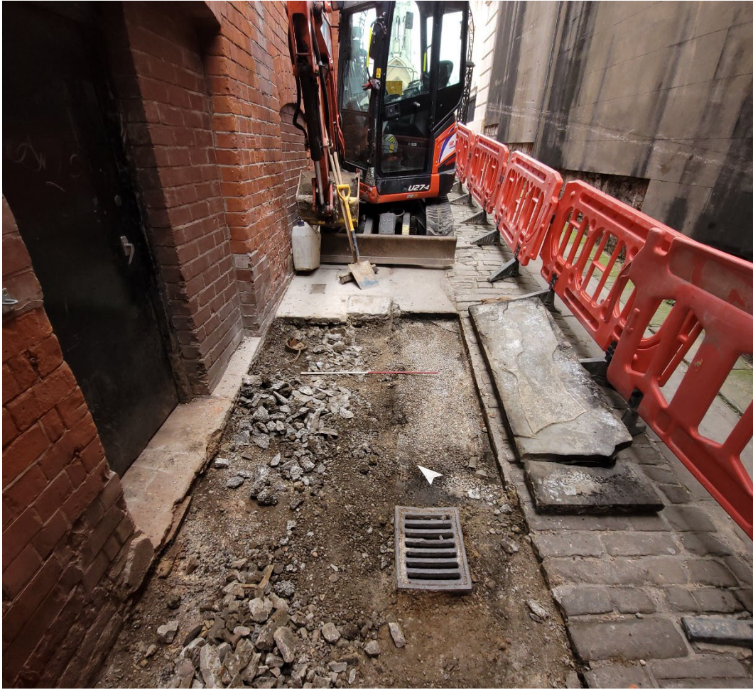
Plate 10: Trench 3 between 22 Lendal and The Mansion House, looking north-west, scale unit 0.50m
