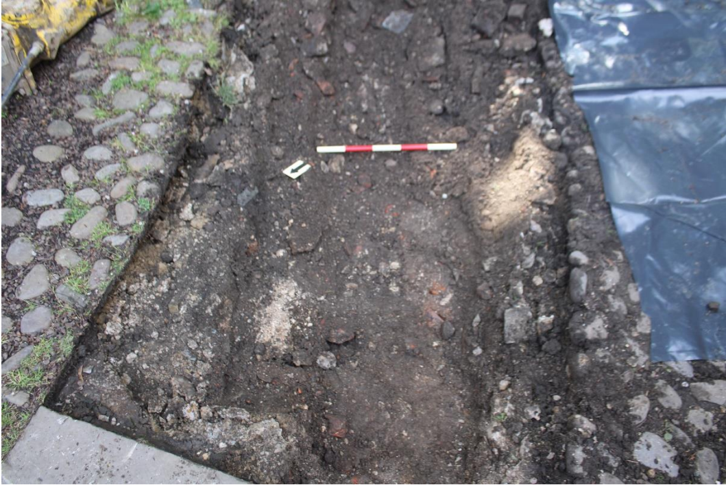
Plate 5: Backfill C1004 of electric service trench at the south end, looking south-south-east, scale unit 0.10m
