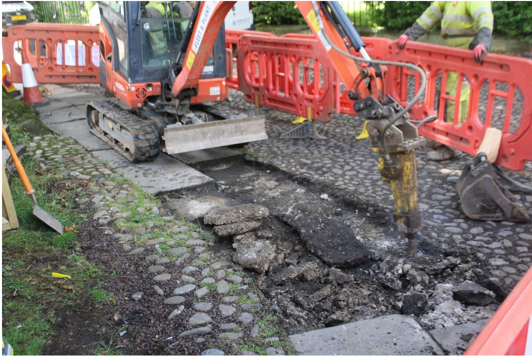
Plate 3: Removal of concrete base C1003 below cobbles C1001 and paving C1002, looking south-west
