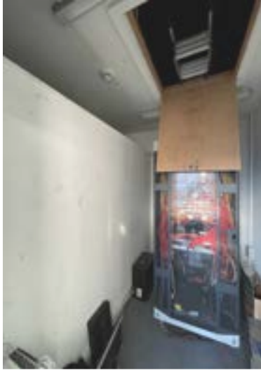
R202 IT Cupboard with access to roof
