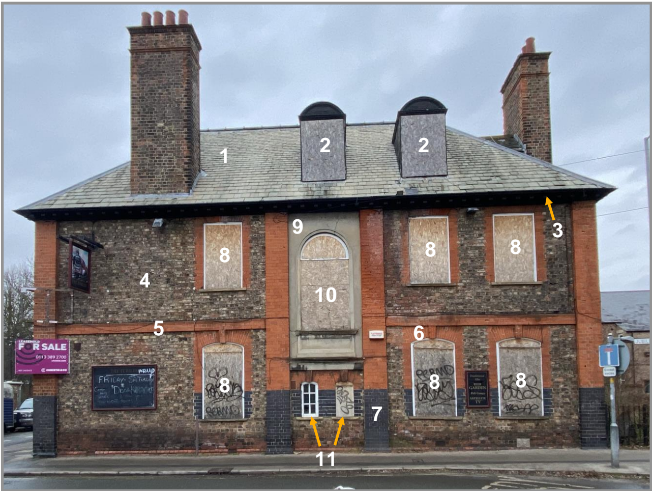
Figure 31. Salisbury Terrace elevation, 2024. Cumberland slate with rolled lead hips (1). Lead-clad dormers with 3-over-6 sash windows (2). Boarded eaves soffit with moulded modillions (3). York common brick in English bond (4). Terracotta brick sting-course with alternating English bond set-out on each façade (5). Rubbed brick voussoirs and keys (6). Black brick bases to giant order pilasters (7). 6-over-6 sash windows on stone cills (8). Stuccoed central bay with moulded window reveal, sill and panel (9). Fan-lighted stairwell window with paired sliding sashes (10). Fixed moulded casement windows on stone sills (11).
