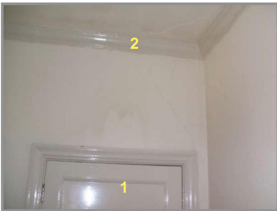
Figure 70. Doorway with lower status architrave and single upper panel (1). Intact plaster or timber coving (2). Source: Taylor (2023).
