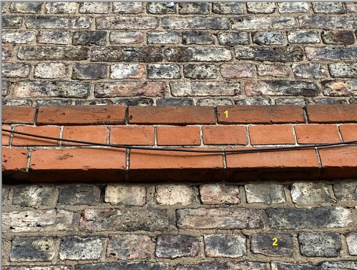
Figure 42. Salisbury Terrace elevation. Detail of red brick string course set in English bond, showing variance with the west façade. The building is constructed with lime mortar and the pointing is in generally good condition (1). Red brick stringcourse (2). York common brick set in English bond.
