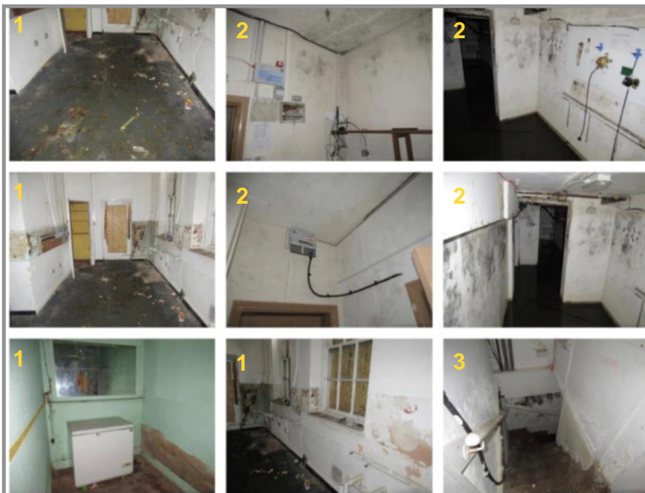
Figure 55. Service rooms have been stripped of fittings and services. It is unlikely that they would have had elaborate or bespoke fittings designed by Brierley. Kitchen (1), basement keg cellar (2), stairs to cellars (3). The keg cellar is sited directly below the original ground floor bar. Keg pipes can still be seen in the top-middle image. Source: Taylor (2023).
