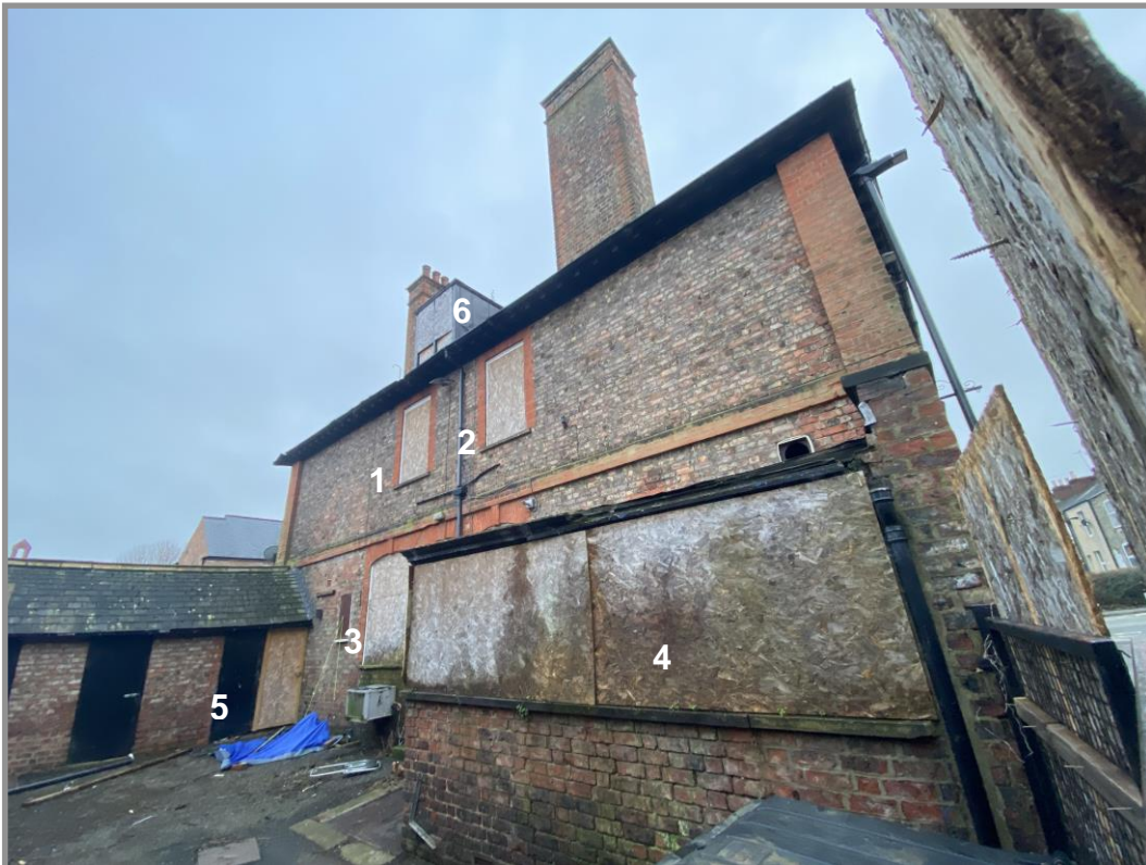
Figure 37. This north facing elevation follows the general pattern of the two principal elevations but without pilasters to the central bay. First floor level window (1) originally provided light to a bedroom, now a kitchen and window (2), lights the large functions room. On the ground floor, windows provide light to the men's WC (3). A door in the north service range leads to the kitchen and side garden. Leading from a door onto Balfour Street, a lean-to building (4) was constructed with brick lower walls and glazed timber upper section. The original function of this room is unclear. The kitchen and the garden are accessed via the ground floor service yard range via a door in the south bay (5). A dormer lighting an attic bedroom appears to be slightly smaller than those on the Salisbury Terrace elevation and early photographs indicate that its fenestration may have been different to the other dormers.
