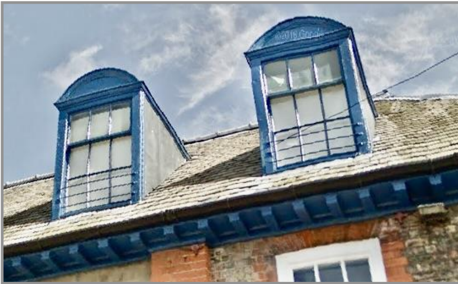
Figure 27. Detail of roof showing fine detailing to Salisbury Terrace elevation dormers and soffit with modillions. Safety bars have been fitted to the dormer lower frames. Source: Google Streetview (2012 http://tinyurl.com/yewnx9mx ).
