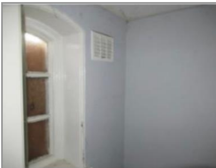
Figure 67. Detail of ground floor ladies WC showing moulded window reveal and the quality of window joinery. This window has recently been vandalised. See figure 37 Source: Taylor (2023).
