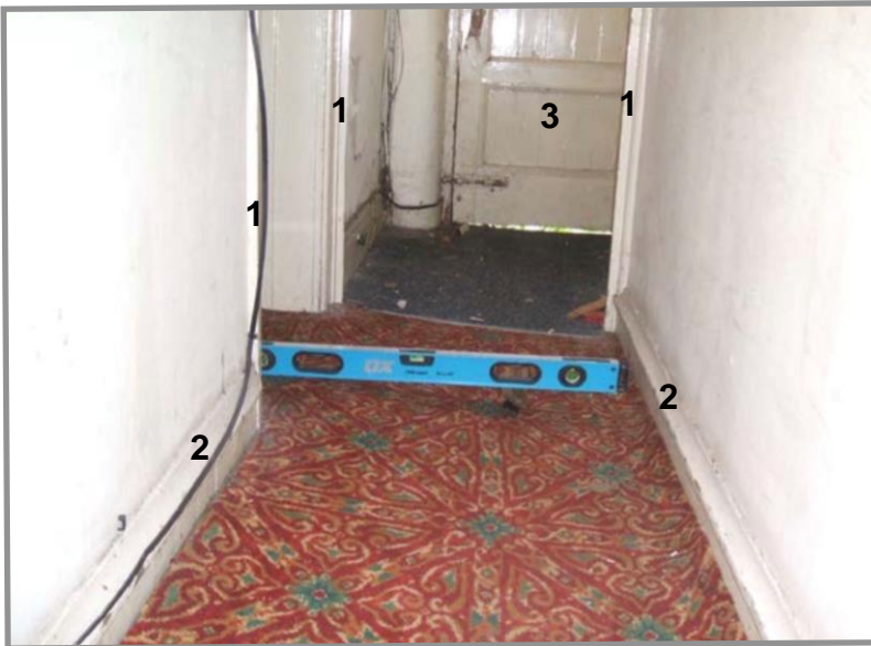
Figure 56. North elevation hall with door leading to service yard. This image shows that at the time of photographing, interior period details were still intact; moulded door architraves (1), tiled and bullnose skirtings (2) (for ease of mopping), and framed and boarded exterior door (3). Source: Taylor (2023).
