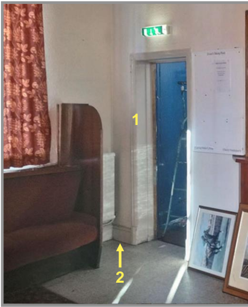
Figure 59. Northwest lounge leading off door to main entrance. Architrave (1) and moulded deep skirtings (2) are still present. Source: Taylor (2023).
