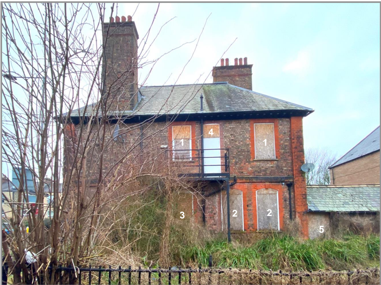
Figure 28. This east-facing elevation follows the general pattern of the two principal elevations but the black brick detail at ground-floor level is not repeated and it omits the central bay pilasters. First-floor level windows (1), relate to bedrooms and the close-set ground floor windows provide light to the kitchen (2), and to the still-room (3). A modern fire escape and door have been inserted into this elevation (4), and this leads to an enclosed garden. The garden is accessed via the ground floor service yard buildings via a door in the south bay (5).
