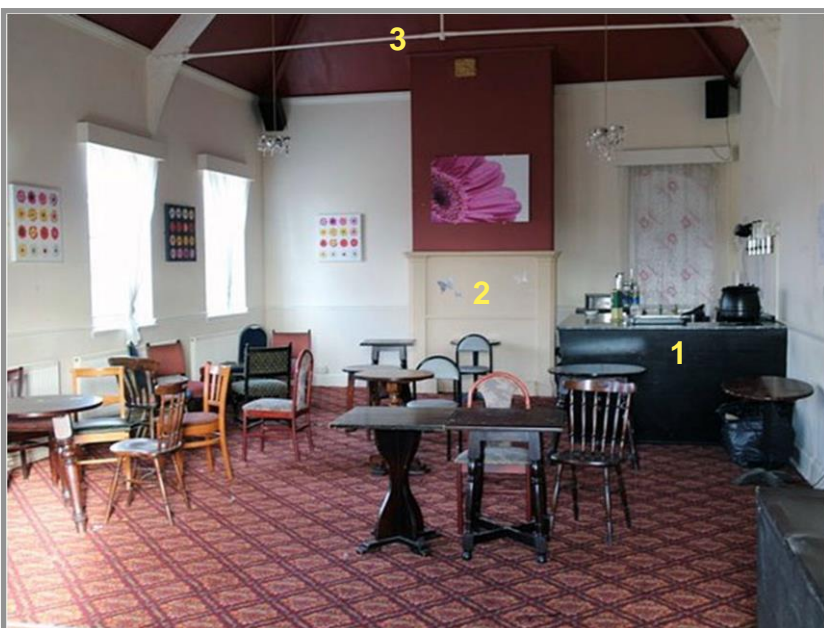
Figure 61. Games room to southeast with period fire surround and coal grate (1). Deep moulded skirting (2) appears to be intact, and the ceiling has a moulded cornice (3). Source: Taylor (2023).
