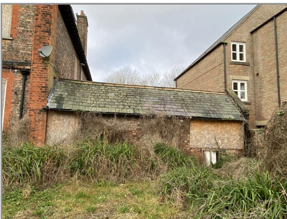
Figure 34. Rear elevation of the service range buildings showing the random width and coursed Welsh slate roof with clay ridge tiles. The windows and doors have been boarded-up, so it has not been possible to analyse these elements.
