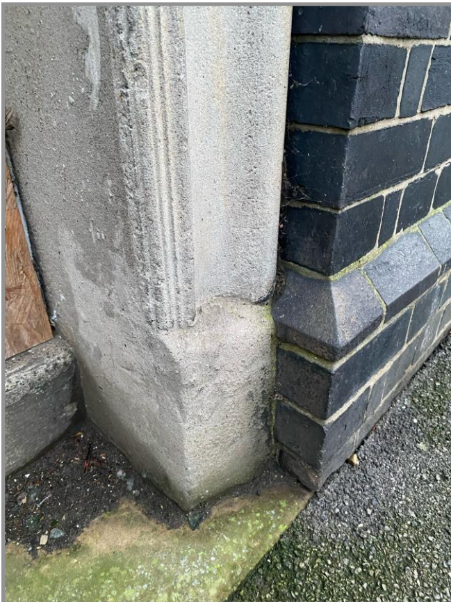
Figure 48. Moulding detail of stucco work at ground level to the main entrance door casement. Stucco, if not maintained is prone to rapid deterioration. Even at exposed ground floor level, the stucco on the Jubilee is remarkably fresh.
