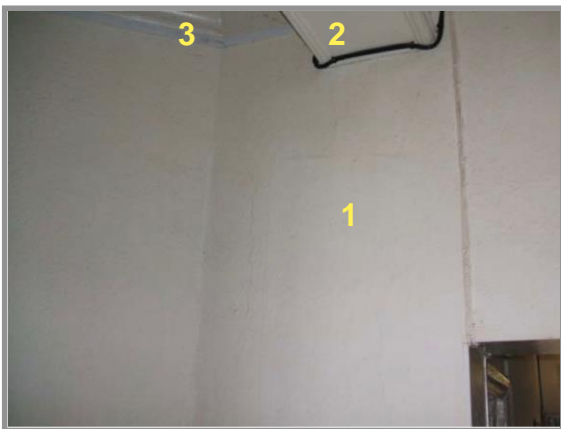
Figure 69. The interior walls are lime plastered (1). This is evidenced by the use of plastering staff beads. Generally, plasterwork appears to be in good condition despite graffiti on the upper floors and the damage caused by the strip-out of fittings in the lounges and kitchen. The large lateral beams (2), which support the function room floor above, are clad in timber with moulded details. It is possible that these beams are steel rather than timber. Decorative timber or plaster cornice (3). Source: Taylor (2023).
