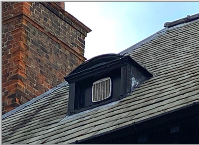
Figure 25. The Balfour Street elevation small dormers were once glazed with horizontal triple pane casements. The joinery detail to dormers is particularly fine. See Figure 5 for an earlier image.
