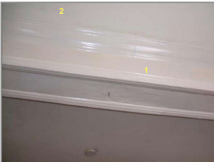
Figure 73. Main lateral lounge beam supporting the function room floor above clad in timber with moulded details, (1). It is possible that these beams are steel rather than timber. Decorative timber or plaster cornice (2). Source: Taylor (2023).
