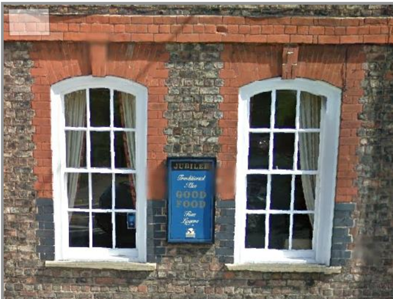
Figure 53. Ground floor windows. This design is repeated across the whole of ground floor with the exception of the small ladies' WC windows on the south elevation and the gent's WC on the north elevation. See Figure 37 above. Source: Google Street (2012, http://tinyurl.com/mcjdnmdc ).
