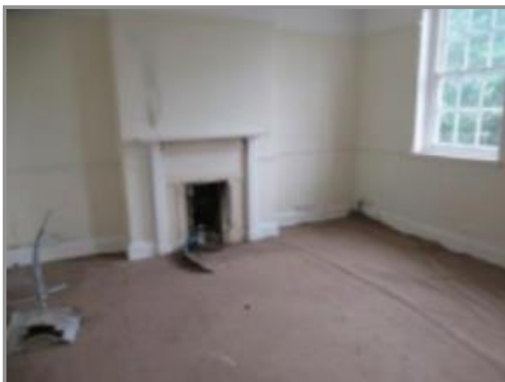
Figure 66. First floor southeast bedroom showing the survival of joinery detail; fire surround, skirting, dado rail, picture rails. Bedrooms have been carpeted, which would contribute to their preservation. Source: Taylor (2023).
