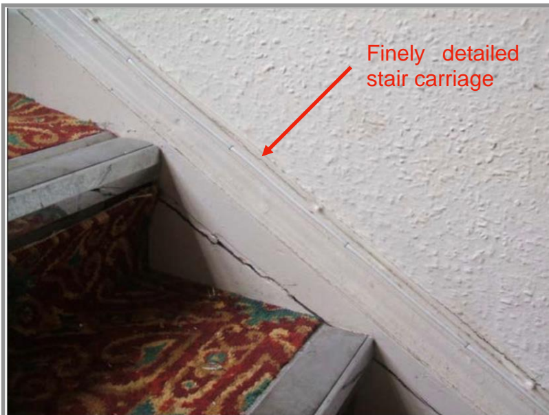
Figure 57. The staircase to the first-floor function room and bedrooms has a finely moulded closed stinger. It is most likely that the original treads and risers are in good condition, protected by the later fitted carpets. Source: Taylor (2023).
