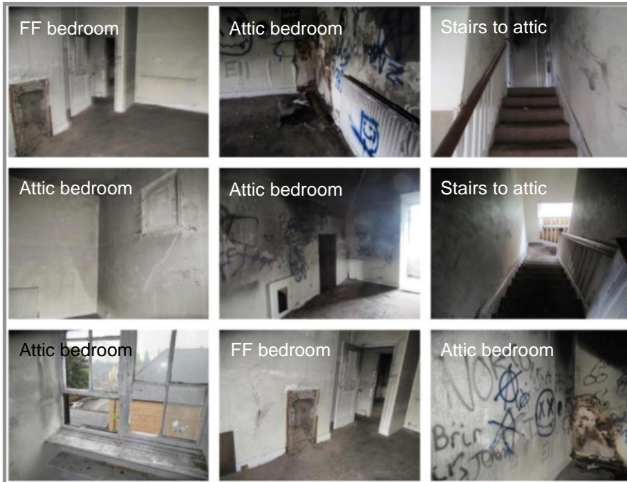
Figure 65. General views of the upper floor bedrooms. Despite the loss of some fire surrounds, the unsightly graffiti, and the damage to windows, almost all the original joinery elements are still present. Detail of simply detailed fire surrounds elsewhere in the property could be used to reconstruct losses. Source: Taylor (2023).
