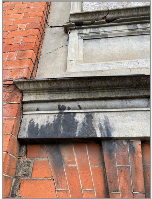
Figure 47. Detail of stucco work to the Salisbury Terrace central bay. Despite some settlement fractures, the material is in good condition after more than a century.
