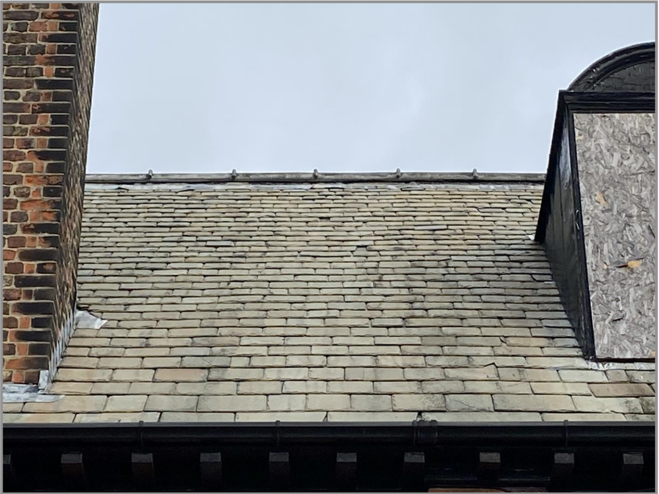
Figure 20. Detail of random width Cumbrian roof slates laid in diminishing courses and with lead hip rolls.
