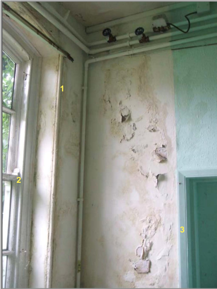
Figure 72. Kitchen window detail with door leading to Still Room. Timber plasterwork staff-bead, including the segmental-arched tops of window reveals (1). The quality of the window detail is evident. Sliding sashes are horned (2). The doorway to the Still Room has simple bevelled architraves (3). Source: Taylor (2023).
