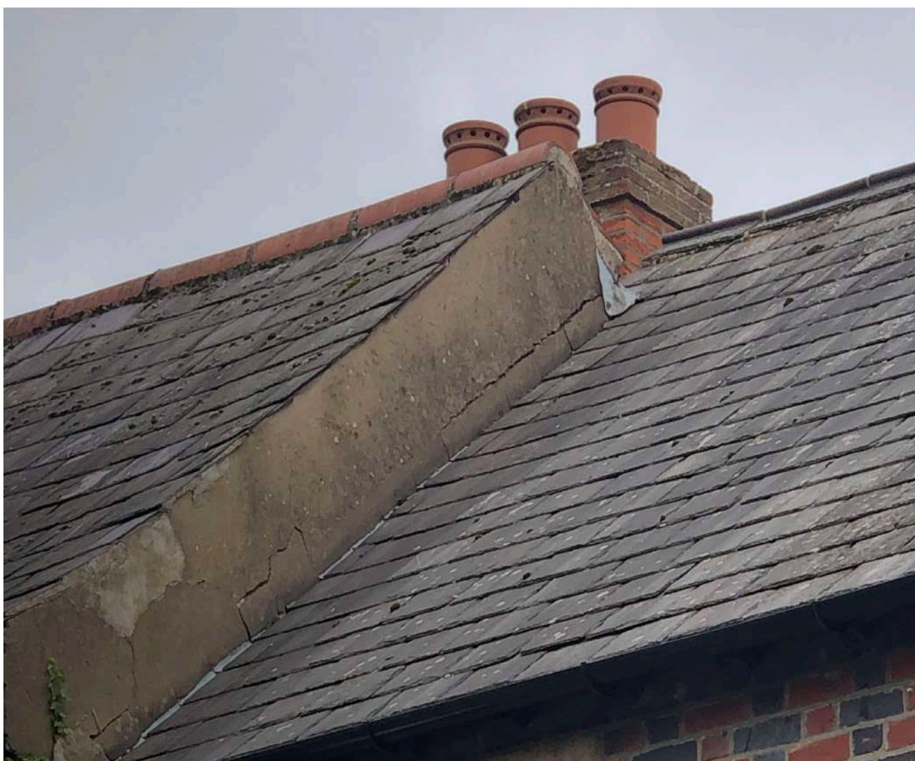
Figure 16: The cement render which joins No. 7 Minster Yard to No. 1 Deangate at present.
