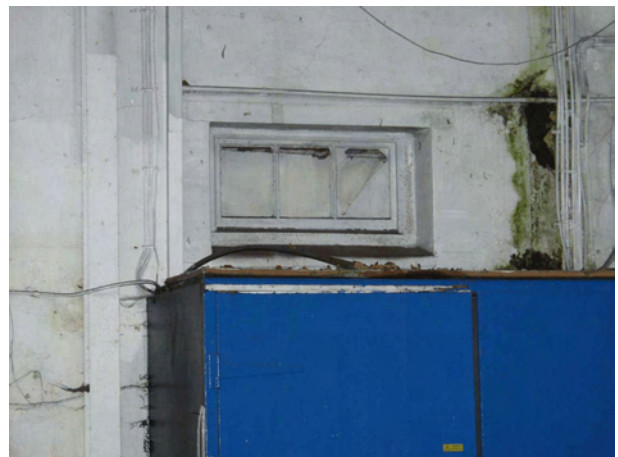
Plate 25 High level three-pane window in the southeast elevation of the central shed
