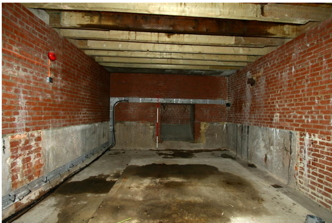
Plate 3 View of interior of the generator enclosure, looking NNE
