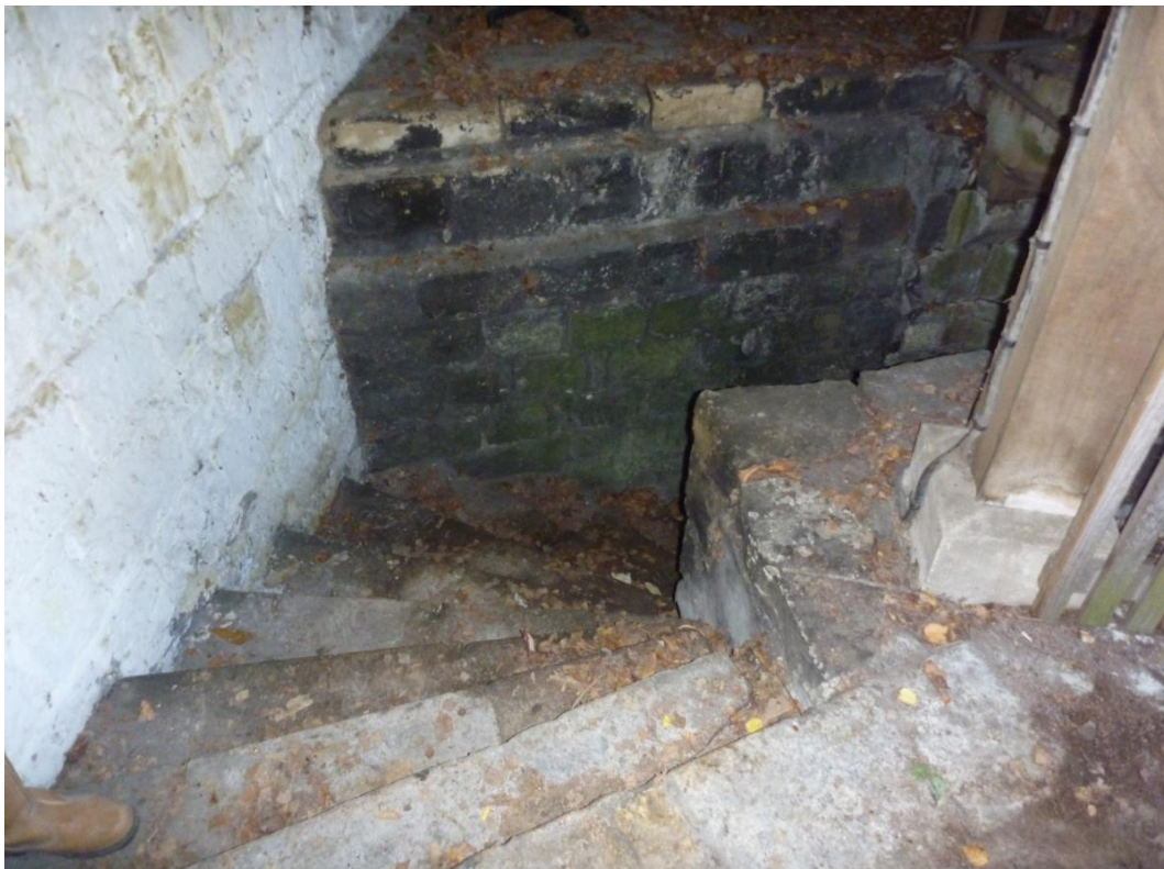
Plate 7 Steps leading to the entrance to the cellar and generator enclosure, looking S
