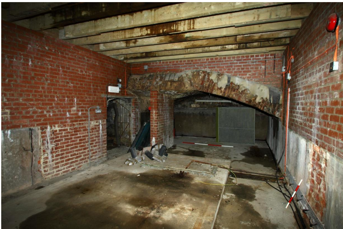
Plate 2 View of interior of the generator enclosure, with old cellar beyond and entrance to the left. Note the truncated brick arch of the cellar roof. Looking SSW
