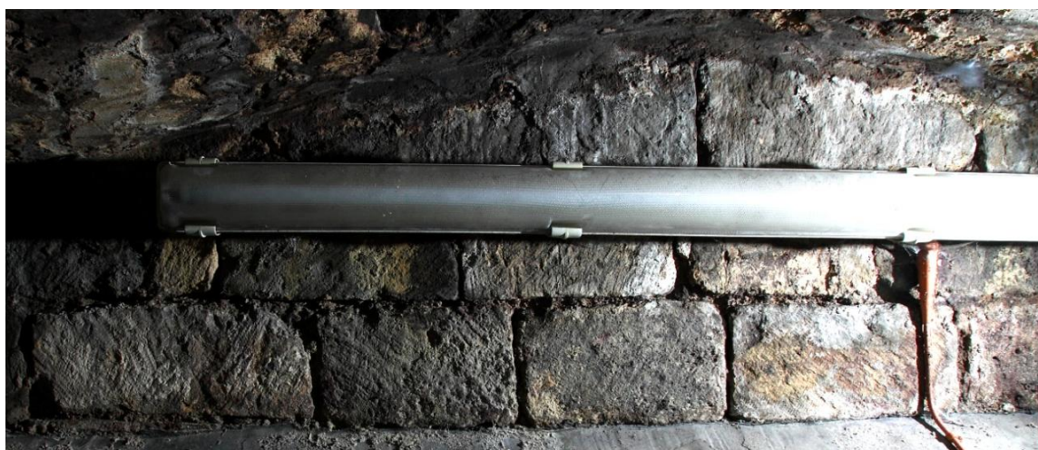
Plate 5 Claw-tooling visible in raking light to stonework of upper part of S wall of cellar. Looking SSW
