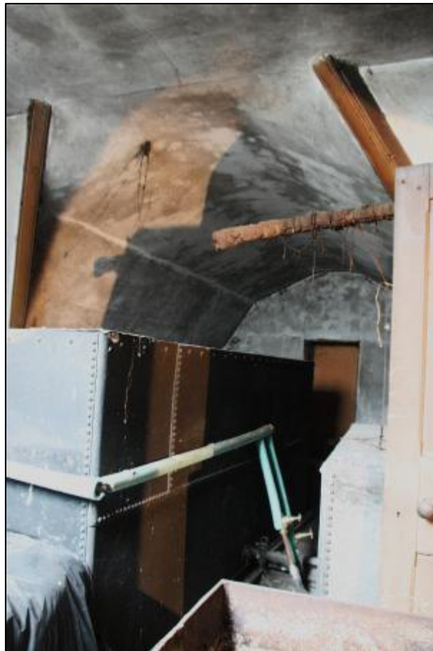
Plate 105: Room A3, looking north, noting boarded window at end of room
