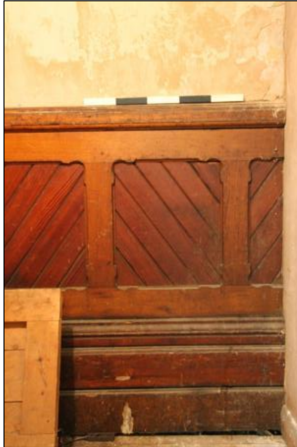
Plate 49: Detail of panelled dado in cellar head of Room G1, looking northwest
