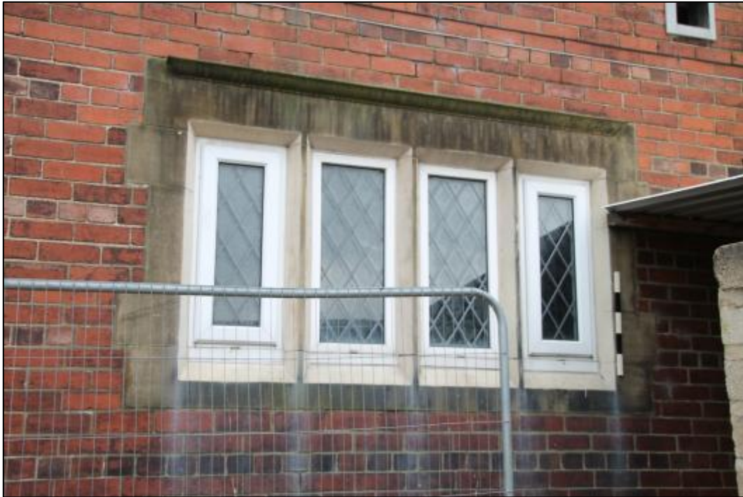
Plate 29: Detail of stone mullion window in northwest elevation of pitched roof extension
