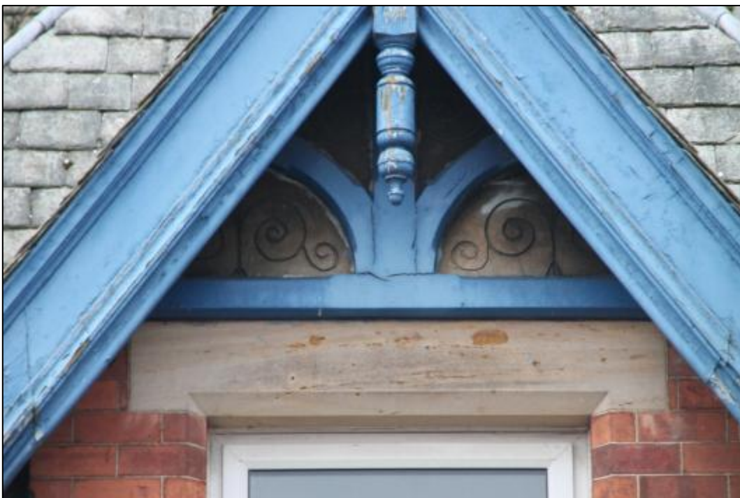
Plate 22: Detail of decorative plaster panels in gable of northeast elevation of cottage
