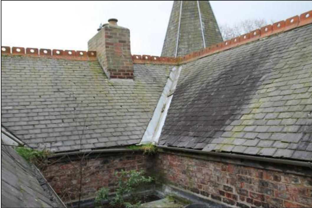
Plate 112: View of central flat roofed area from window in Room A3, looking south
