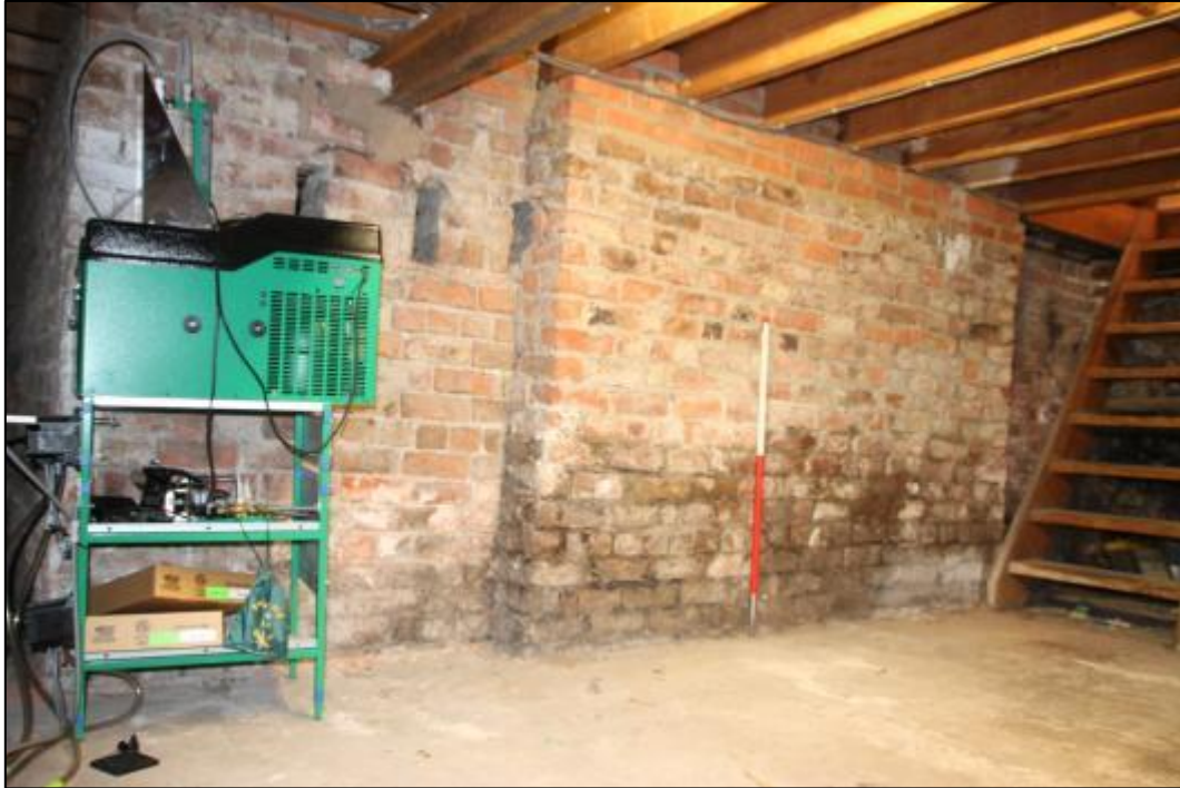
Plate 33: Room B1, looking north, noting redundant joist holes
