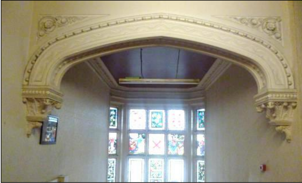
Plate 75: Detail of the arch over the stairs in Room F1, looking northeast
