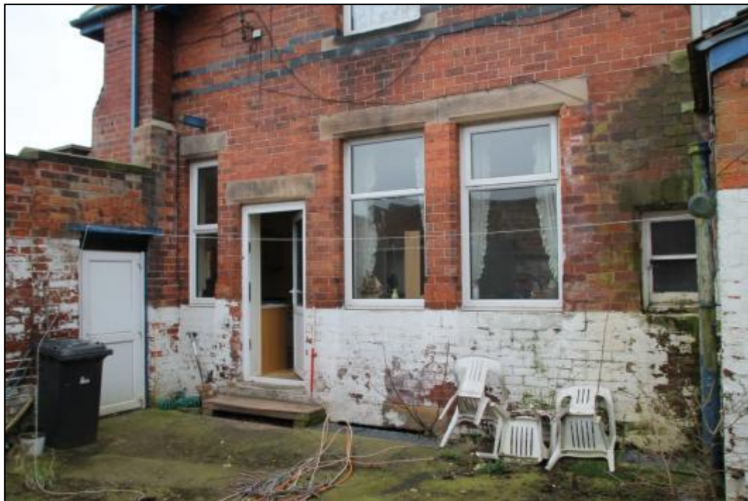
Plate 24: General view of ground floor of northeast bay of the cottage's northwest elevation looking, across the yard
