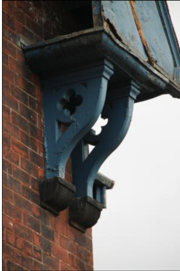
Plate 15: Detail of bracket to bargeboard of the eastern bay of the southeast elevation
