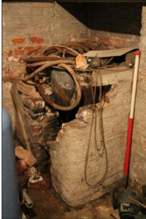
Plate 41: Water boiler in Room B13, looking east
