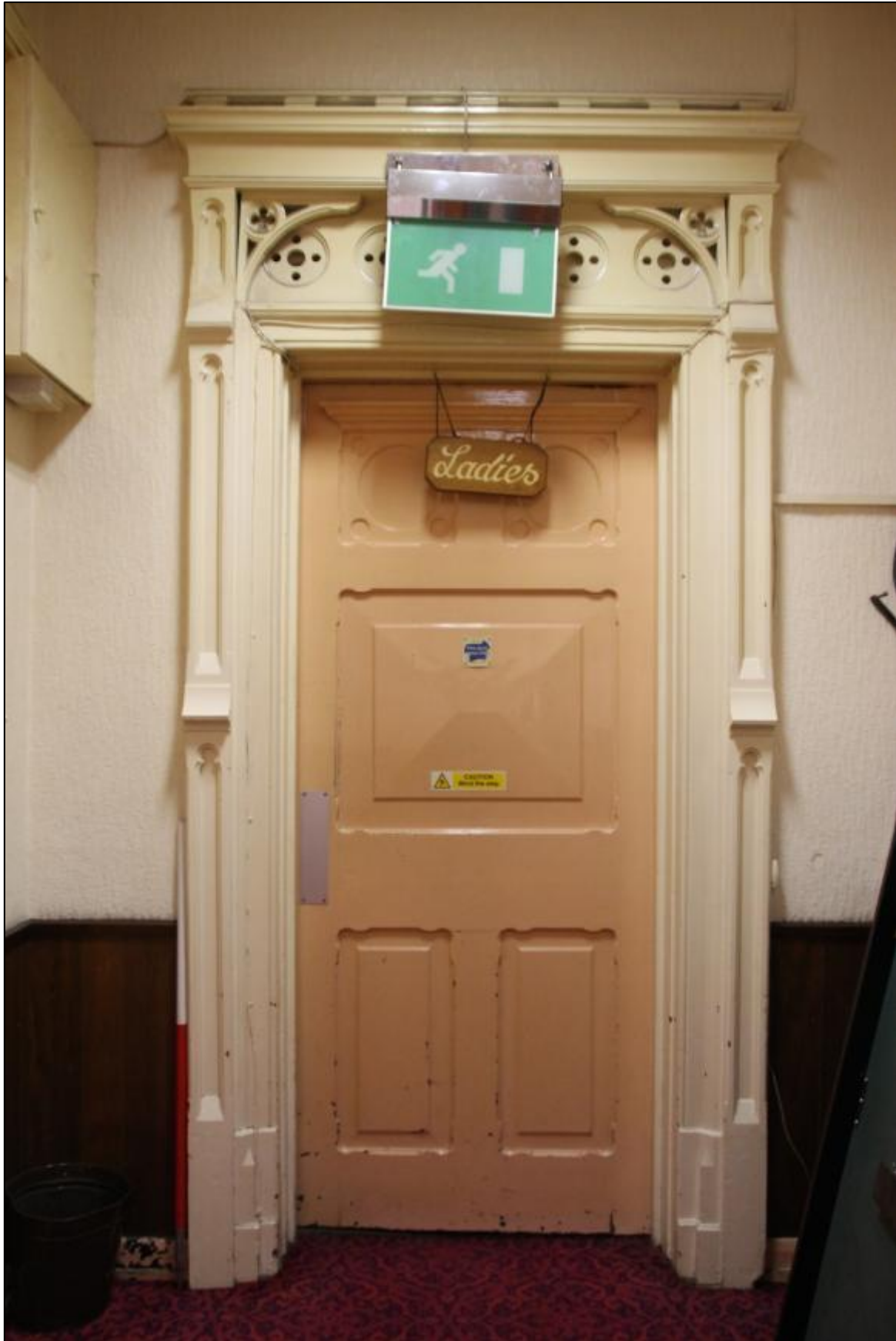
Plate 44: Detail of door through to Room G6 from Room F1, looking northwest
