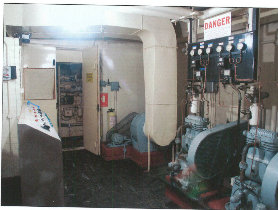
Plate 6: General view of the plant equipment room for the ventilation system
